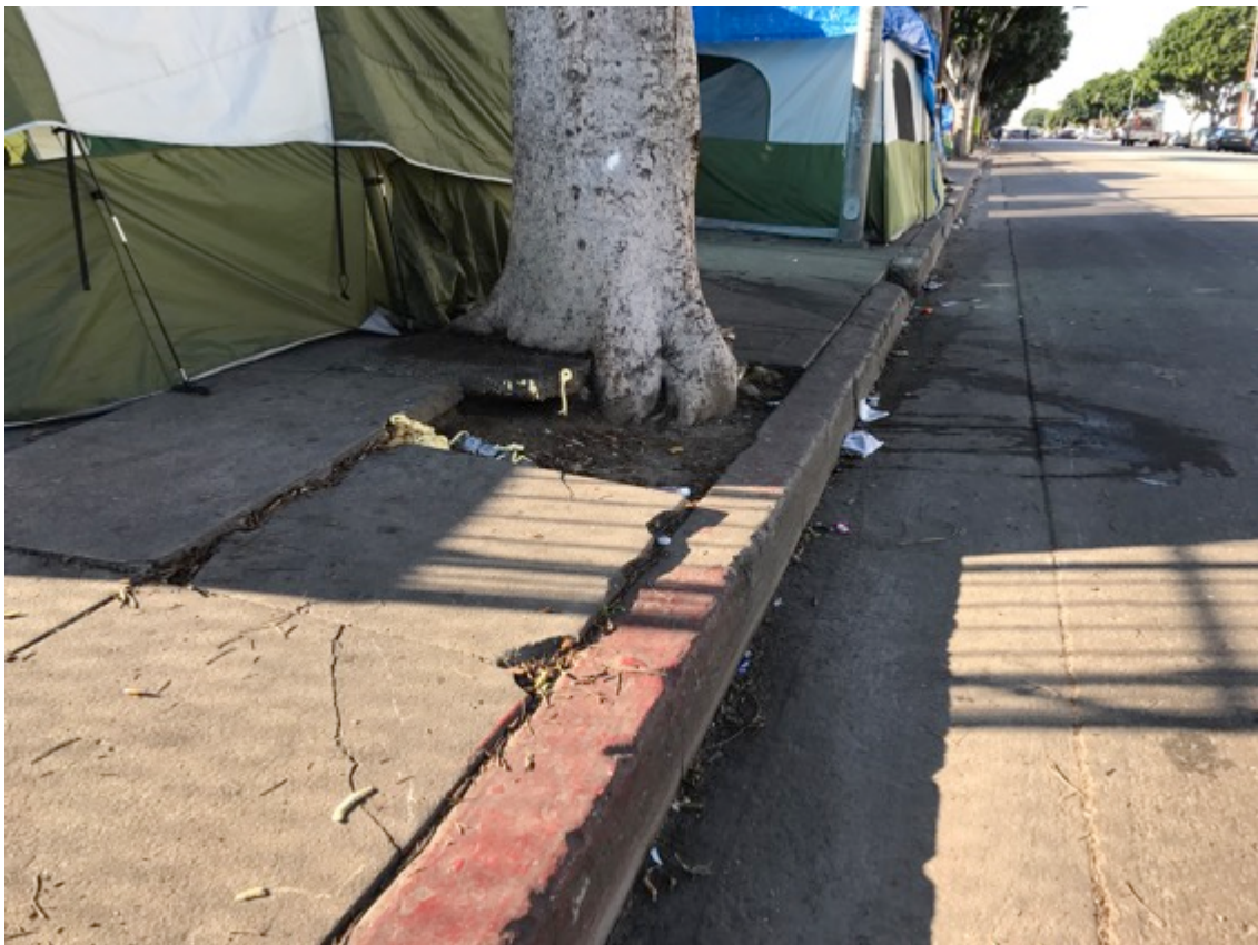
Tree well imbedded in trunk / Sidewalk raised (Tree#2)
