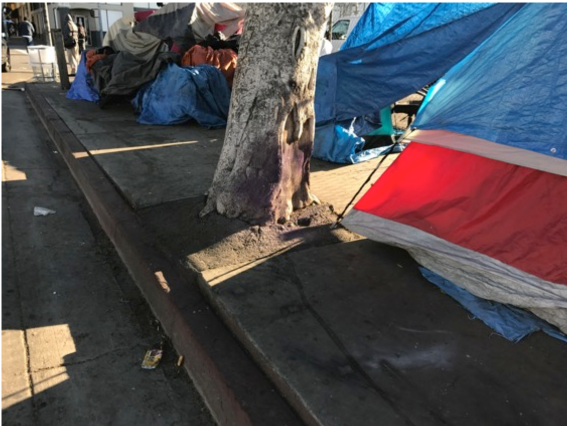
Decay at tree base / Sidewalk raised (Tree#1)
