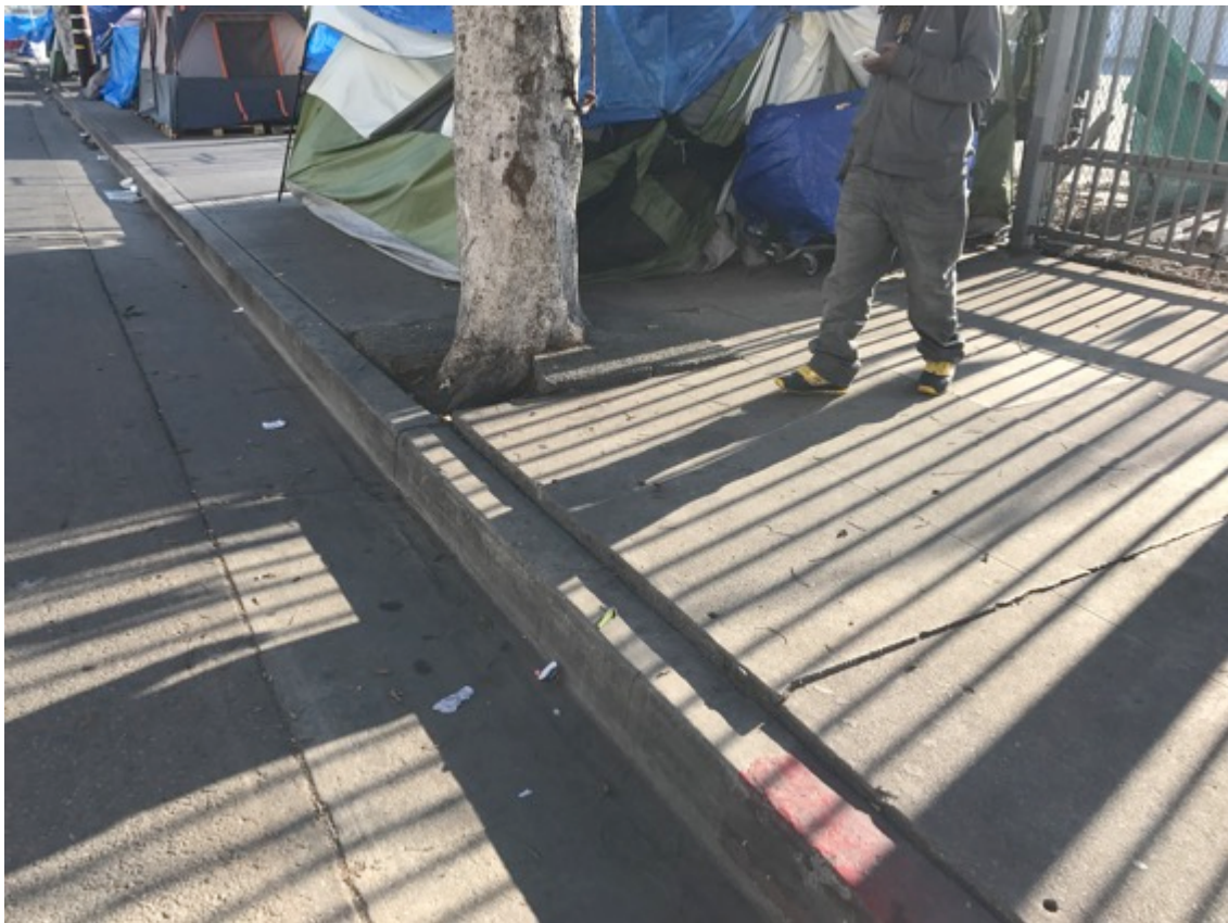
Tree well imbedded in trunk / Sidewalk raised (Tree #4)
