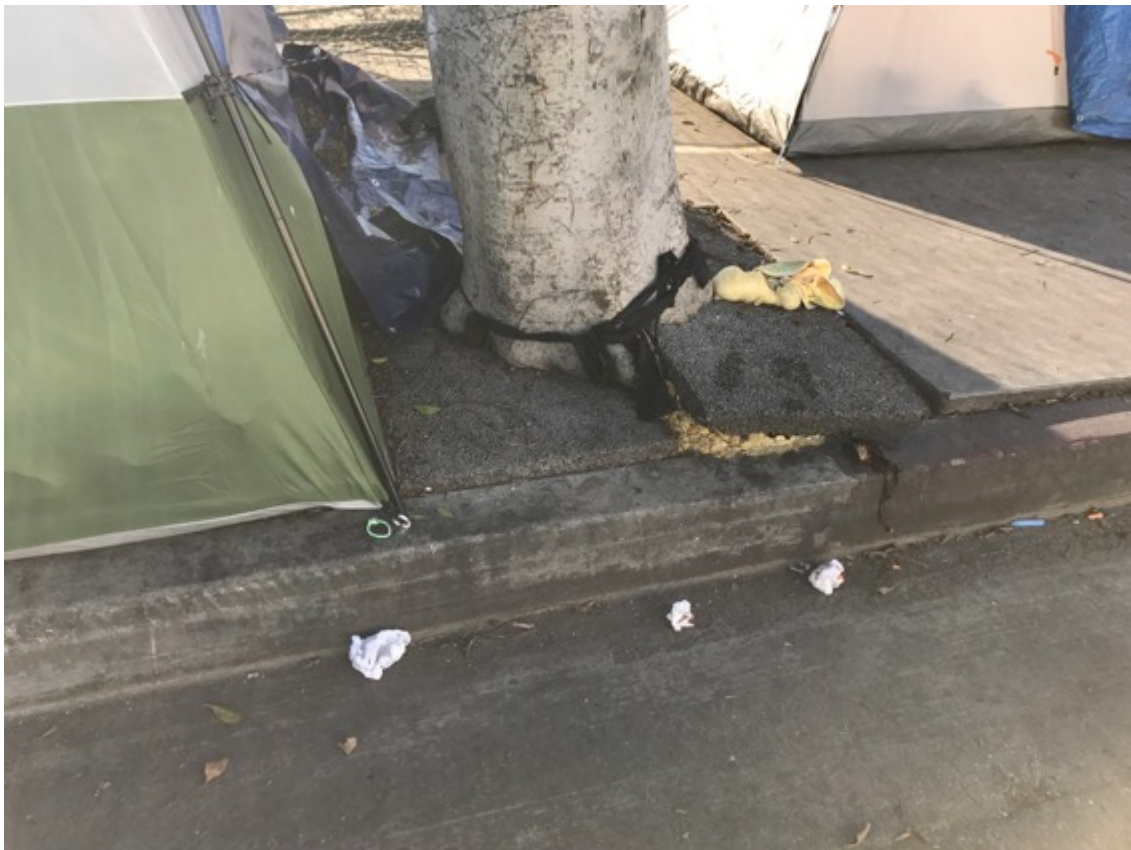
Tree well imbedded in trunk / Sidewalk raised (Tree#3)
