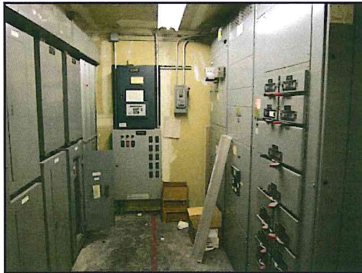
9 : Main electrical panel
