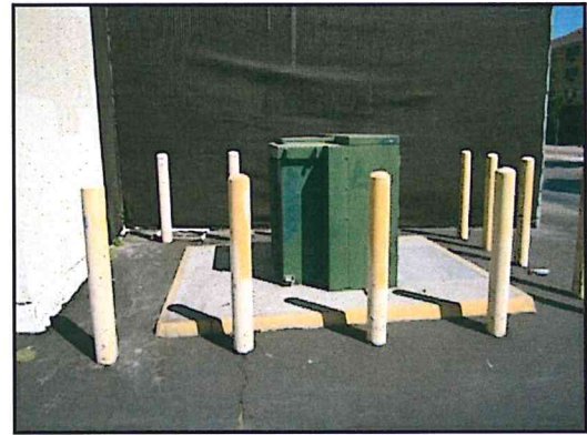
16 : Utility-owned, pad-mounted electrical transformer
