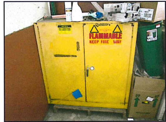
12 : Fire storage cabinet in rear utility area
