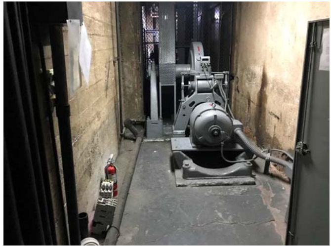
26. Elevator machinery in the 6381 building.
