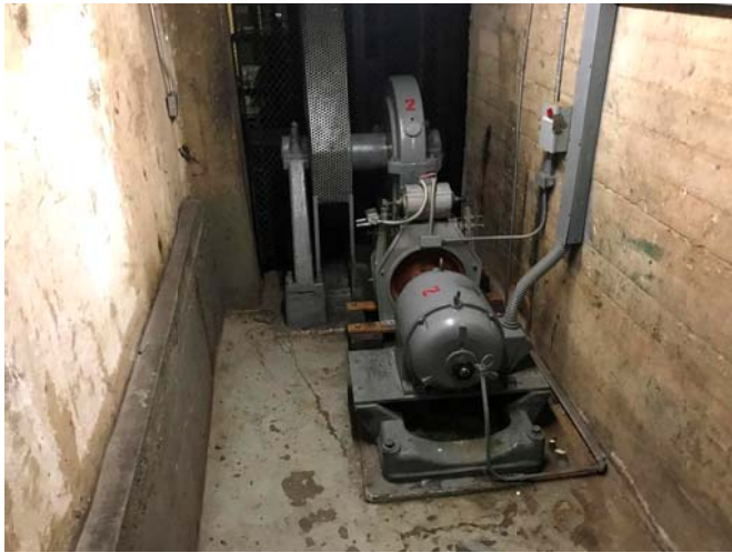
25. Elevator machinery in the 6381 building.
