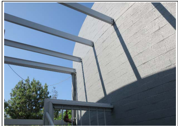
West elevation, detail of metal tie beams at top of exterior stairwell (ARG, 2020)
