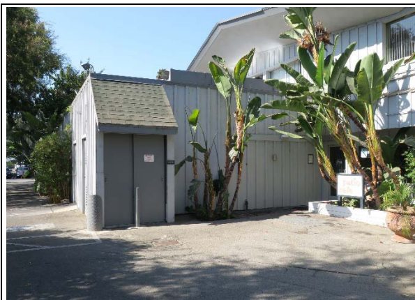
Detail of east elevation, view southwest. The one-story volume is an addition (ARG, 2020)
