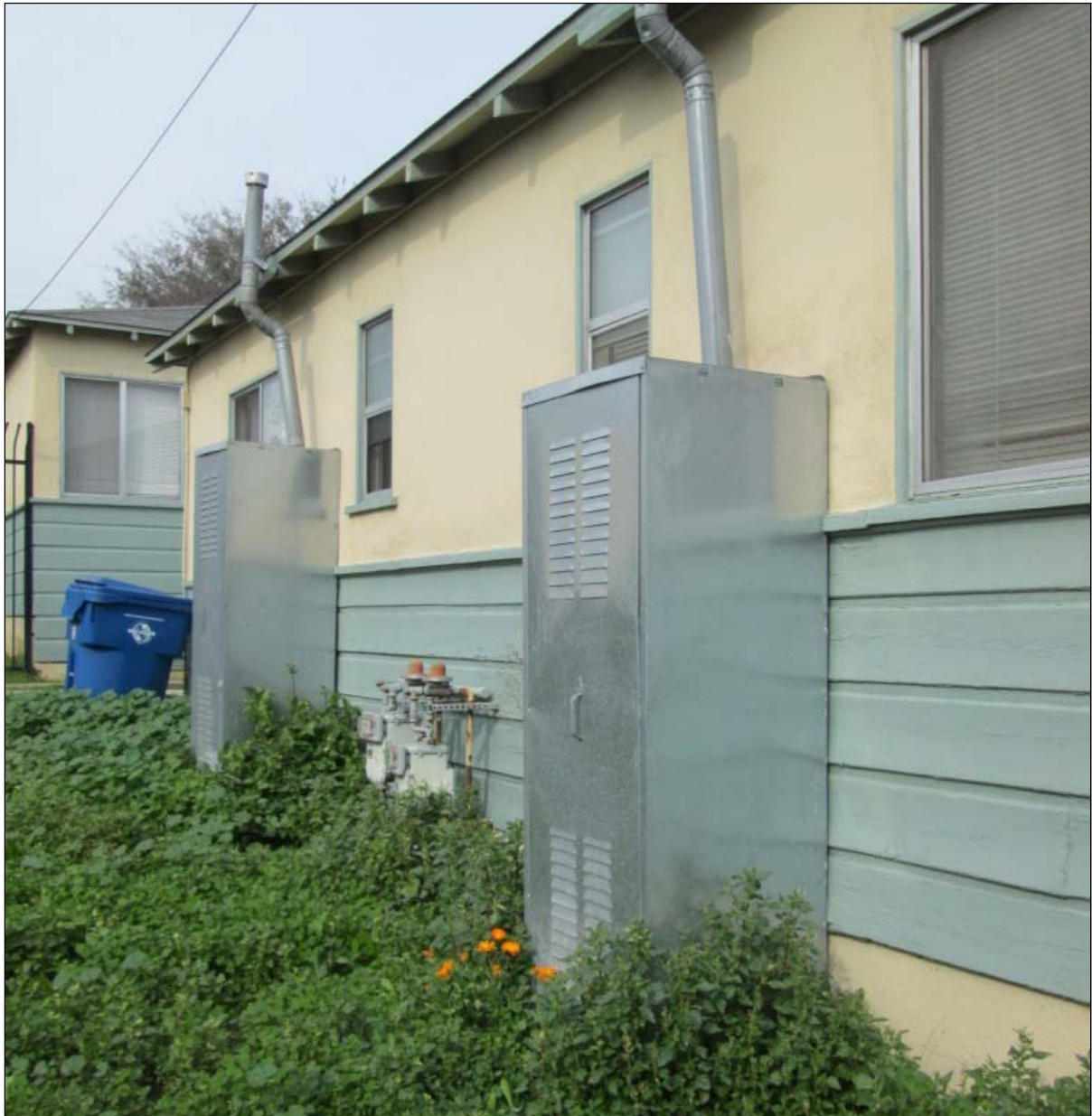
Figure 8: Exterior water heaters, typical (1/18/17)
