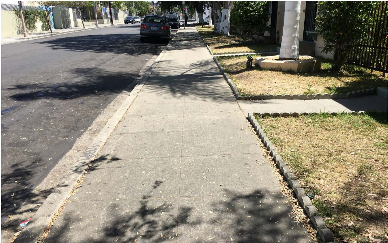
6. Condition of abutting sidewalk, facing north on Grand View St.
