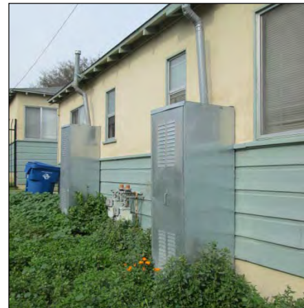
Exterior water heaters
