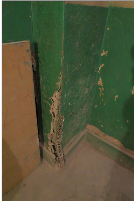
Image 23: Subject property, basement, detail of damage to wall by stairs (Chattel, 2019)
