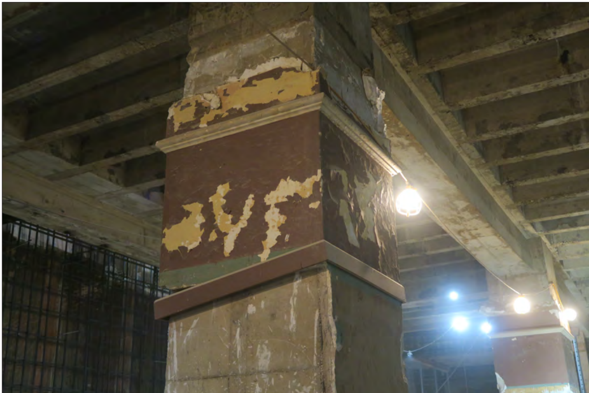
Image 41: Subject property, basement, detail of damage to column (Chattel, 2019)
