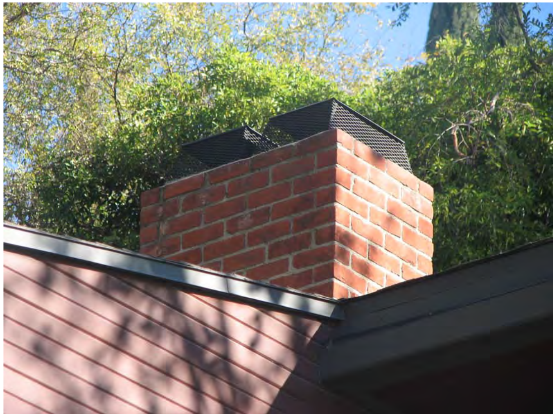
Bonnet House, chimney 2256 El Contento Drive, December 4, 2018 (Photograph by Charles J. Fisher)
