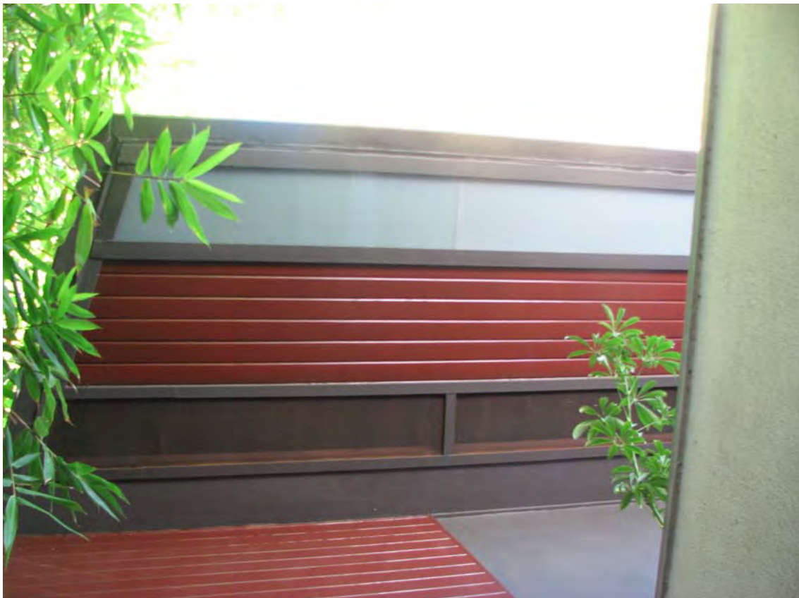
Bonnet House, underside of main eave, 2256 El Contento Drive, December 4, 2018 (Photograph by Charles J. Fisher)
