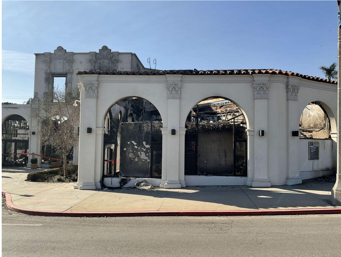
Remains of the Palisades Business Block. View from Sunset Blvd, east of Via de La Paz.
