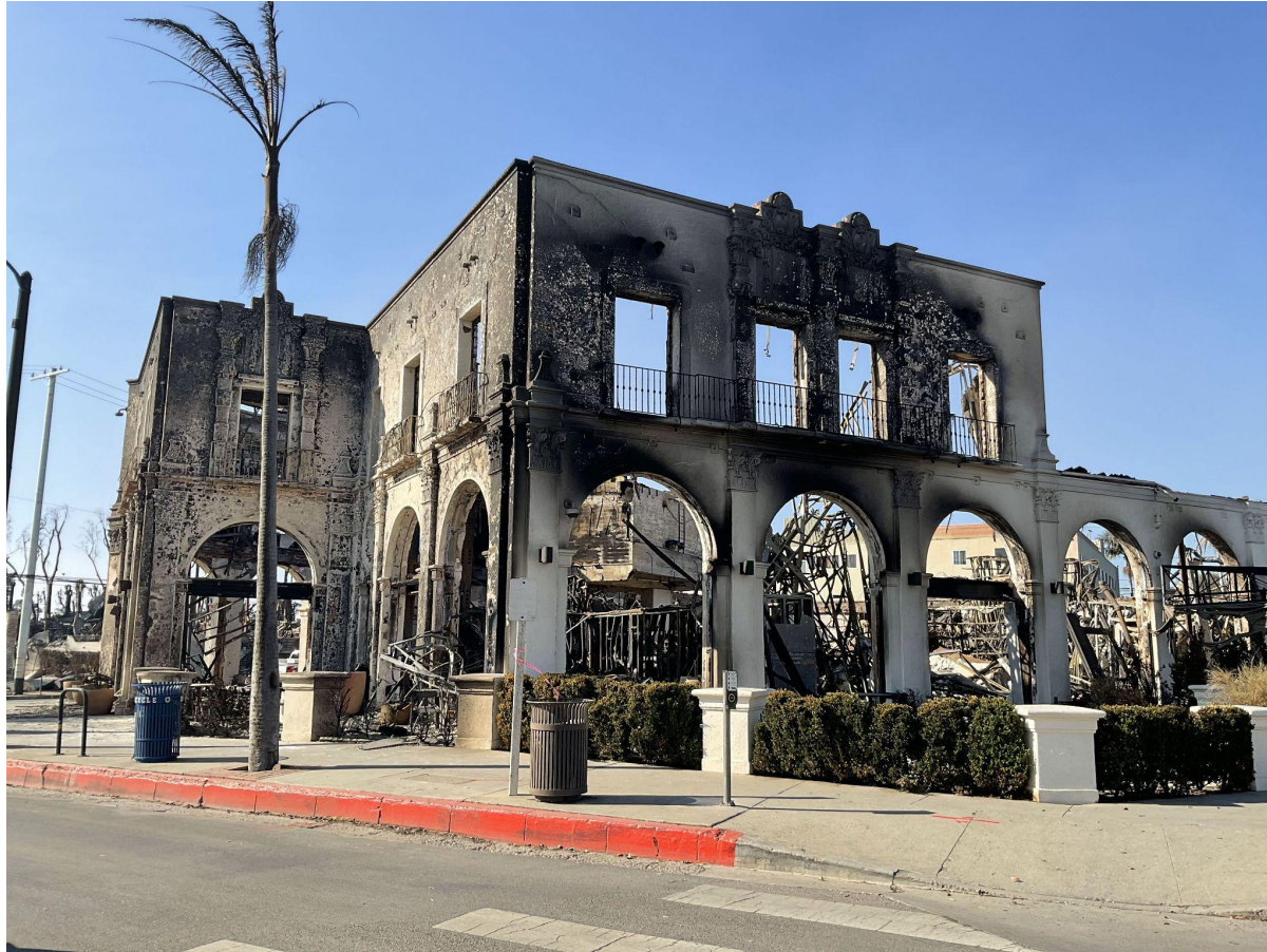
Remains of the Palisades Business Block. View from Swarthmore at Sunset Blvd.
