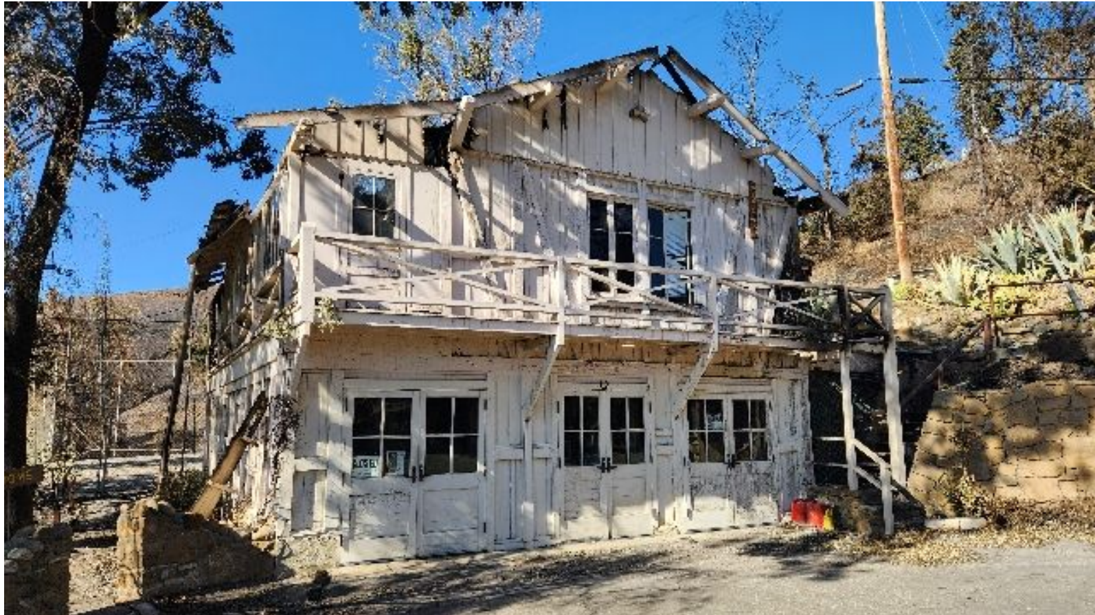
Remains of the garage
