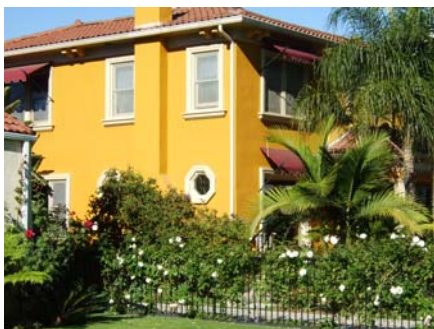
The octagonal windows and the styrofoam frames and sills that have been added to this Italian Renaissance Revival home are inconsistent with the original architectural style and diminish the historic integrity of the home.
