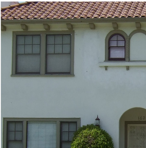
Historic windows, shown below, tend to have a configuration that provides scale and harmony on the facade; depth and texture; and arrangements in groups. Inappropriate windows, shown above, tend not to relate to the facade dimensions, are installed flush to the wall and may have unsightly ornamentation such as faux muntins.
