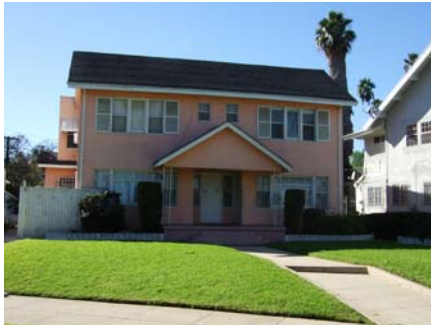
The original porch columns on this house have been replaced with metal devices that are out of scale and substantially alter the look of the house.
