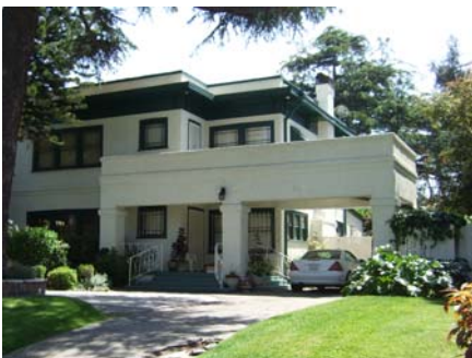
The addition of safety railing may be appropriate however such features should be simple in style and should not alter the intended design of the porch.
