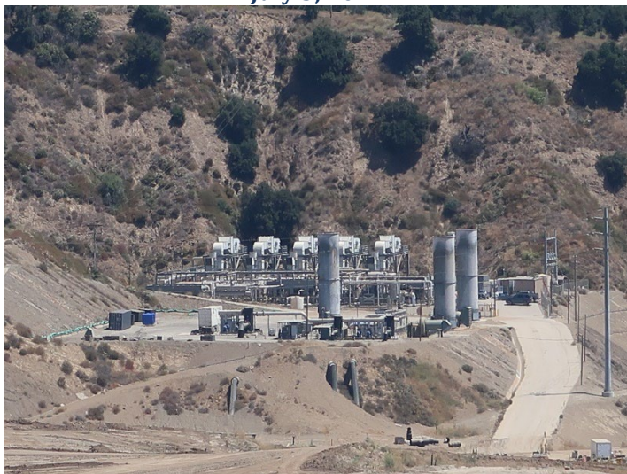
Photo 143: Flares 9, 10, 11 and Gas-to-Energy Facility: July 3, 2024
