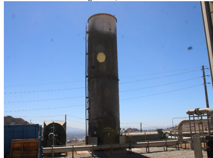
Photo 148: Flares 9, 10, 11 and Gas-to-Energy Facility: August 19, 2024
