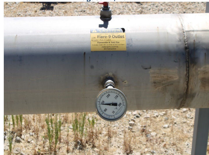
Photo 152: Flares 9, 10, 11 and Gas-to-Energy Facility: August 19, 2024
