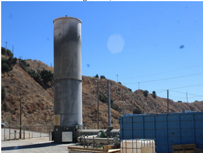
Photo 147: Flares 9, 10, 11 and Gas-to-Energy Facility: August 19, 2024
