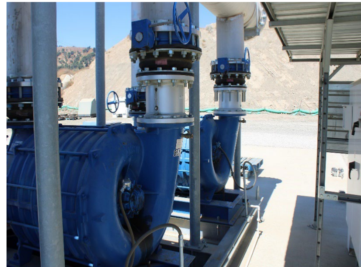
Photo 158: Flares 9, 10, 11 and Gas-to-Energy Facility: August 19, 2024
