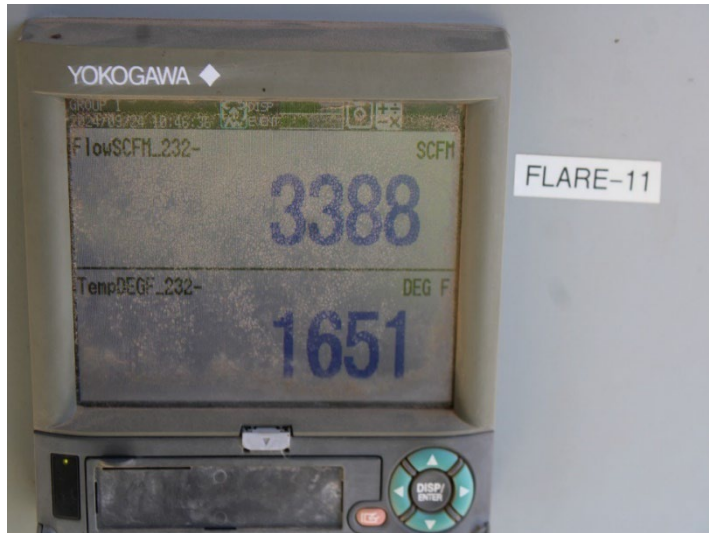
Photo 169: Flares 9, 10, 11 and Gas-to-Energy Facility: September 24, 2024
