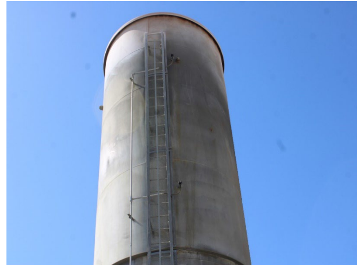
Photo 162: Flares 9, 10, 11 and Gas-to-Energy Facility: September 24, 2024
