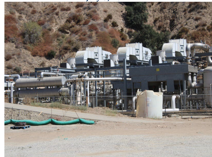
Photo 144: Flares 9, 10, 11 and Gas-to-Energy Facility: August 19, 2024
