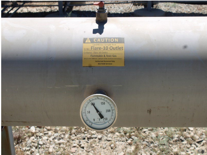
Photo 149: Flares 9, 10, 11 and Gas-to-Energy Facility: August 19, 2024
