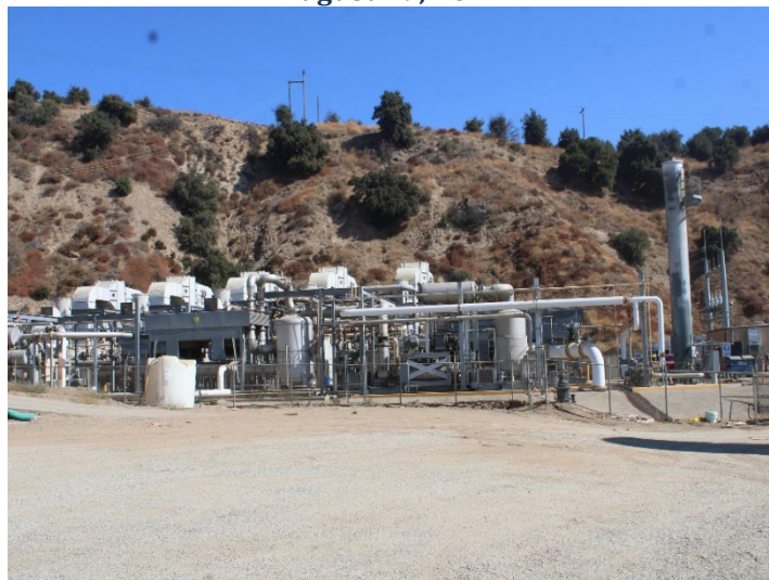
Photo 159: Flares 9, 10, 11 and Gas-to-Energy Facility: September 24, 2024
