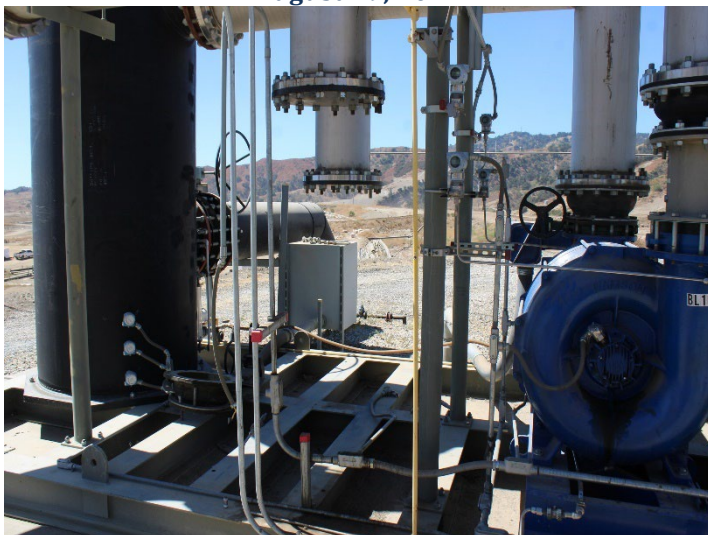
Photo 155: Flares 9, 10, 11 and Gas-to-Energy Facility: August 19, 2024
