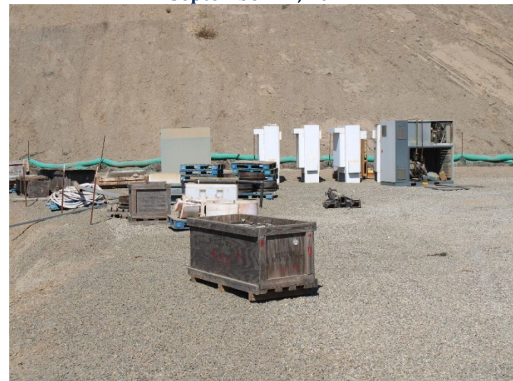
Photo 172: Flares 9, 10, 11 and Gas-to-Energy Facility: September 24, 2024
