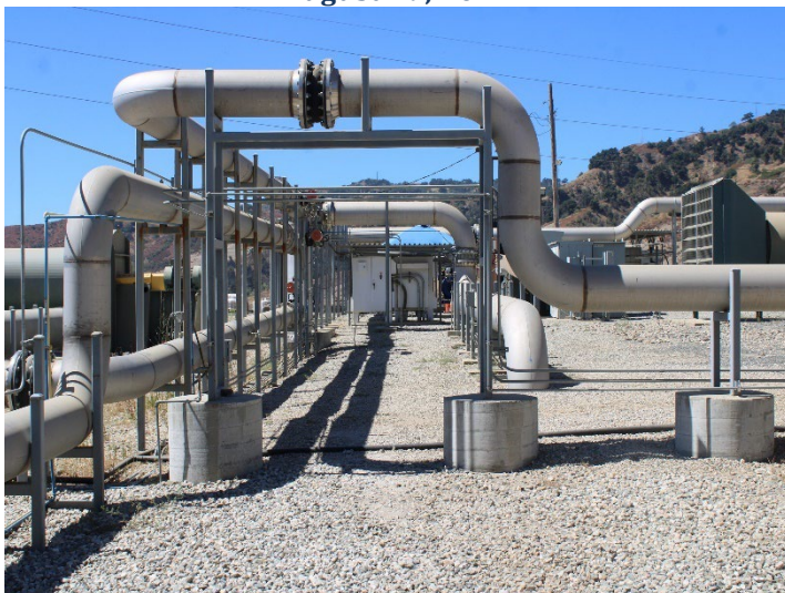
Photo 151: Flares 9, 10, 11 and Gas-to-Energy Facility: August 19, 2024
