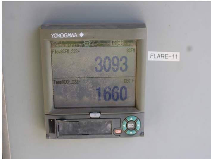
Photo 157: Flares 9, 10, 11 and Gas-to-Energy Facility: August 19, 2024
