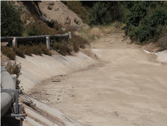
Photo 5: Basin A: July 3, 2024
