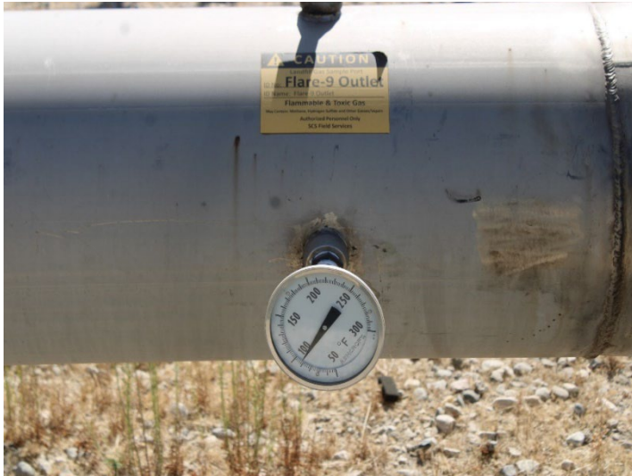
Photo 165: Flares 9, 10, 11 and Gas-to-Energy Facility: September 24, 2024
