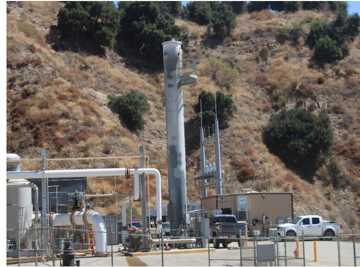
Photo 146: Flares 9, 10, 11 and Gas-to-Energy Facility: August 19, 2024
