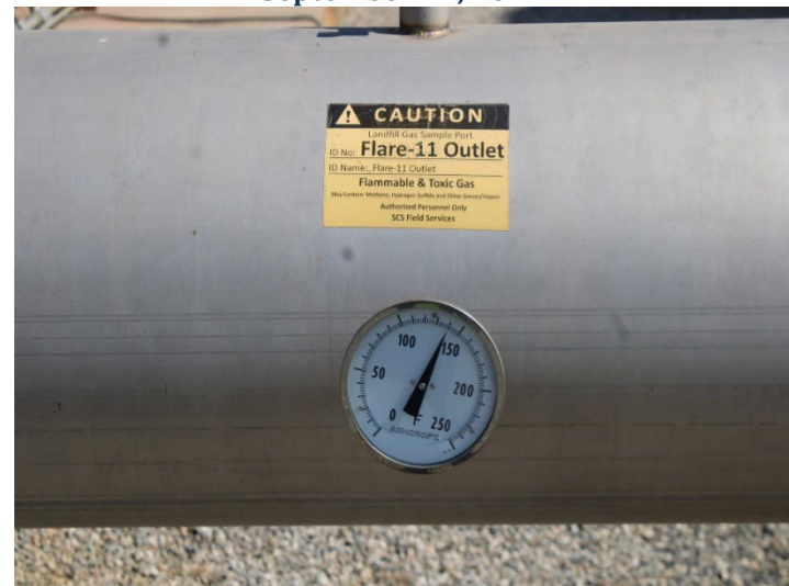
Photo 164: Flares 9, 10, 11 and Gas-to-Energy Facility: September 24, 2024
