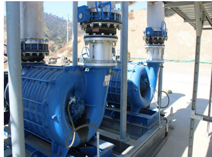
Photo 170: Flares 9, 10, 11 and Gas-to-Energy Facility: September 24, 2024
