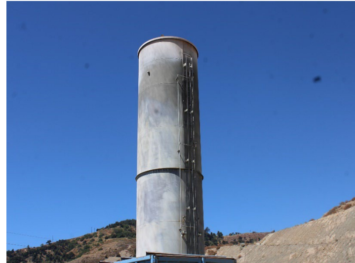
Photo 150: Flares 9, 10, 11 and Gas-to-Energy Facility: August 19, 2024
