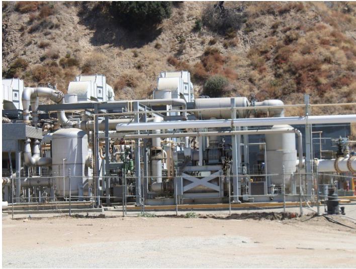
Photo 145: Flares 9, 10, 11 and Gas-to-Energy Facility: August 19, 2024
