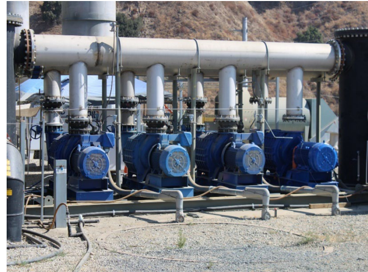
Photo 174: Flares 9, 10, 11 and Gas-to-Energy Facility: September 24, 2024
