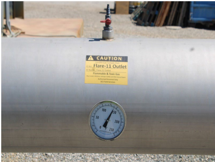
Photo 153: Flares 9, 10, 11 and Gas-to-Energy Facility: August 19, 2024
