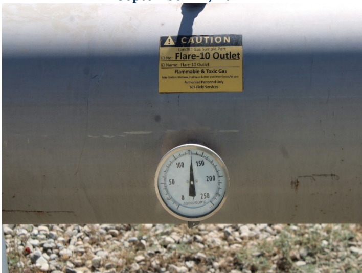
Photo 163: Flares 9, 10, 11 and Gas-to-Energy Facility: September 24, 2024
