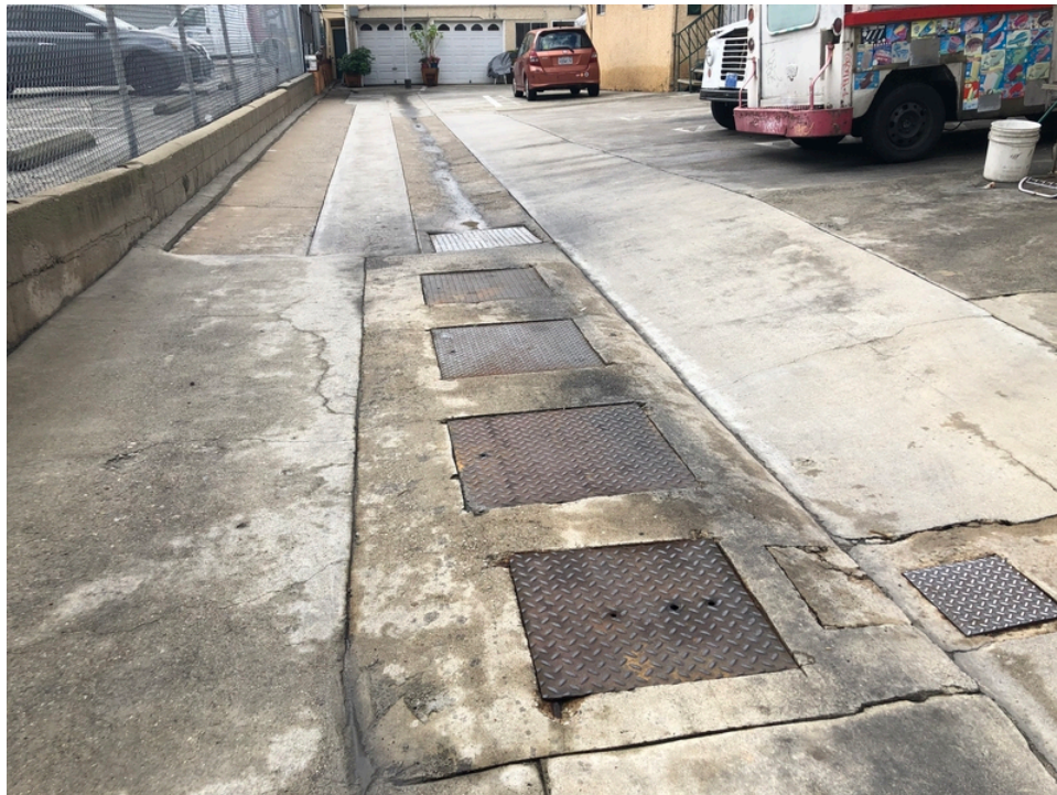
8. View of three-chambered grease interceptor in commissary area.
