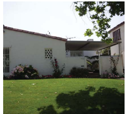
This patio cover is inappropriate and disrupts the intended form and use of the outdoor space.
