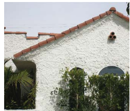
Heavily textured stucco is a modern look and detracts from the appearance of this structure.
