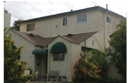
Aluminum slider windows are not an appropriate choice for Period Revival homes.
