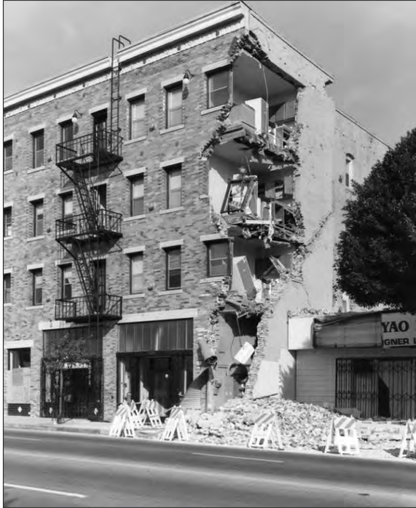
Damage sustained to an apartment building on Hollywood Boulevard as a result of the Northridge earthquake in 1994. (Photo courtesy of Los Angeles Public Library)
