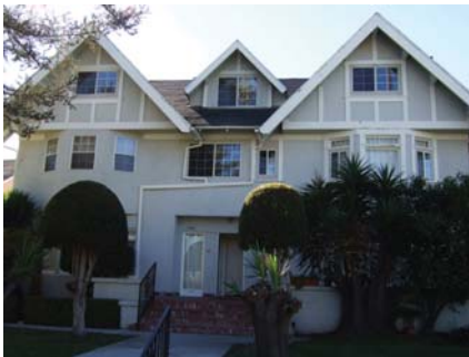
The modern windows that have been added to this home are poorly scaled and dramatically alter the home's original appearance.
