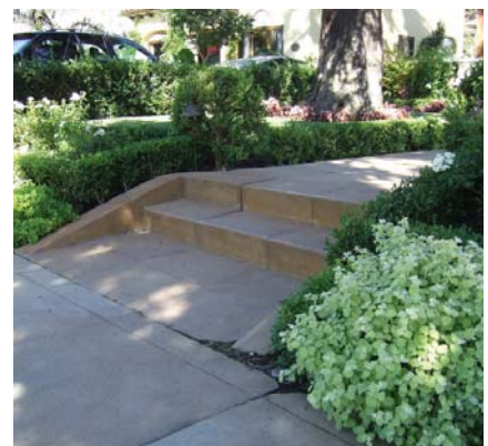
A typical front walkway and steps are shown. Concrete colors and score patterns should be carefully preserved.
