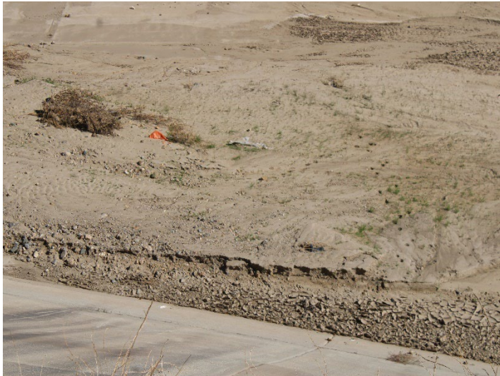
Photo 337: Basin B: November 6, 2025
