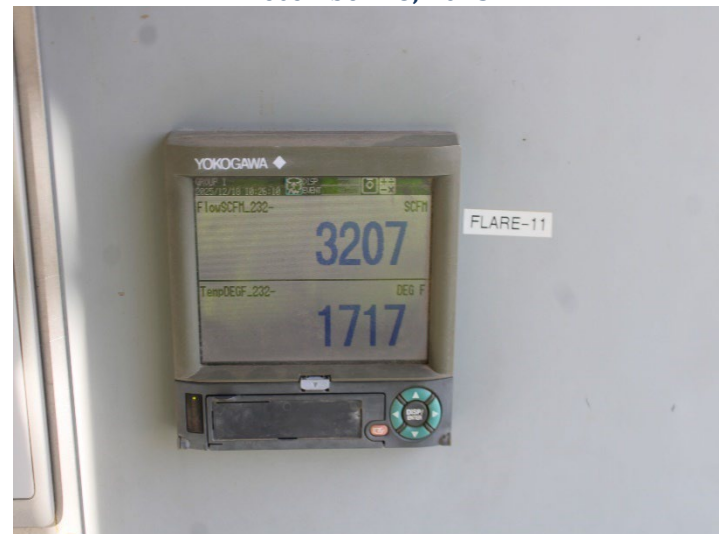
Photo 284: Flares 9, 10, 11 and Gas-to-Energy Facility: December 18, 2025
