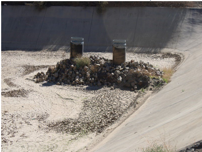
Photo 339: Basin B: November 6, 2025
