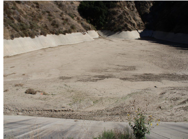
Photo 334: Basin B: November 6, 2025
