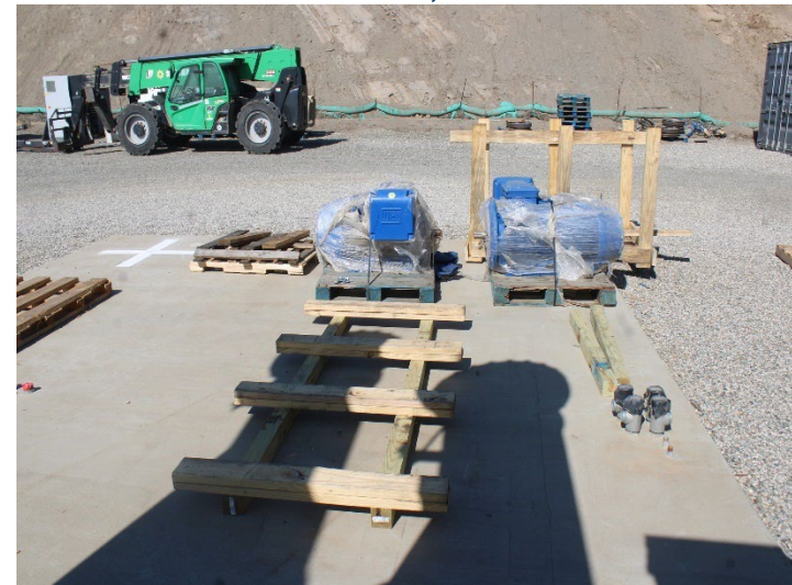
Photo 260: Flares 9, 10, 11 and Gas-to-Energy Facility: October 8, 2025
