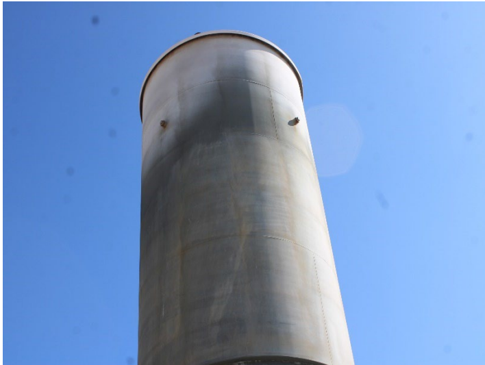
Photo 253: Flares 9, 10, 11 and Gas-to-Energy Facility: October 8, 2025
