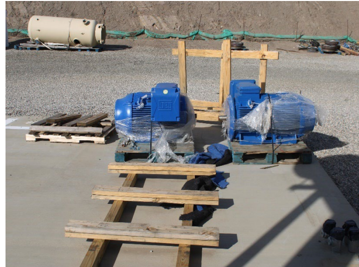
Photo 286: Flares 9, 10, 11 and Gas-to-Energy Facility: December 18, 2025
