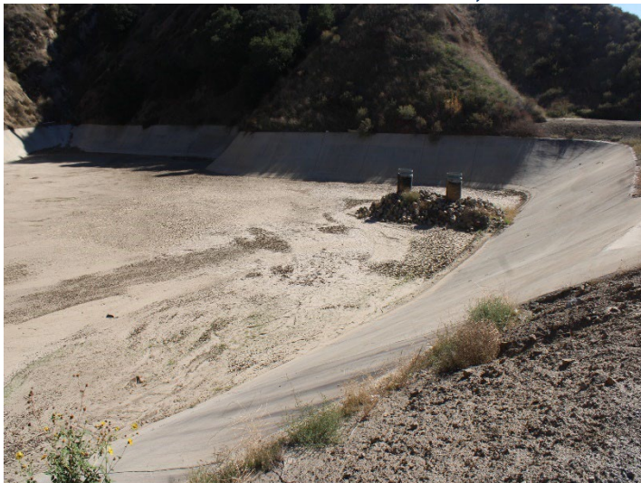
Photo 335: Basin B: November 6, 2025
