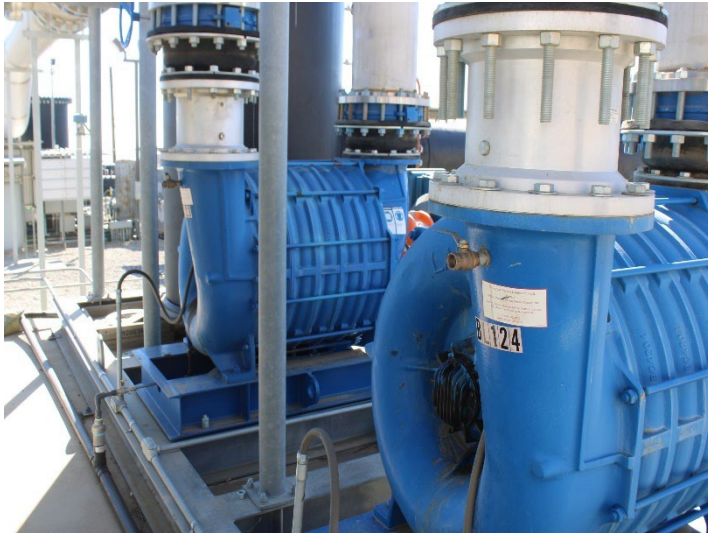
Photo 269: Flares 9, 10, 11 and Gas-to-Energy Facility: November 6, 2025
