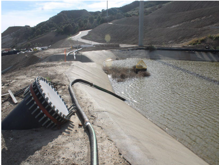
Photo 13: Basin A: December 18, 2025
