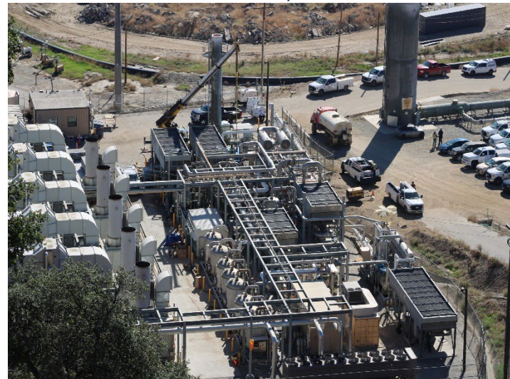
Photo 276: Flares 9, 10, 11 and Gas-to-Energy Facility: November 6, 2025
