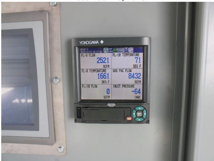
Photo 283: Flares 9, 10, 11 and Gas-to-Energy Facility: December 18, 2025
