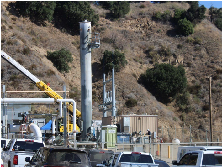
Photo 275: Flares 9, 10, 11 and Gas-to-Energy Facility: November 6, 2025
