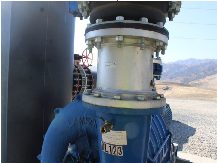
Photo 259: Flares 9, 10, 11 and Gas-to-Energy Facility: October 8, 2025
