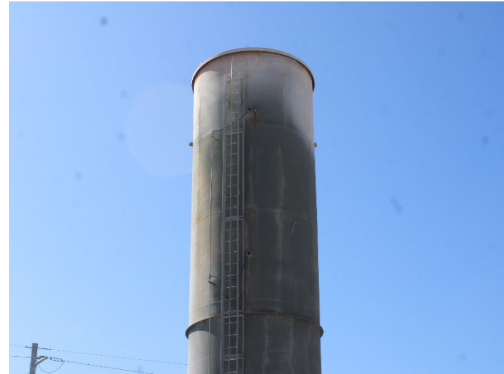
Photo 254: Flares 9, 10, 11 and Gas-to-Energy Facility: October 8, 2025
