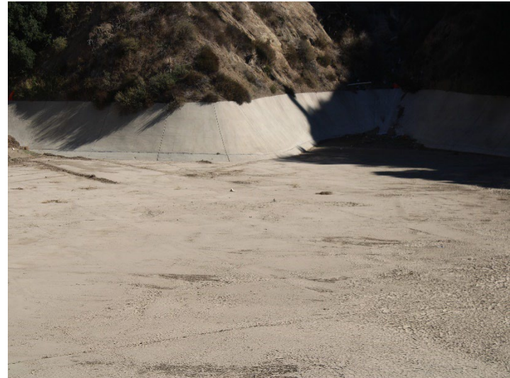
Photo 338: Basin B: November 6, 2025
