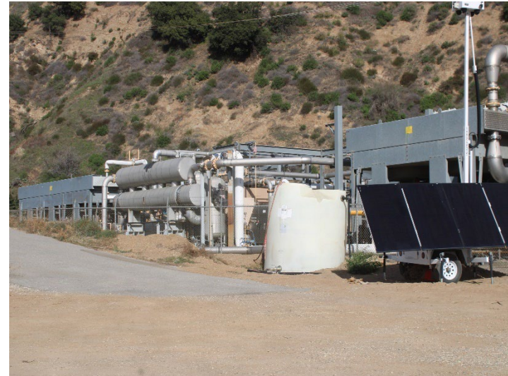
Photo 290: Flares 9, 10, 11 and Gas-to-Energy Facility: December 18, 2025
