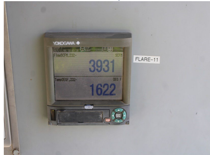
Photo 268: Flares 9, 10, 11 and Gas-to-Energy Facility: November 6, 2025
