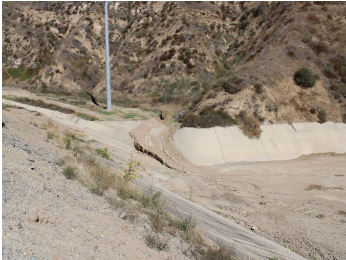
Photo 333: Basin B: November 6, 2025
