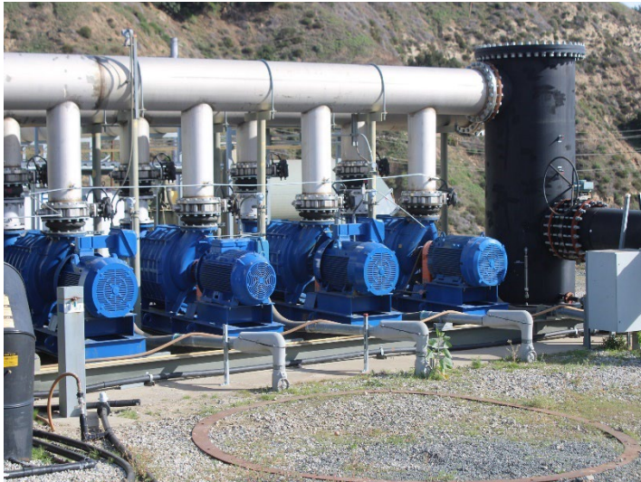
Photo 289: Flares 9, 10, 11 and Gas-to-Energy Facility: December 18, 2025
