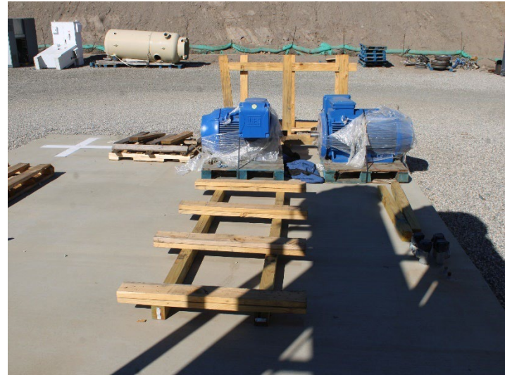
Photo 270: Flares 9, 10, 11 and Gas-to-Energy Facility: November 6, 2025
