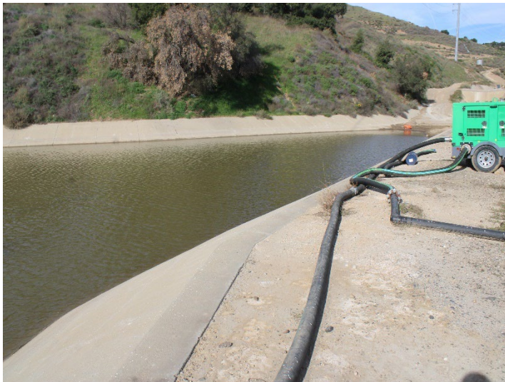
Photo 15: Basin A: December 18, 2025
