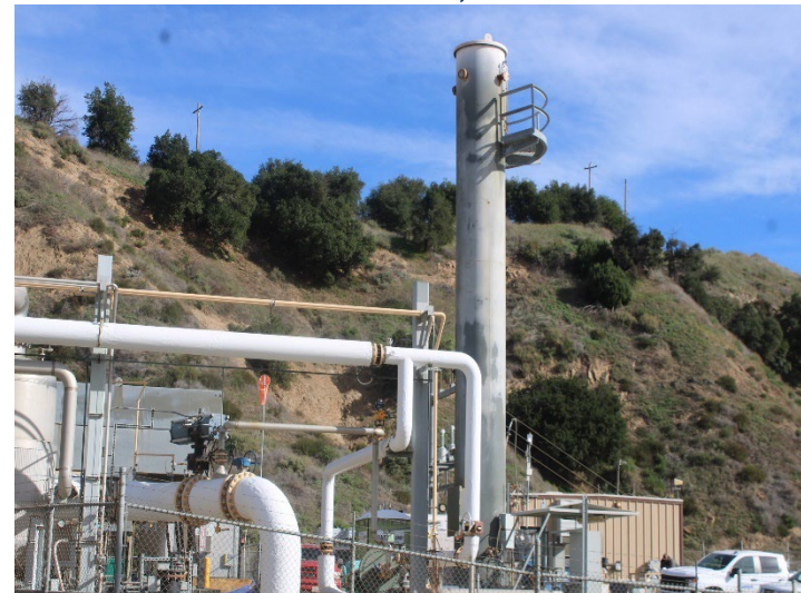
Photo 292: Flares 9, 10, 11 and Gas-to-Energy Facility: December 18, 2025
