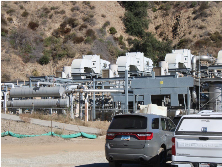
Photo 273: Flares 9, 10, 11 and Gas-to-Energy Facility: November 6, 2025
