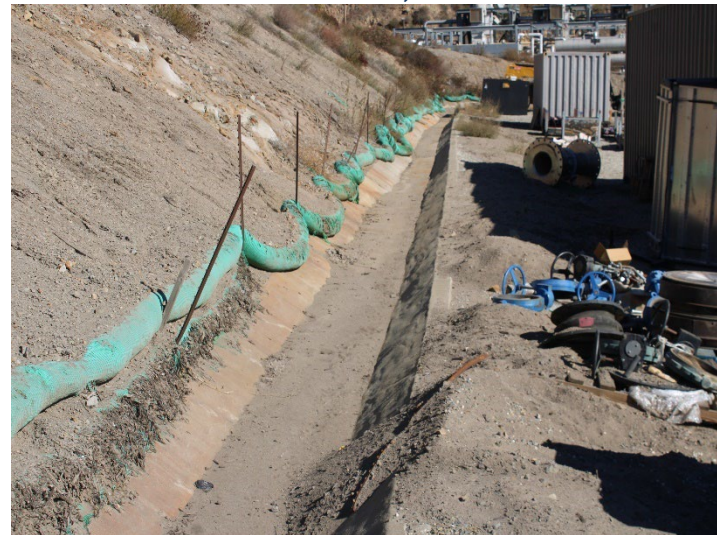
Photo 272: Flares 9, 10, 11 and Gas-to-Energy Facility: November 6, 2025
