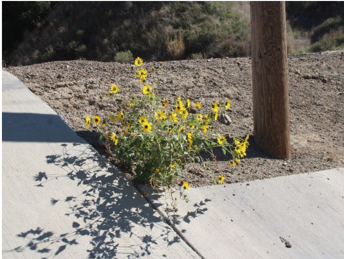
Photo 341: Basin B: November 6, 2025
