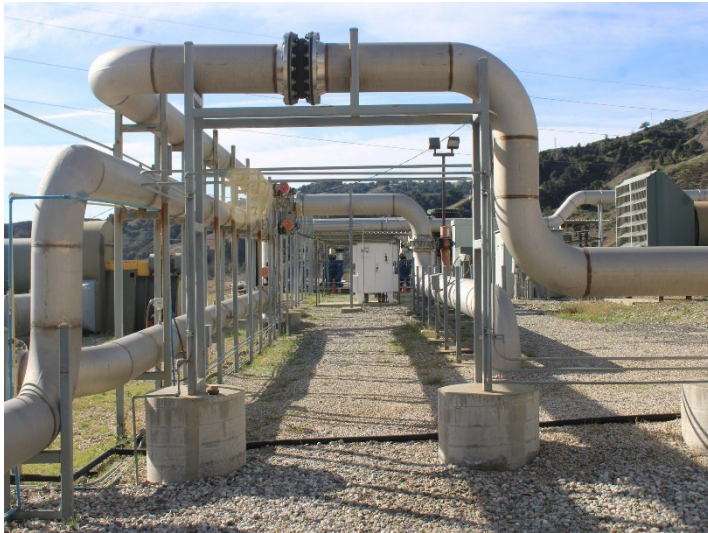
Photo 281: Flares 9, 10, 11 and Gas-to-Energy Facility: December 18, 2025
