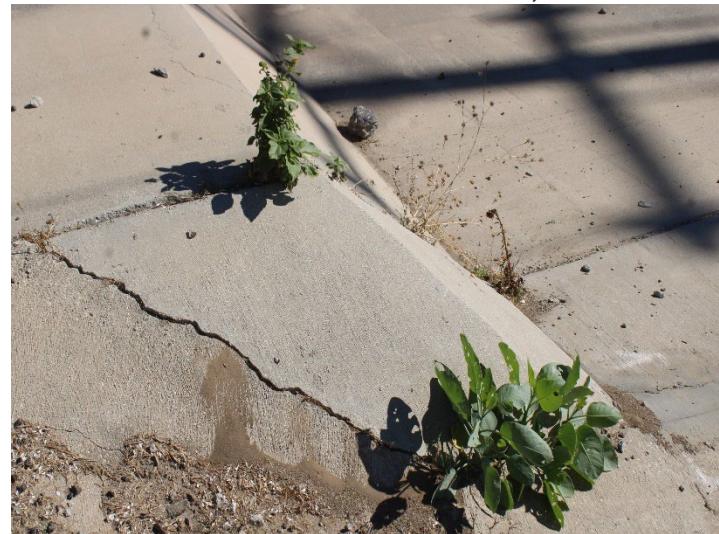
Photo 340: Basin B: November 6, 2025
