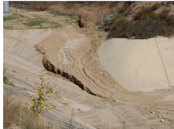
Photo 336: Basin B: November 6, 2025
