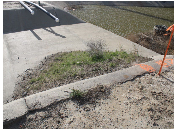
Photo 16: Basin A: December 18, 2025
