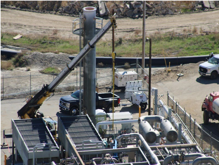
Photo 277: Flares 9, 10, 11 and Gas-to-Energy Facility: November 6, 2025
