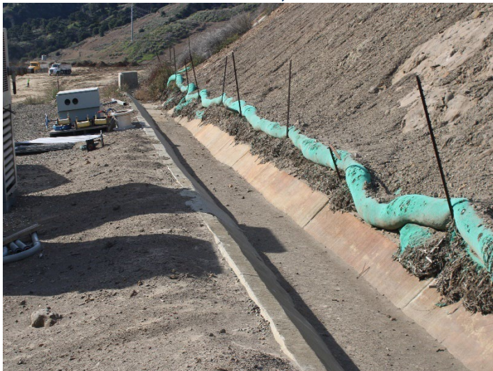
Photo 287: Flares 9, 10, 11 and Gas-to-Energy Facility: December 18, 2025
