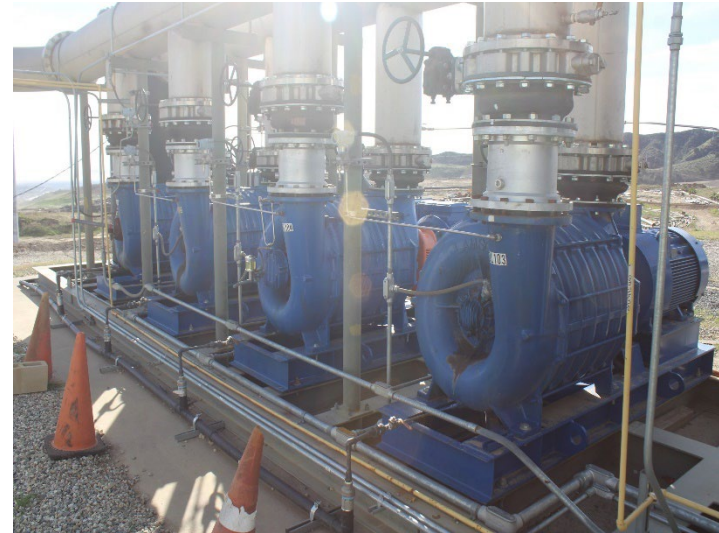
Photo 282: Flares 9, 10, 11 and Gas-to-Energy Facility: December 18, 2025
