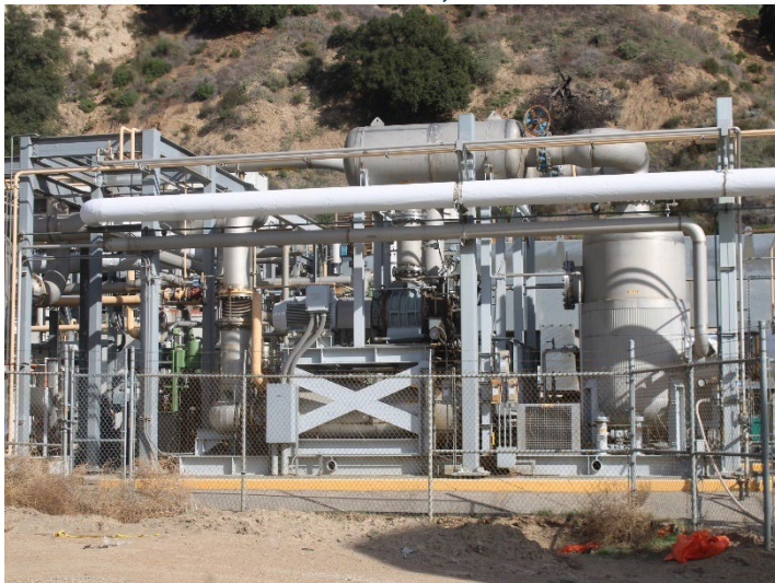
Photo 291: Flares 9, 10, 11 and Gas-to-Energy Facility: December 18, 2025
