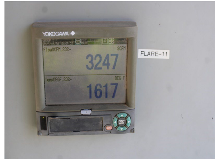
Photo 258: Flares 9, 10, 11 and Gas-to-Energy Facility: October 8, 2025
