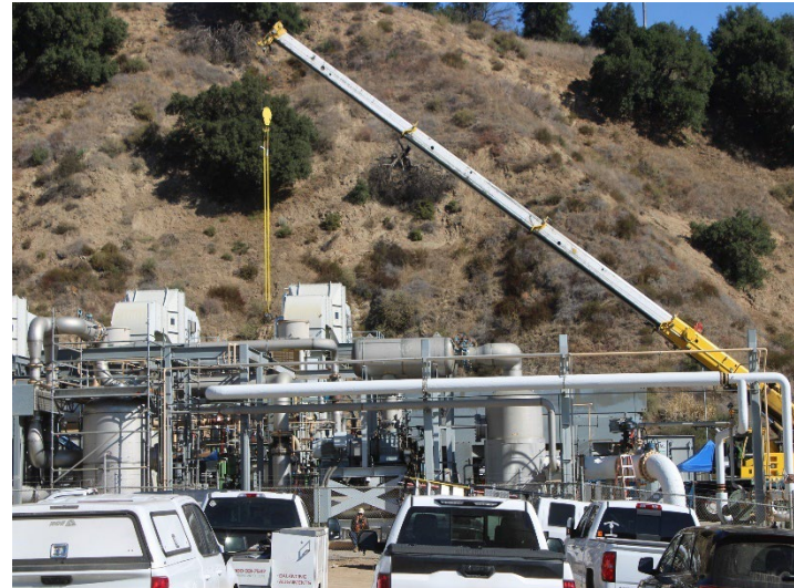
Photo 274: Flares 9, 10, 11 and Gas-to-Energy Facility: November 6, 2025
