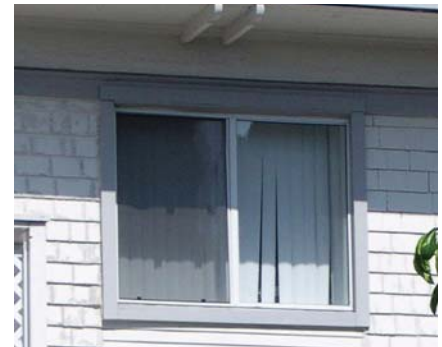
An inappropriately sized aluminum window diminishes the historic value of a house.
