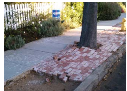
Landscape parkways are intended as green space and should not be covered in hardscape.
