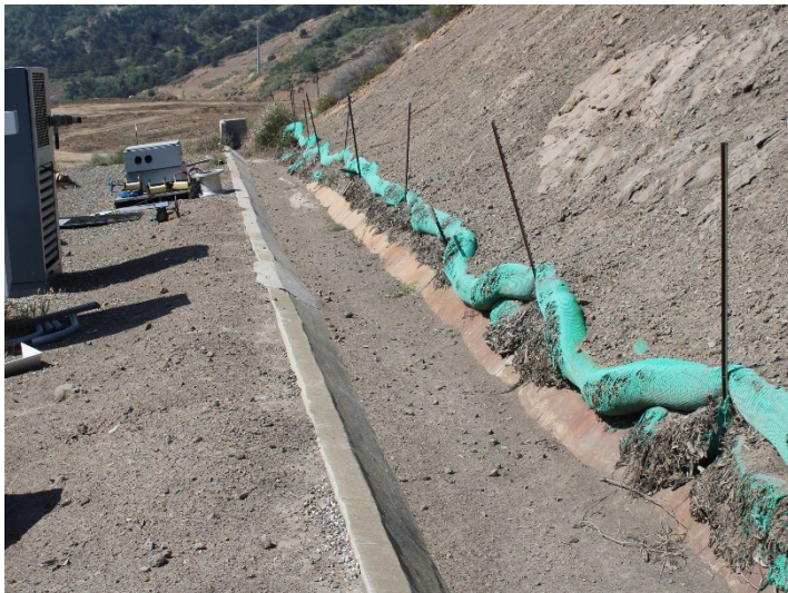
Photo 223: Flares 9, 10, 11 and Gas-to-Energy Facility: April 9, 2026
