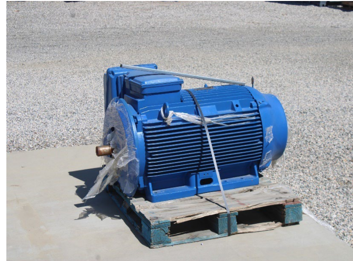
Photo 234: Flares 9, 10, 11 and Gas-to-Energy Facility: May 21, 2026
