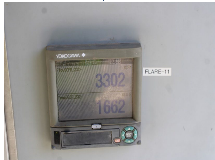
Photo 244: Flares 9, 10, 11 and Gas-to-Energy Facility: June 11, 2026
