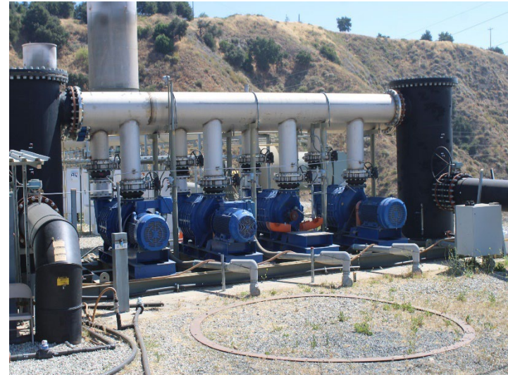
Photo 238: Flares 9, 10, 11 and Gas-to-Energy Facility: May 21, 2026
