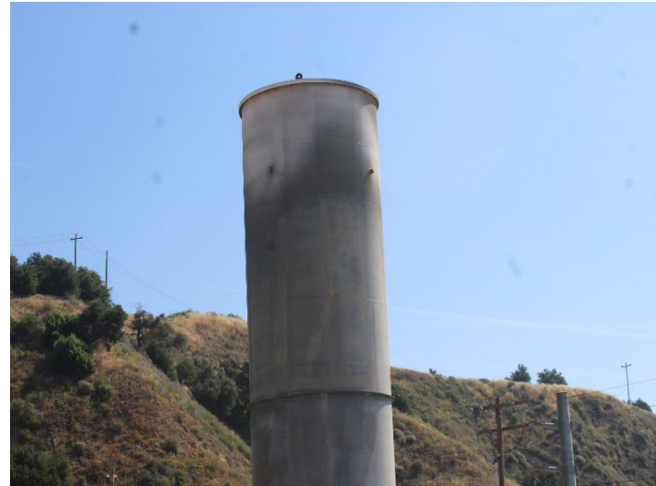
Photo 214: Flares 9, 10, 11 and Gas-to-Energy Facility: April 9, 2026
