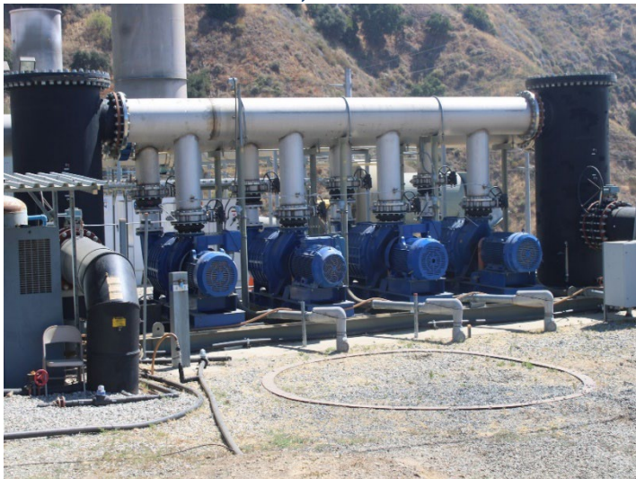
Photo 247: Flares 9, 10, 11 and Gas-to-Energy Facility: June 11, 2026
