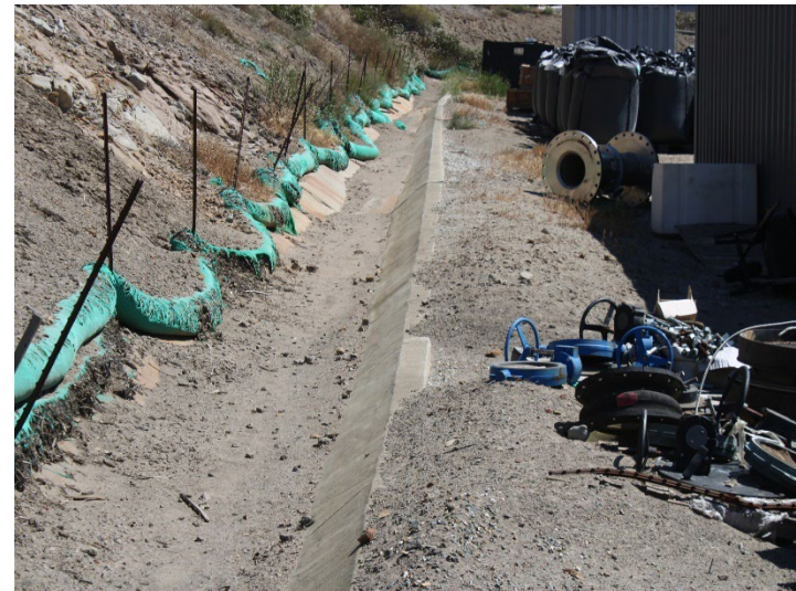
Photo 236: Flares 9, 10, 11 and Gas-to-Energy Facility: May 21, 2026
