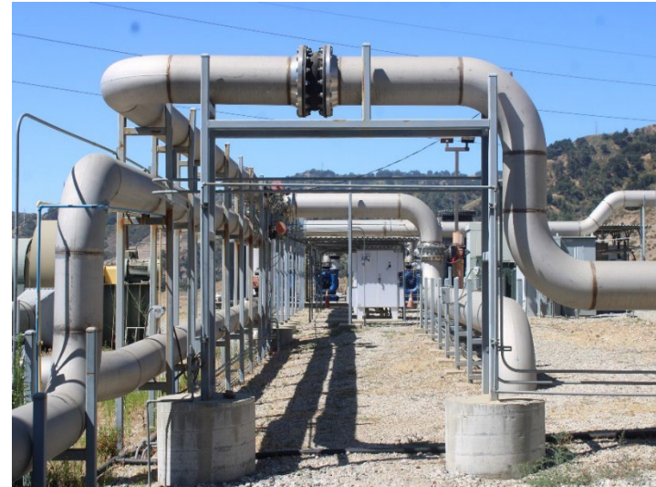
Photo 242: Flares 9, 10, 11 and Gas-to-Energy Facility: June 11, 2026
