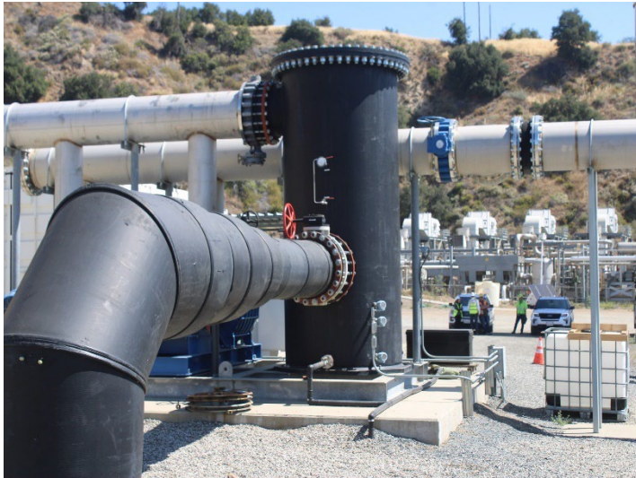
Photo 237: Flares 9, 10, 11 and Gas-to-Energy Facility: May 21, 2026
