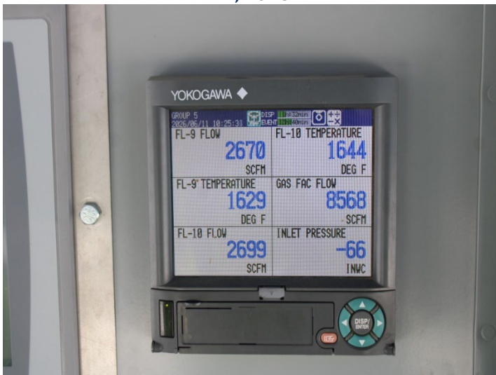
Photo 243: Flares 9, 10, 11 and Gas-to-Energy Facility: June 11, 2026
