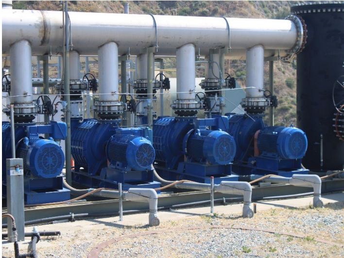
Photo 225: Flares 9, 10, 11 and Gas-to-Energy Facility: April 9, 2026
