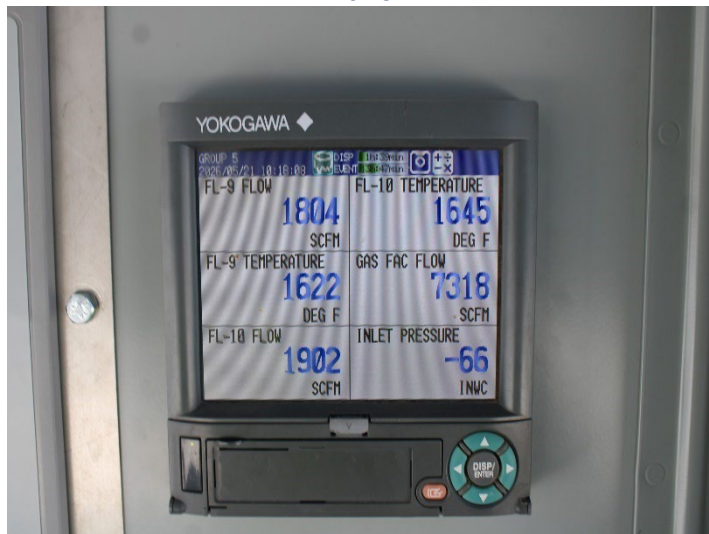
Photo 231: Flares 9, 10, 11 and Gas-to-Energy Facility: May 21, 2026
