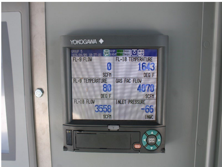
Photo 219: Flares 9, 10, 11 and Gas-to-Energy Facility: April 9, 2026
