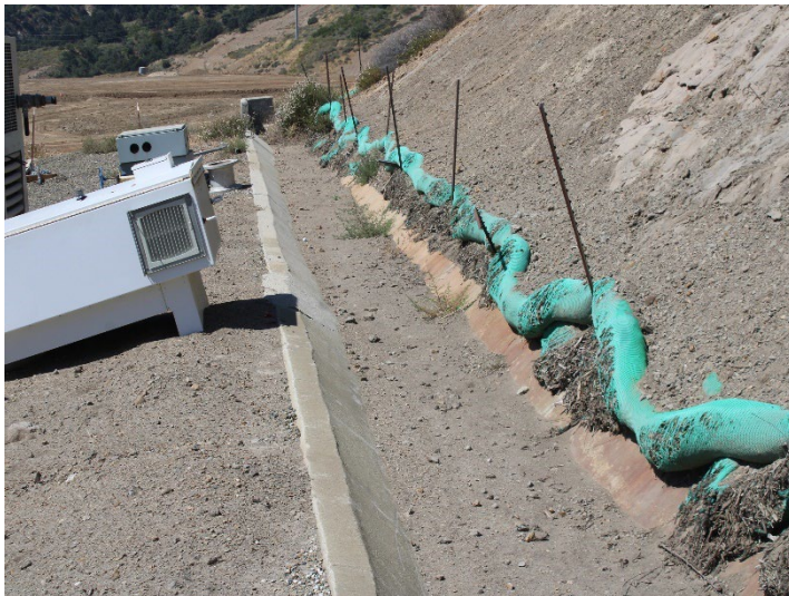
Photo 235: Flares 9, 10, 11 and Gas-to-Energy Facility: May 21, 2026
