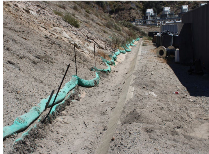
Photo 246: Flares 9, 10, 11 and Gas-to-Energy Facility: June 11, 2026
