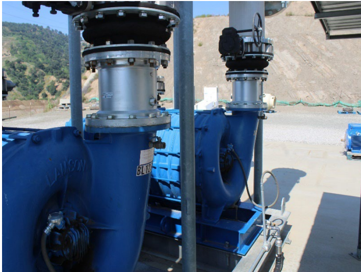
Photo 221: Flares 9, 10, 11 and Gas-to-Energy Facility: April 9, 2026
