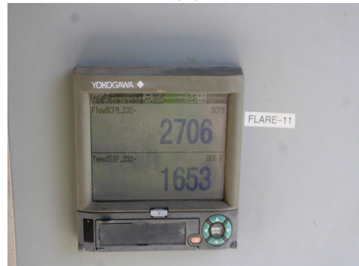
Photo 232: Flares 9, 10, 11 and Gas-to-Energy Facility: May 21, 2026
