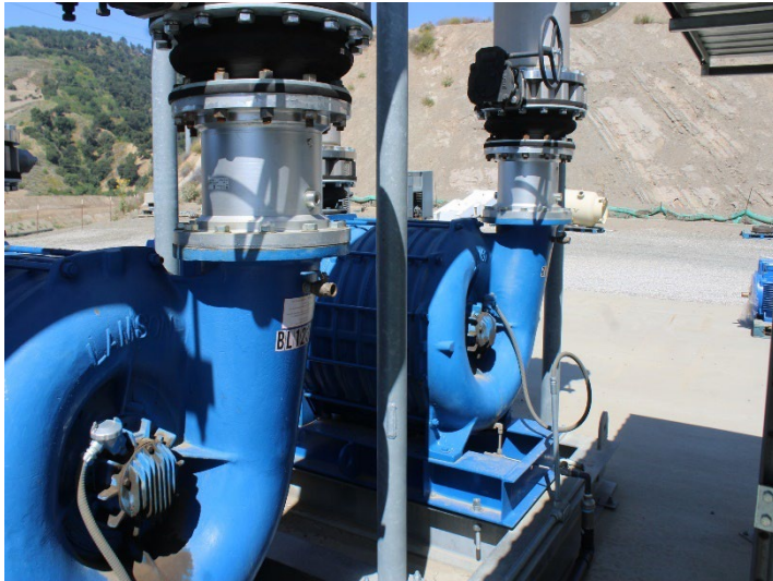
Photo 233: Flares 9, 10, 11 and Gas-to-Energy Facility: May 21, 2026
