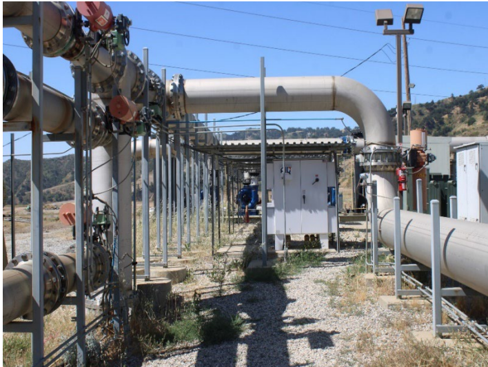
Photo 229: Flares 9, 10, 11 and Gas-to-Energy Facility: May 21, 2026
