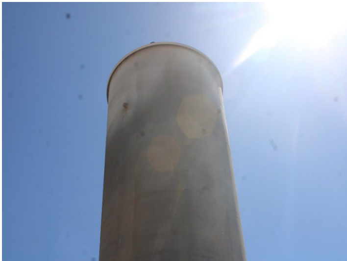
Photo 239: Flares 9, 10, 11 and Gas-to-Energy Facility: June 11, 2026
