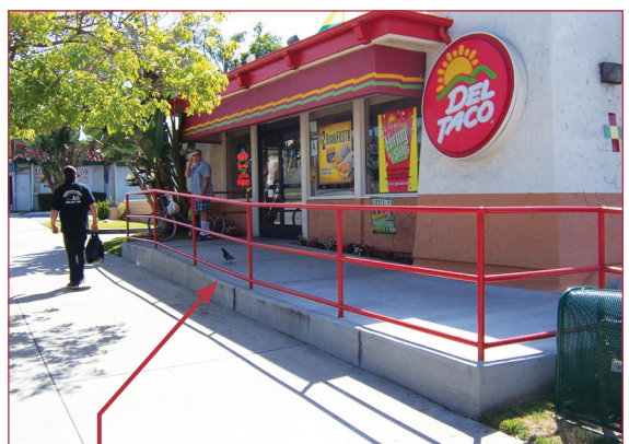
⚠ Entrance is obstructed by ramp and creates barrier from the sidewalk
