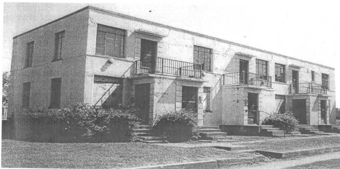
Figure 16 - A contemporary view of an individual building in Cedar Springs showing subsequent deterioration. (National Register of Historic Places Nomination, 1991)
