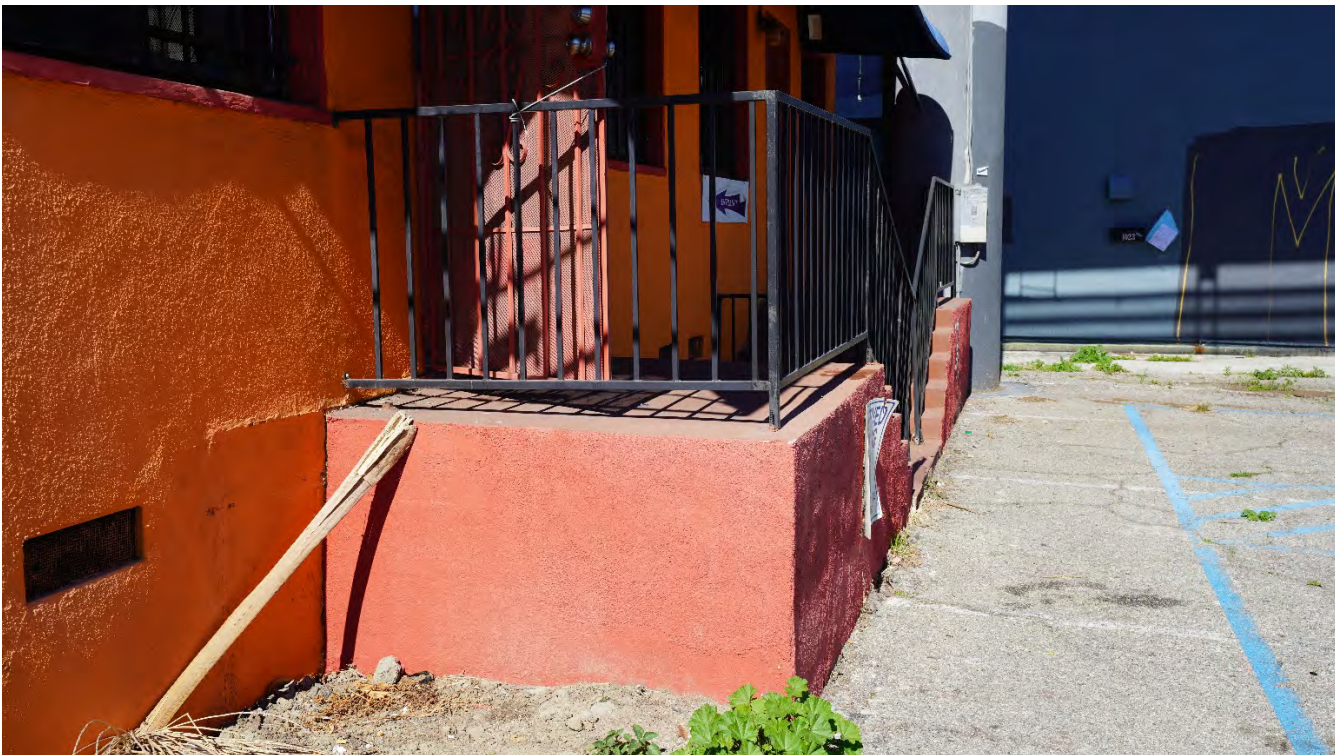
1025-1027 South Crenshaw Boulevard – Crenshaw Women’s Center Detail of porch on main east elevation Photograph taken: February 18, 2021
