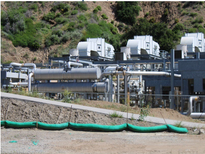
Photo 99: Flares 9, 10, 11 and Gas-to-Energy Facility: April 16, 2024
