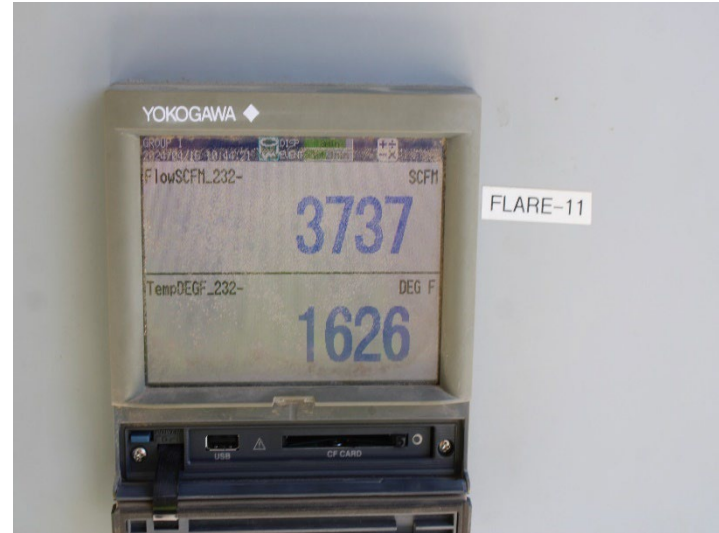
Photo 94: Flares 9, 10, 11 and Gas-to-Energy Facility: April 16, 2024
