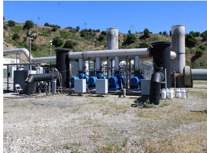
Photo 98: Flares 9, 10, 11 and Gas-to-Energy Facility: April 16, 2024
