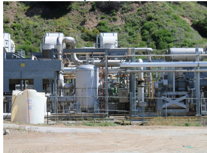
Photo 100: Flares 9, 10, 11 and Gas-to-Energy Facility: April 16, 2024
