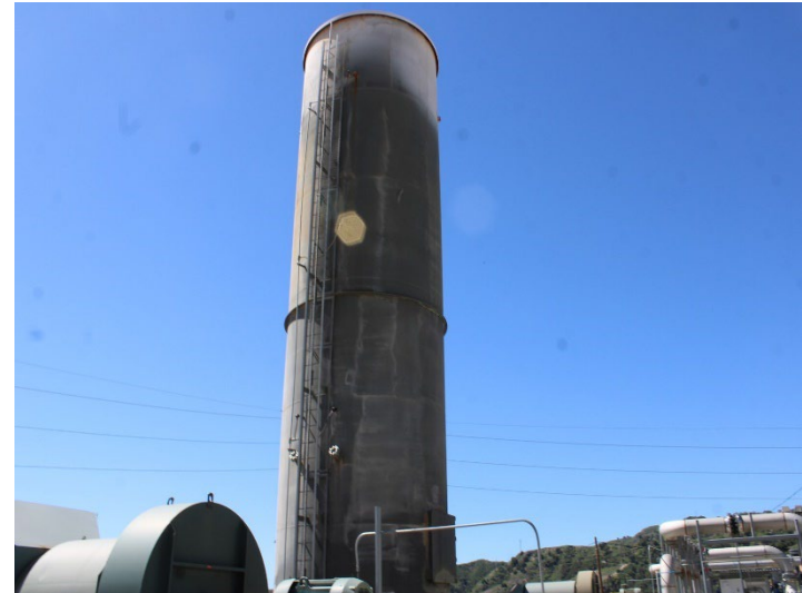
Photo 90: Flares 9, 10, 11 and Gas-to-Energy Facility: April 16, 2024
