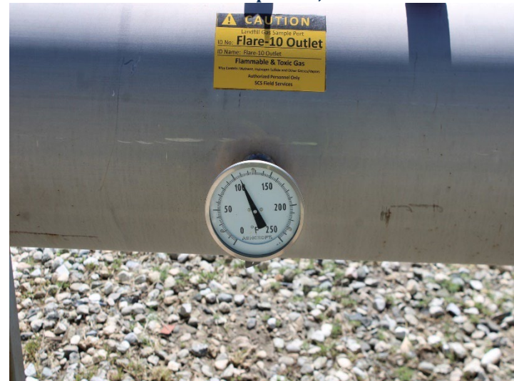
Photo 88: Flares 9, 10, 11 and Gas-to-Energy Facility: April 16, 2024
