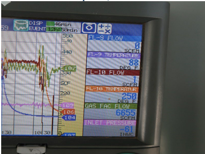
Photo 103: Flares 9, 10, 11 and Gas-to-Energy Facility: May 21, 2024
