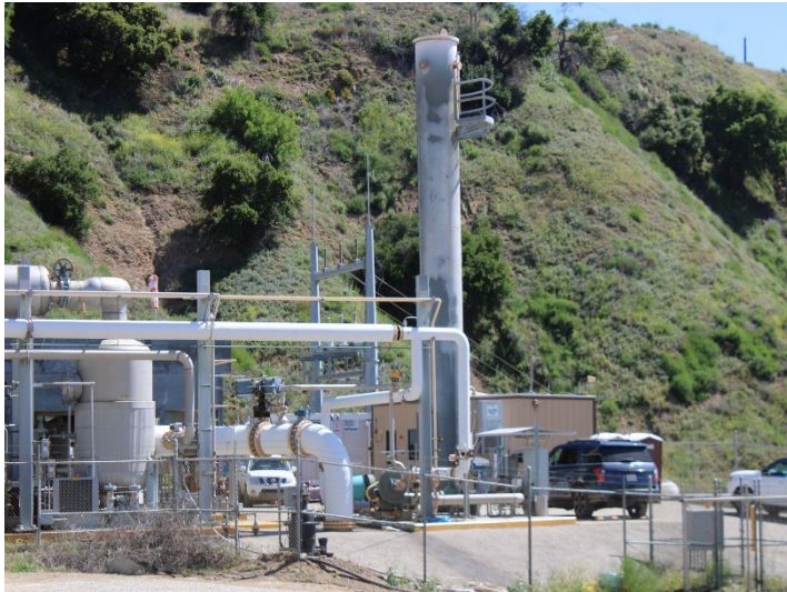
Photo 101: Flares 9, 10, 11 and Gas-to-Energy Facility: April 16, 2024
