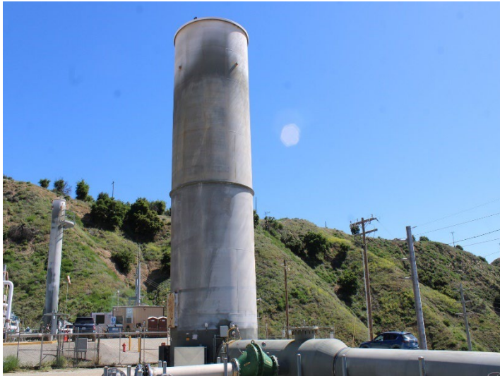
Photo 89: Flares 9, 10, 11 and Gas-to-Energy Facility: April 16, 2024
