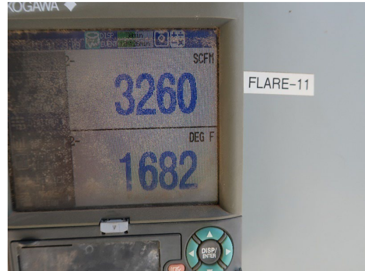
Photo 106: Flares 9, 10, 11 and Gas-to-Energy Facility: June 11, 2024
