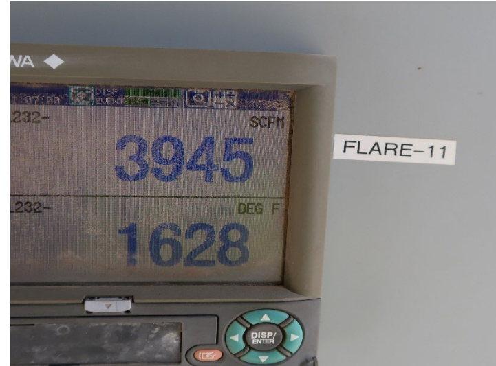
Photo 102: Flares 9, 10, 11 and Gas-to-Energy Facility: May 21, 2024
