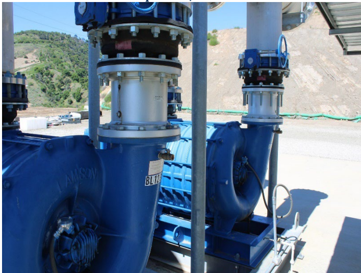
Photo 95: Flares 9, 10, 11 and Gas-to-Energy Facility: April 16, 2024
