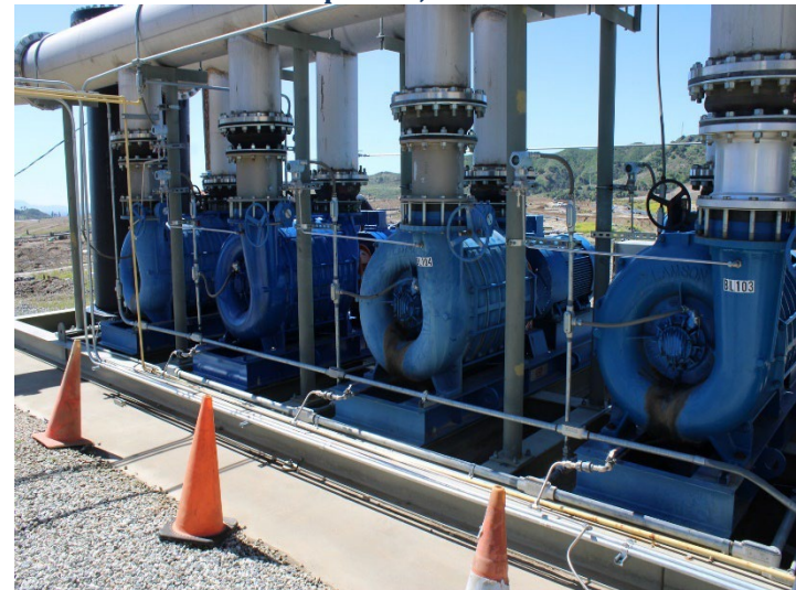
Photo 92: Flares 9, 10, 11 and Gas-to-Energy Facility: April 16, 2024
