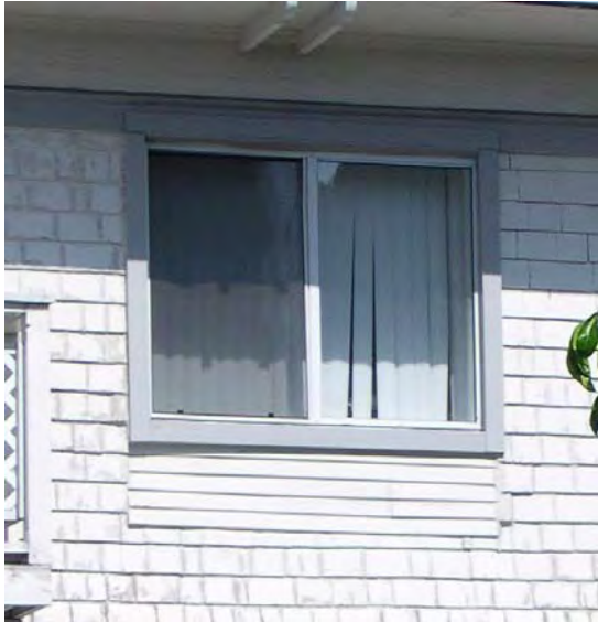
This window has been inappropriately filled in. New windows are often not the same size as historic windows, so fitting them into historic window openings is difficult.
