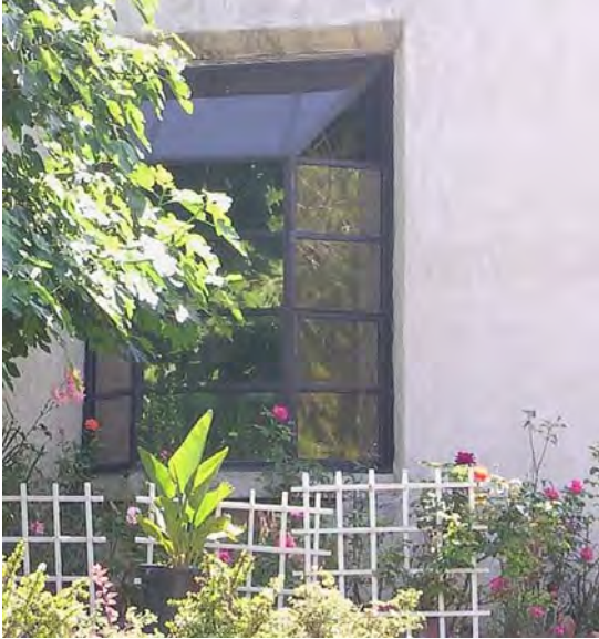
Replacing original windows with greenhouse style windows is inappropriate
