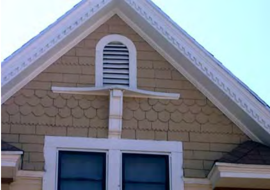
This home has specialty "fishscale" shingles. When repairing these shingles, it is important to "piece in" materials that match the original.
