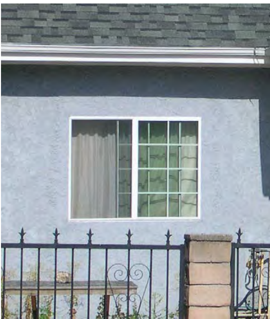
These windows are inappropriate, because they have "stick-on" muntins, instead of true divided light windows, in which small panes of glass are separated by the muntin framework.
