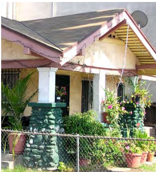
The character of the porch columns has been destroyed by inappropriate paint.
