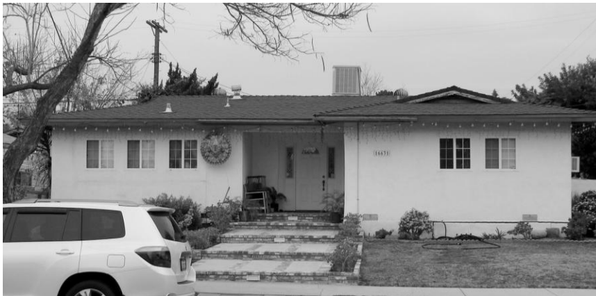
The smaller replacement windows on the façade of this house, with no trim or sills, severely diminish the house's integrity of design, materials, and feeling. This house would be a non-contributor to an historic district.
