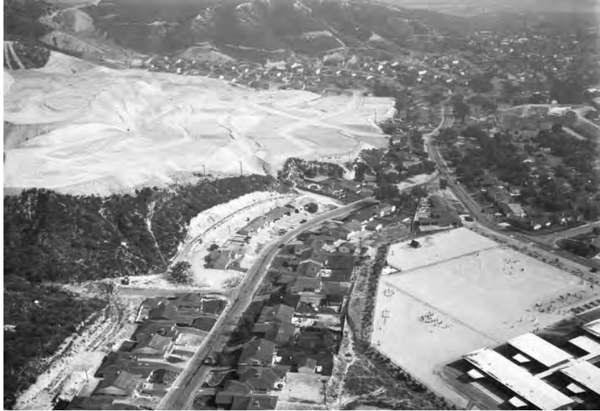
Land cleared and graded for the construction of tract houses, Los Angeles County, 1955. (Howard D. Kelly, photographer. Courtesy of the Los Angeles Public Library.)
