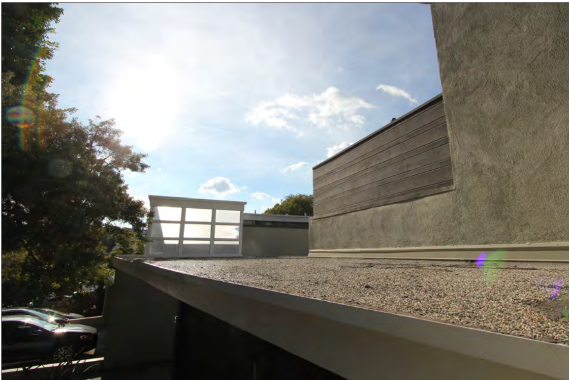
Image 34: Subject property, upper building, east elevation (primary facade), detail of roof, view southwest (Chattel, 2020)
