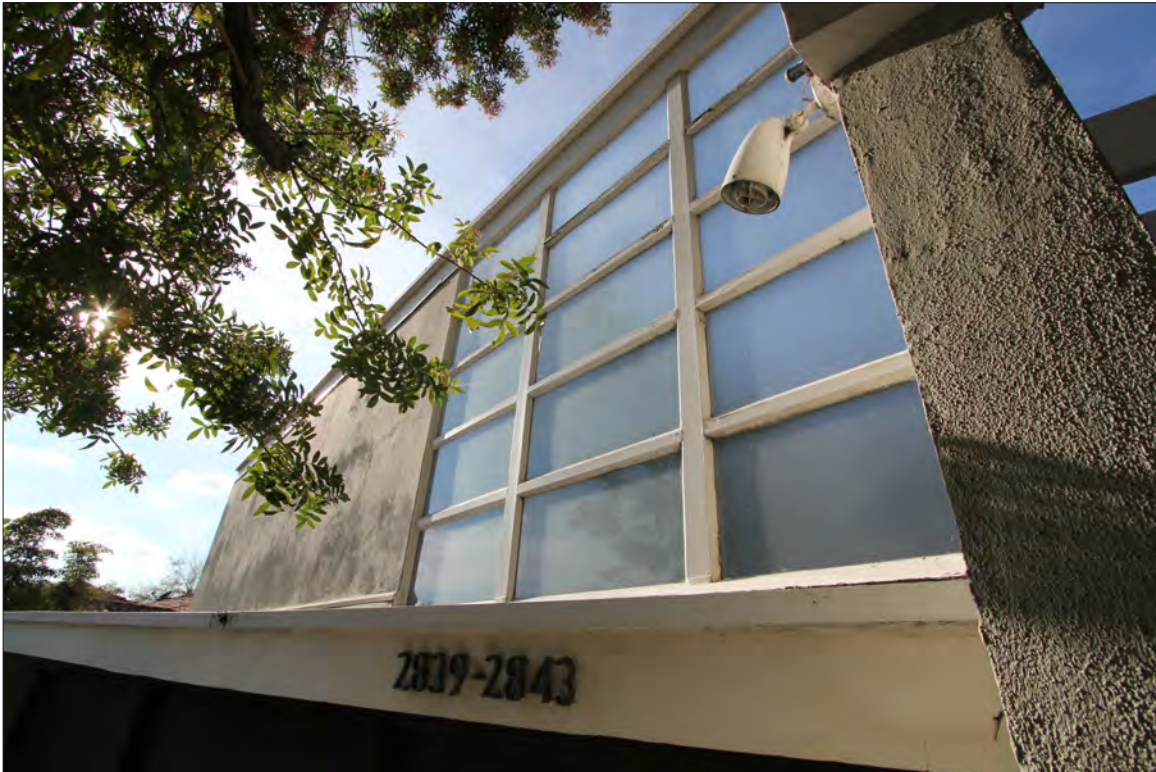
Image 9: Subject property, lower building, east elevation (primary facade), detail of corner window, view west (Chattel, 2020)
