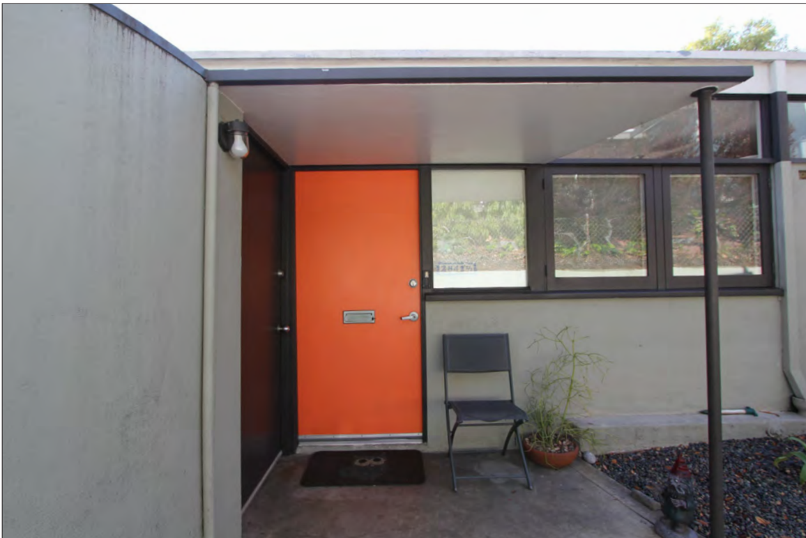
Image 18: Subject property, lower building, north elevation, typical unit entryway, view southwest (Chattel, 2020)
