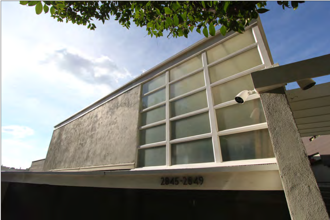
Image 33: Subject property, upper building, east elevation (primary facade), detail of corner window, view west (Chattel, 2020)
