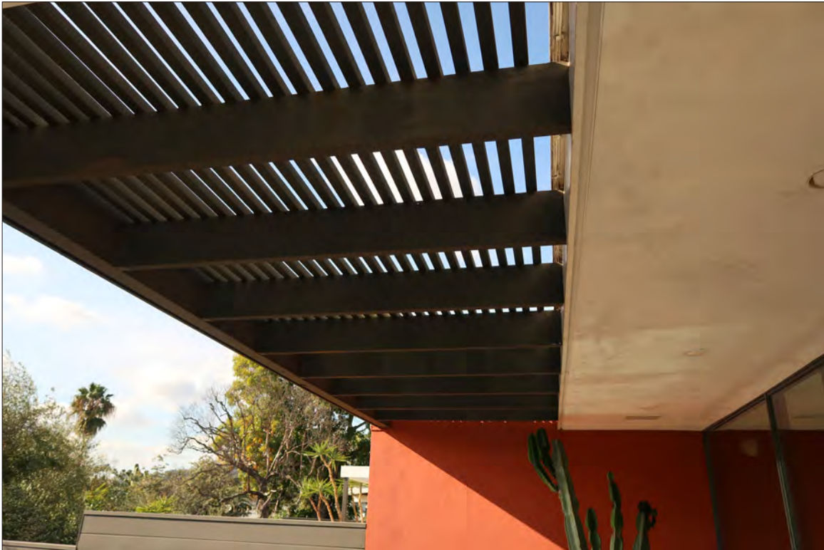
Image 25: Subject property, lower building, detail of non-original backyard patio roof, view northwest (Chattel, 2020)
