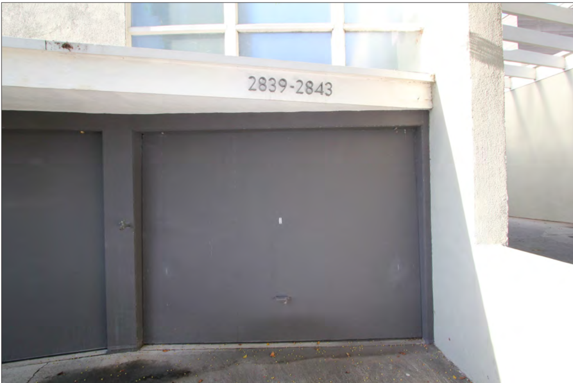
Image 10: Subject property, lower building, east elevation (primary facade), detail of non-original garage door, view northwest (Chattel, 2020)
