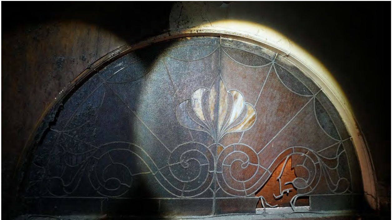
King Edward Hotel Stained glass transom above elevator, behind plywood Photo taken: March 29, 2019
