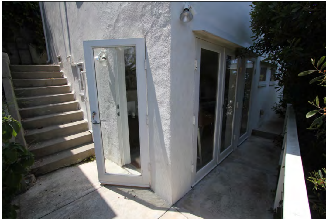
Photo 19: 145 Adelaide Drive, north and east elevations of residence, view southwest. Note the outside access to altered bedroom and bathroom at the tall basement crawlspace (Chattel, 2018)
