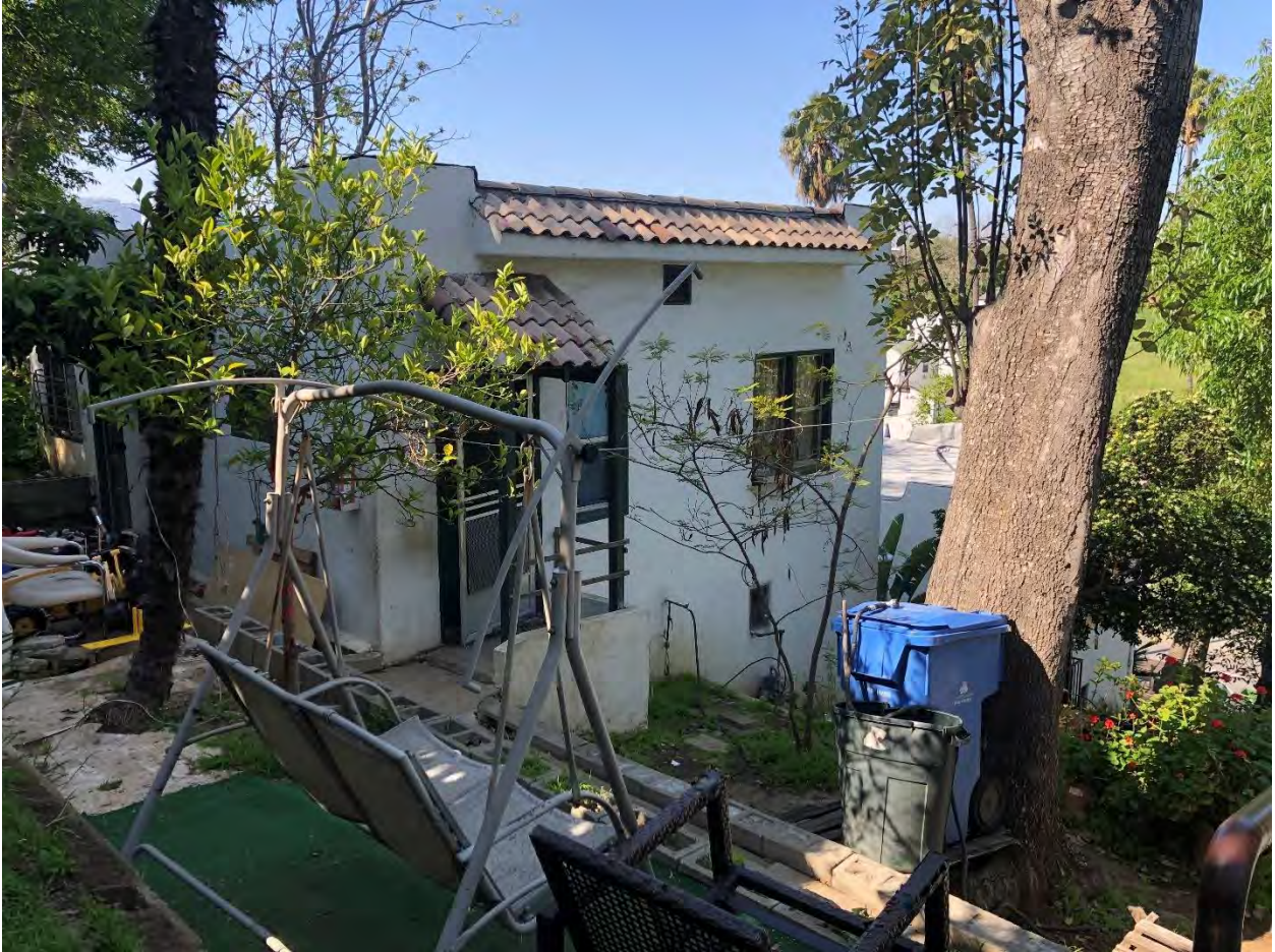
4. 1251–1259 Sunset Boulevard, Individual Bungalow with Altered Courtyard Cinderblock Retaining Walls and Altered Porch; view southwest, April 1, 2020
