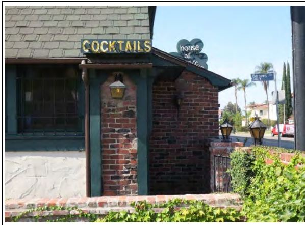
Detail of textured stucco and clinker brick wall cladding on north façade (ARG, 2018)
