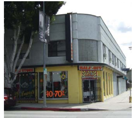
A rough textured stucco has been inappropriately applied to this building.
