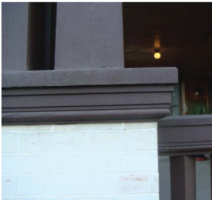
A detail showing where balustr, balustrade and column converge on a Craftsman porch is shown..
