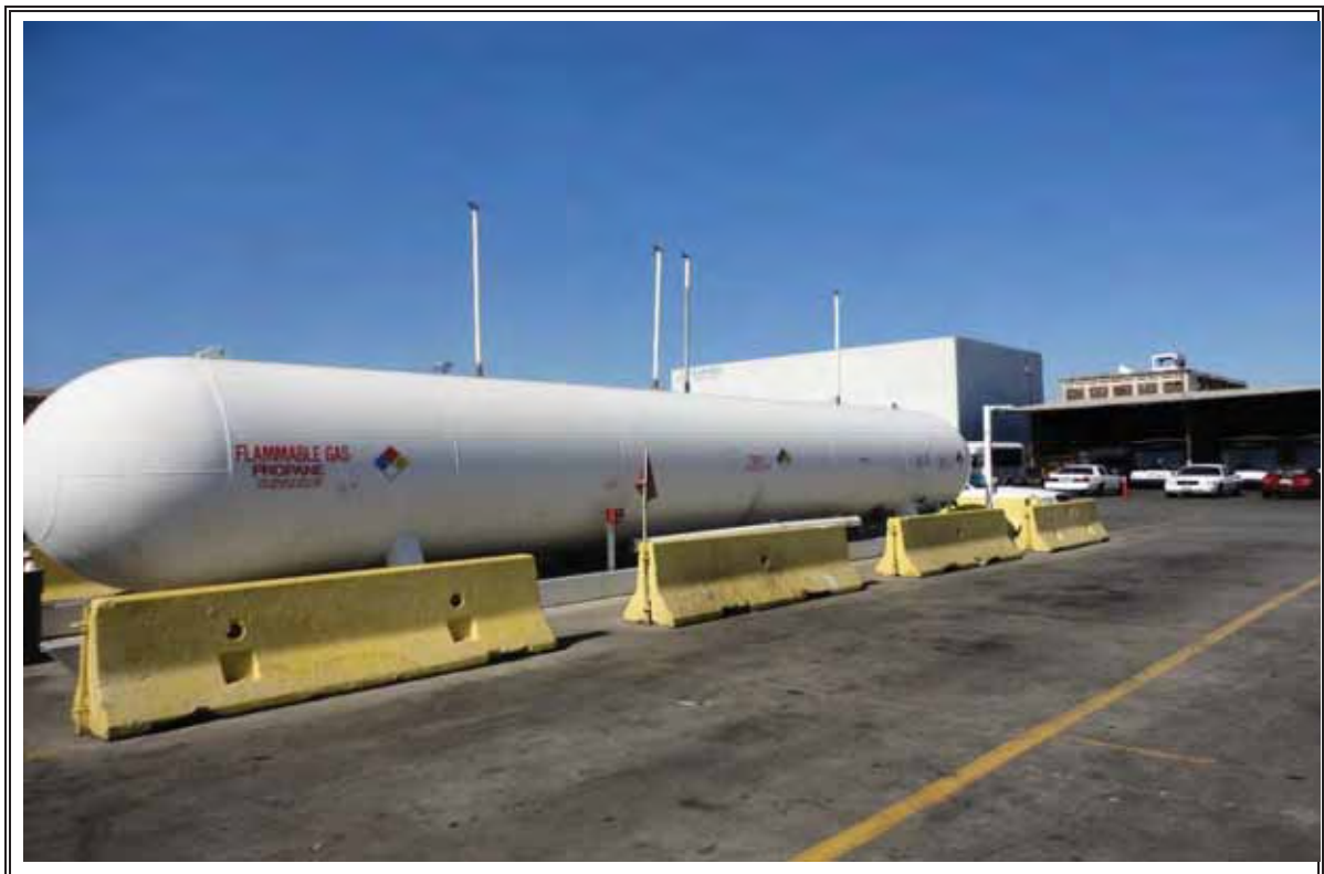
Photograph Number 8: View of propane tank observed in the middle of parking lot.
