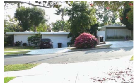
The aesthetic of the Mar Vista Tract flat roofs is sensitive to installation of mechanical apparatus.
