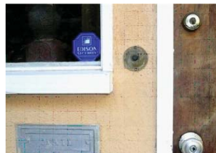
Original entrance door hardware: Lock, doorknob, door bell, and pot metal mail box.
