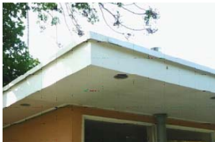
A 1"x1" flashing spacing shim protects the wood fascia from rain water. Eave rafters were covered on the East side of Moore Street and on Meier Street.
