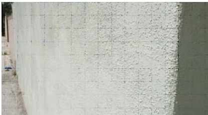
Additions should use similar finish materials as the original structure. Above an example of the original stucco.
