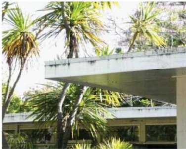
Omission of the flashing shim may cause deterioration of the fascia and water damage
