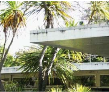
The original eaves design includes a combination of eaves of different depth where the longest eave is 4 ft deep.
