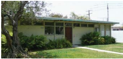
Front window configuration of house parallel to street: Full row of clerestory windows, two 1/2 height kitchen windows and three 3/4 bedroom windows.
