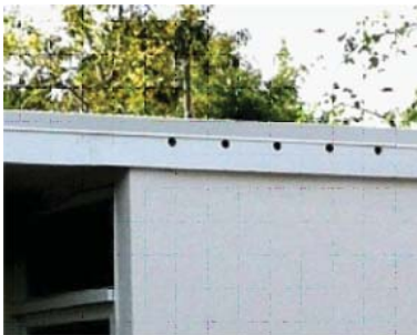
Rear roof vents. Omission of a 1"x1" flashing spacing shim may cause water to enter the house through these vents
