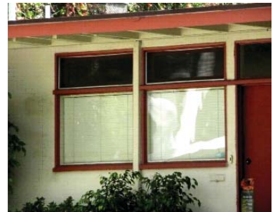
One of two original front side gutter downspouts comes down between the two kitchen windows.
