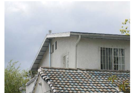
Inappropriate materials can compromise the historic character of a structure. In this case the combination of asphalt shingles with synthetic clay tiles both detract from the appearance of this structure.
