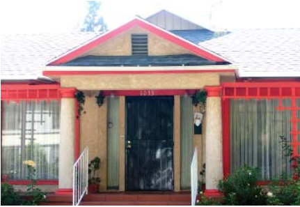
This doorway has been altered with a metal gate and plate glass sidelights.
