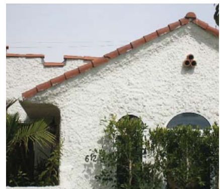
Heavily textured stucco is a modern look and detracts from the appearance of this structure.
