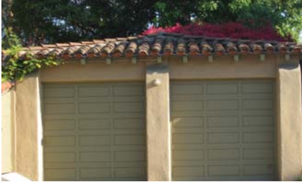
Most often wood doors that replicate the look of old carriage-style garage doors are appropriate.
