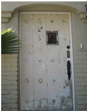
This door with its original hardware and decorative features should be repaired and refinished before replacement is considered.
