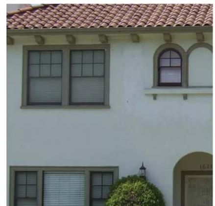
Flush, frameless, and oddly arranged windows may be inappropriate on a new house.
