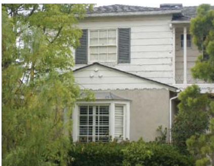
The mix of stucco and wood siding is appropriate for this structure.
