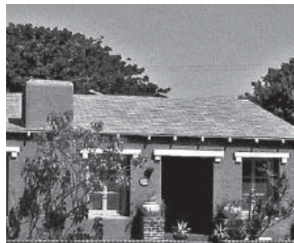
Clay tile would be the historically appropriate roof material on a Spanish Colonial house such as this. Composition shingles are inappropriate.
