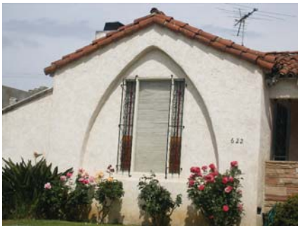
This window has been replaced with an ill-fitted window that diminishes the historic integrity of the house.
