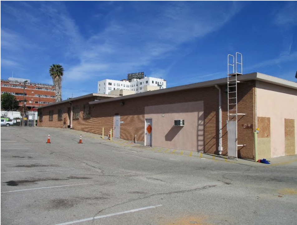
Figure 2. South and east elevation of the Plant Operating Center, looking northwest (IMG_2526)
