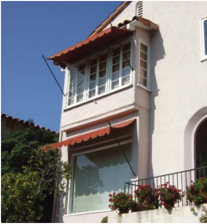
These canvas awnings are appropriately sized, simple in their configuration and are easily removed.
