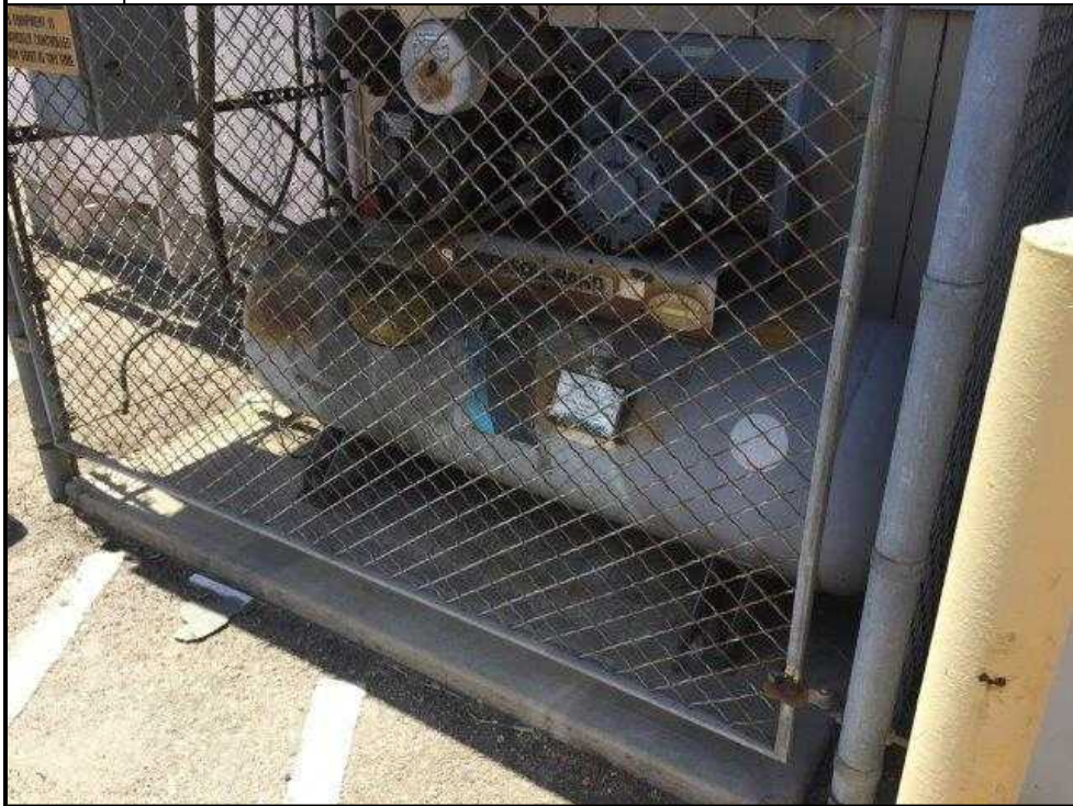
26. Air compressor adjacent to maintenance building.
