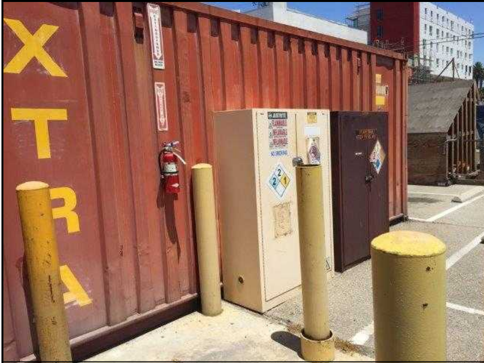
25. Miscellaneous flammable materials storage cabinets.
