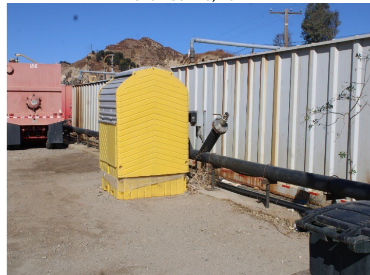
Photo 212: Alder Tank Liquids Treatment System: November 20, 2024
