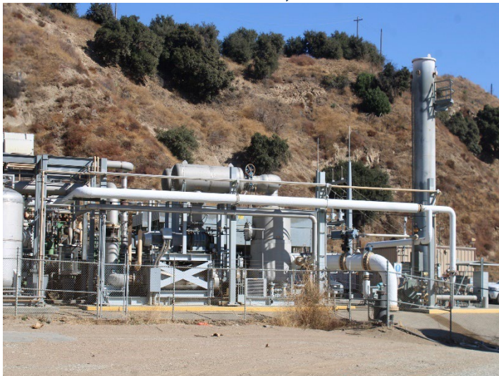
Photo 251: Flares 9, 10, 11 and Gas-to-Energy Facility: November 20, 2024
