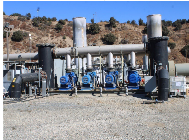
Photo 236: Flares 9, 10, 11 and Gas-to-Energy Facility: October 31, 2024
