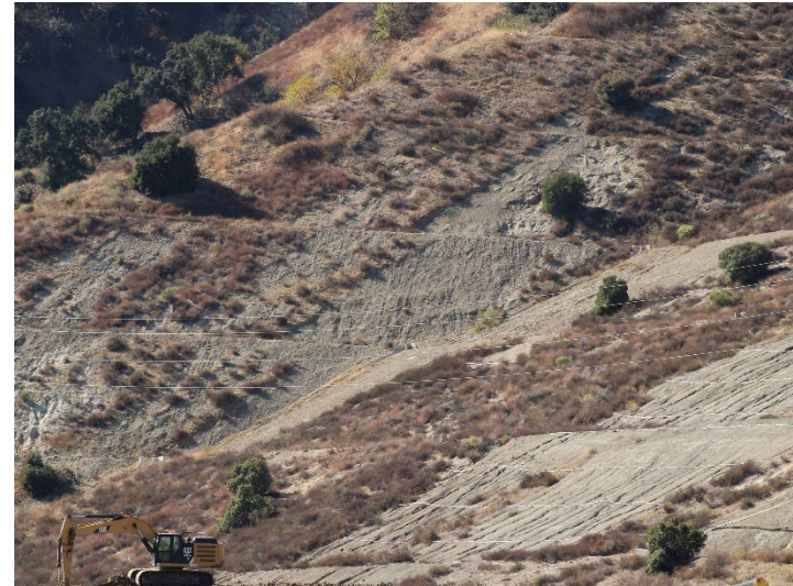
Photo 214: County Sage Mitigation Area and Westside Drainage Channels: November 20, 2024
