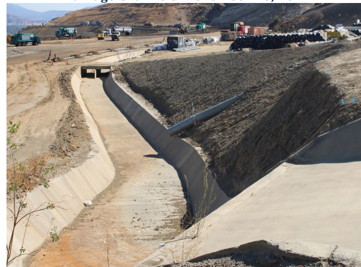
Photo 216: County Sage Mitigation Area and Westside Drainage Channels: November 20, 2024
