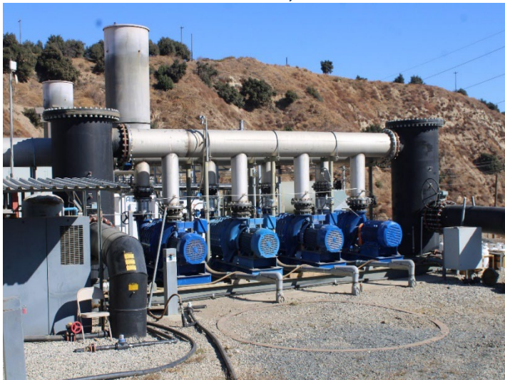
Photo 247: Flares 9, 10, 11 and Gas-to-Energy Facility: November 20, 2024
