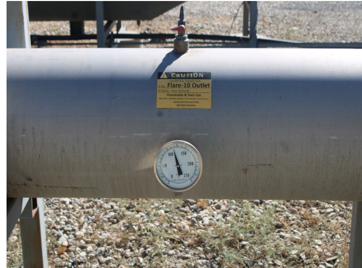
Photo 222: Flares 9, 10, 11 and Gas-to-Energy Facility: October 31, 2024
