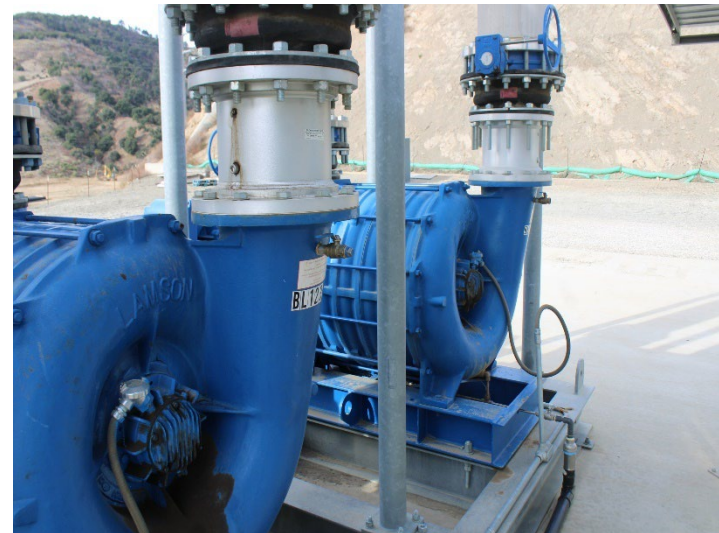
Photo 258: Flares 9, 10, 11 and Gas-to-Energy Facility: December 11, 2024
