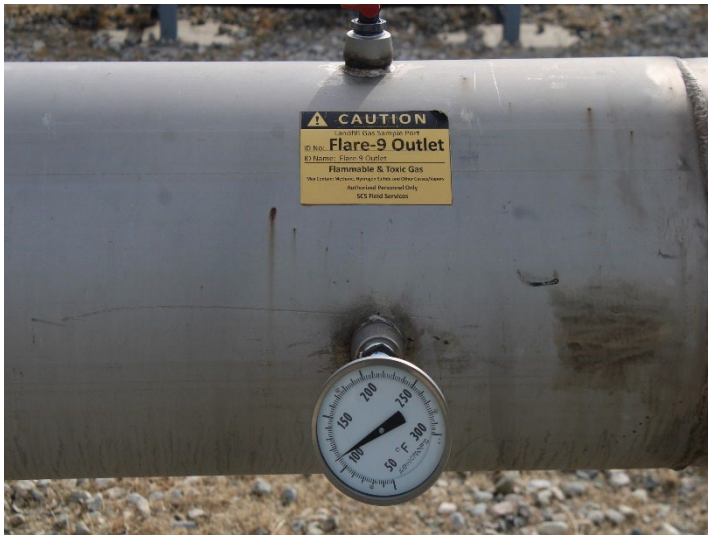
Photo 253: Flares 9, 10, 11 and Gas-to-Energy Facility: December 11, 2024
