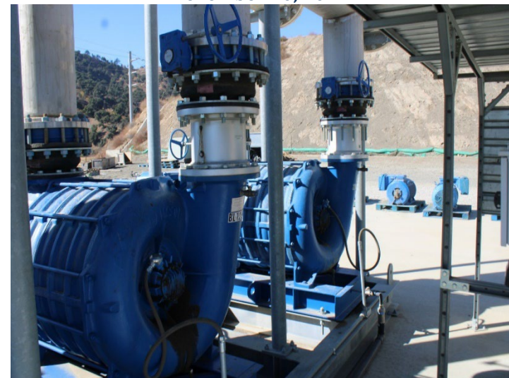
Photo 244: Flares 9, 10, 11 and Gas-to-Energy Facility: November 20, 2024
