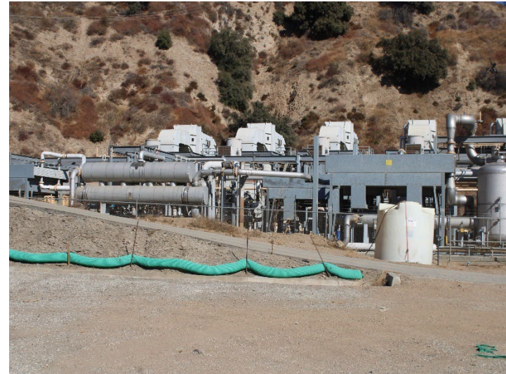
Photo 250: Flares 9, 10, 11 and Gas-to-Energy Facility: November 20, 2024
