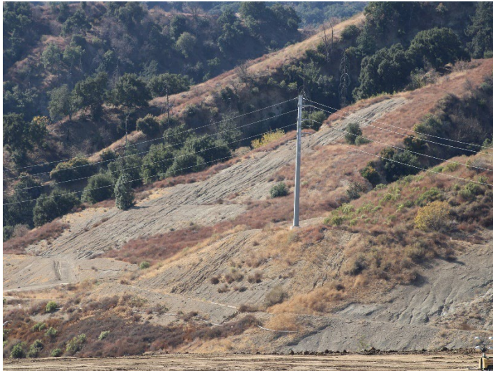
Photo 213: County Sage Mitigation Area and Westside Drainage Channels: November 20, 2024
