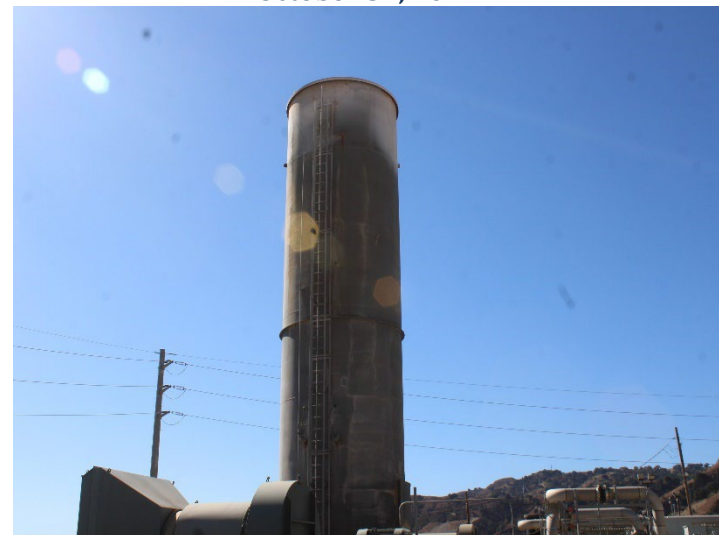
Photo 224: Flares 9, 10, 11 and Gas-to-Energy Facility: October 31, 2024
