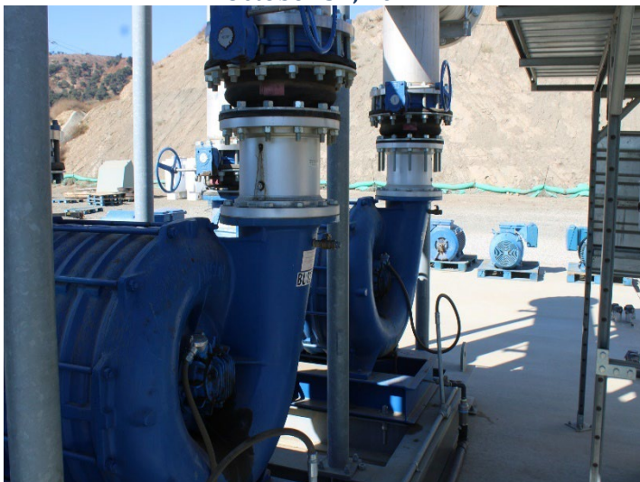
Photo 231: Flares 9, 10, 11 and Gas-to-Energy Facility: October 31, 2024
