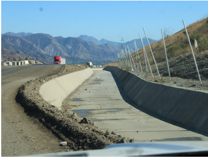
Photo 217: County Sage Mitigation Area and Westside Drainage Channels: November 20, 2024
