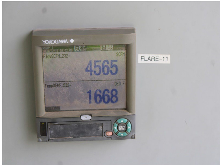
Photo 257: Flares 9, 10, 11 and Gas-to-Energy Facility: December 11, 2024
