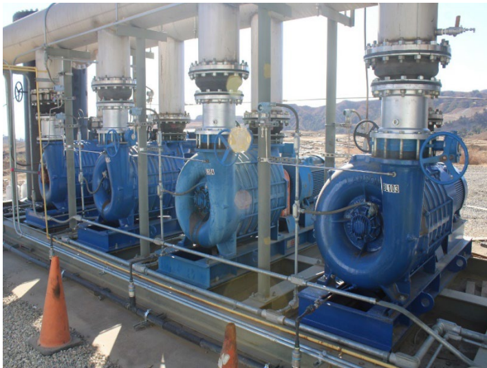
Photo 241: Flares 9, 10, 11 and Gas-to-Energy Facility: November 20, 2024
