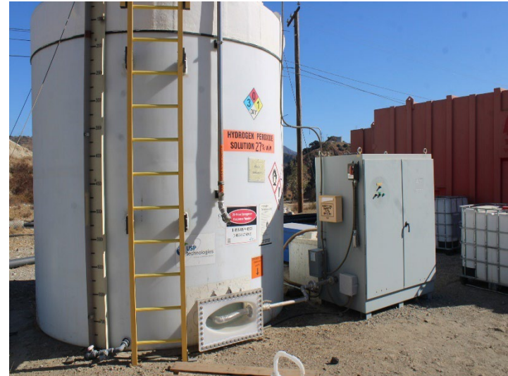
Photo 210: Alder Tank Liquids Treatment System: November 20, 2024
