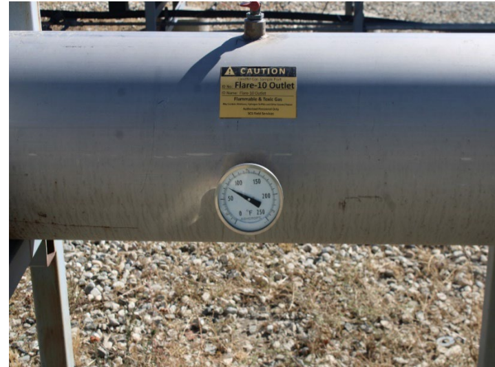
Photo 238: Flares 9, 10, 11 and Gas-to-Energy Facility: November 20, 2024
