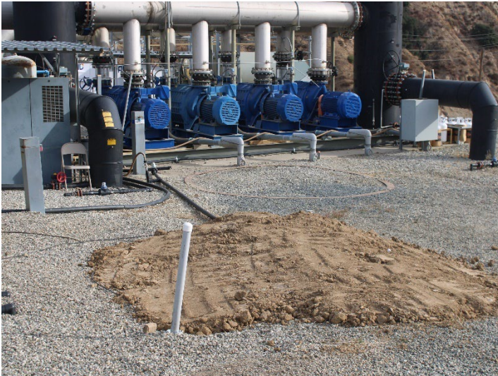
Photo 261: Flares 9, 10, 11 and Gas-to-Energy Facility: December 11, 2024
