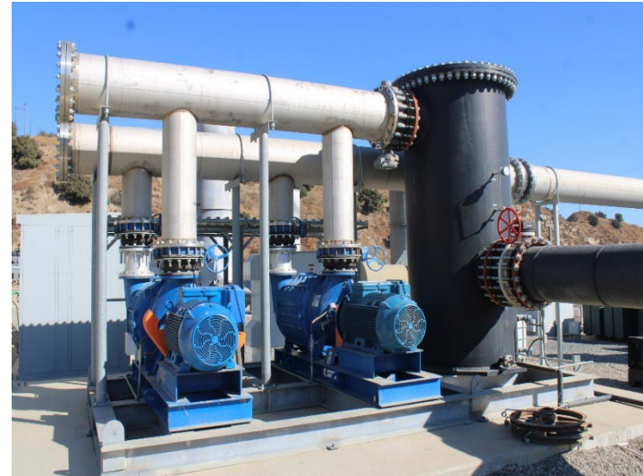
Photo 246: Flares 9, 10, 11 and Gas-to-Energy Facility: November 20, 2024
