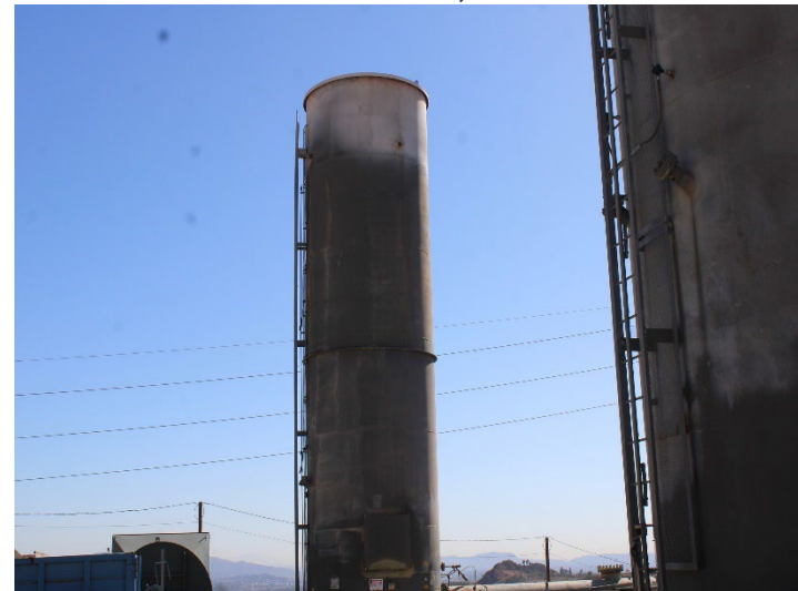
Photo 248: Flares 9, 10, 11 and Gas-to-Energy Facility: November 20, 2024
