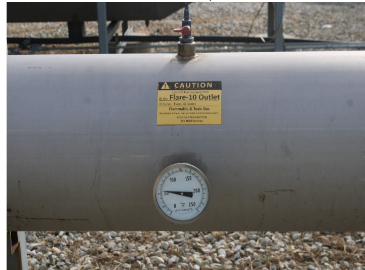
Photo 252: Flares 9, 10, 11 and Gas-to-Energy Facility: December 11, 2024
