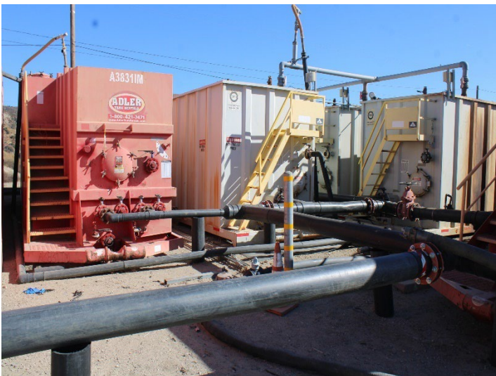
Photo 211: Alder Tank Liquids Treatment System: November 20, 2024
