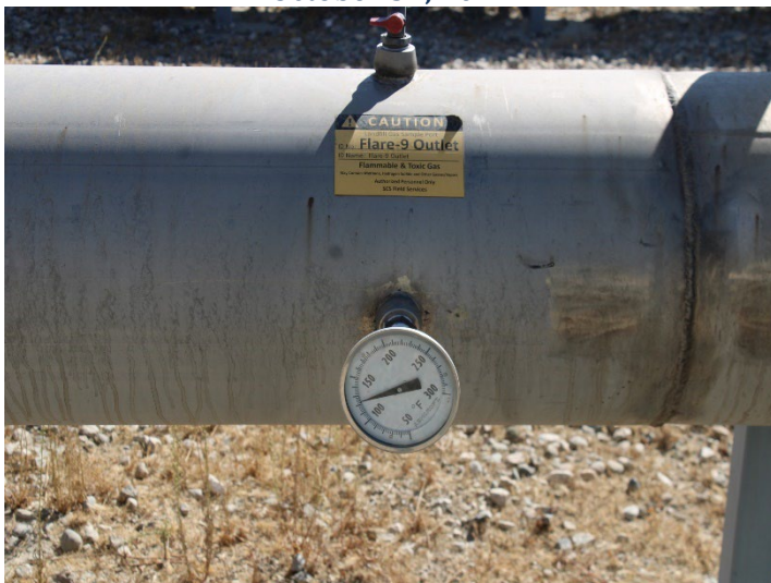
Photo 227: Flares 9, 10, 11 and Gas-to-Energy Facility: October 31, 2024
