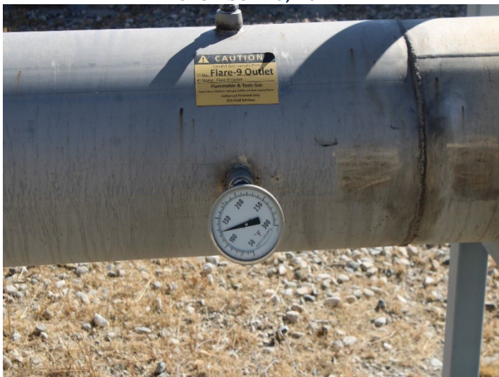
Photo 239: Flares 9, 10, 11 and Gas-to-Energy Facility: November 20, 2024
