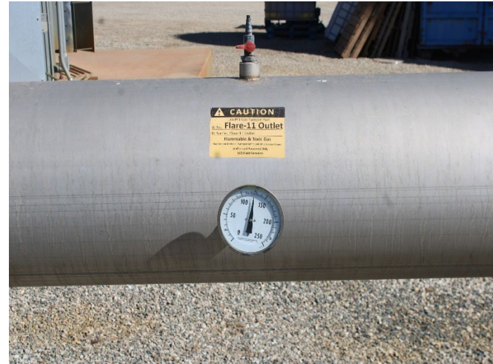
Photo 226: Flares 9, 10, 11 and Gas-to-Energy Facility: October 31, 2024
