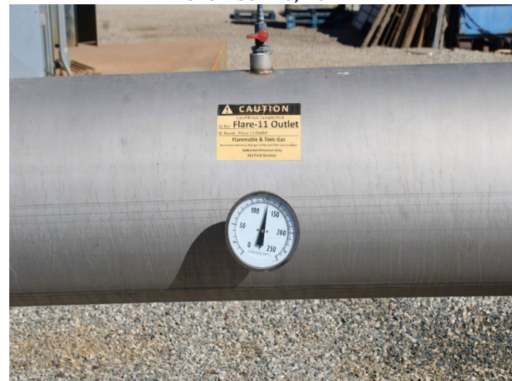
Photo 240: Flares 9, 10, 11 and Gas-to-Energy Facility: November 20, 2024
