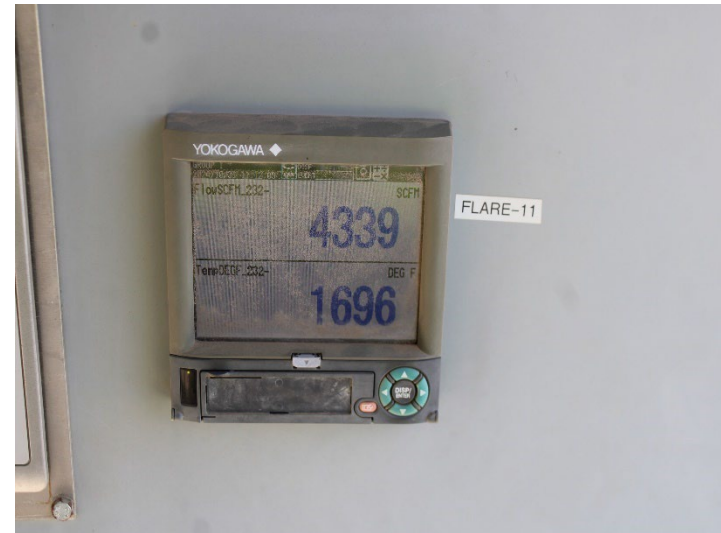
Photo 230: Flares 9, 10, 11 and Gas-to-Energy Facility: October 31, 2024
