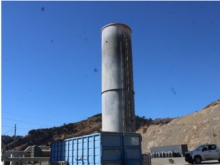
Photo 225: Flares 9, 10, 11 and Gas-to-Energy Facility: October 31, 2024
