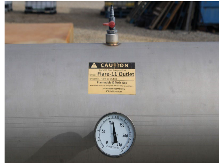
Photo 254: Flares 9, 10, 11 and Gas-to-Energy Facility: December 11, 2024
