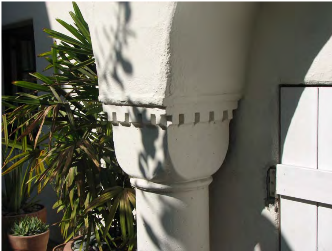
Fred C. Thomson Building, pillar capital, 6526-40 Sunset Boulevard, October 24, 2018, (Charles J. Fisher photo)
