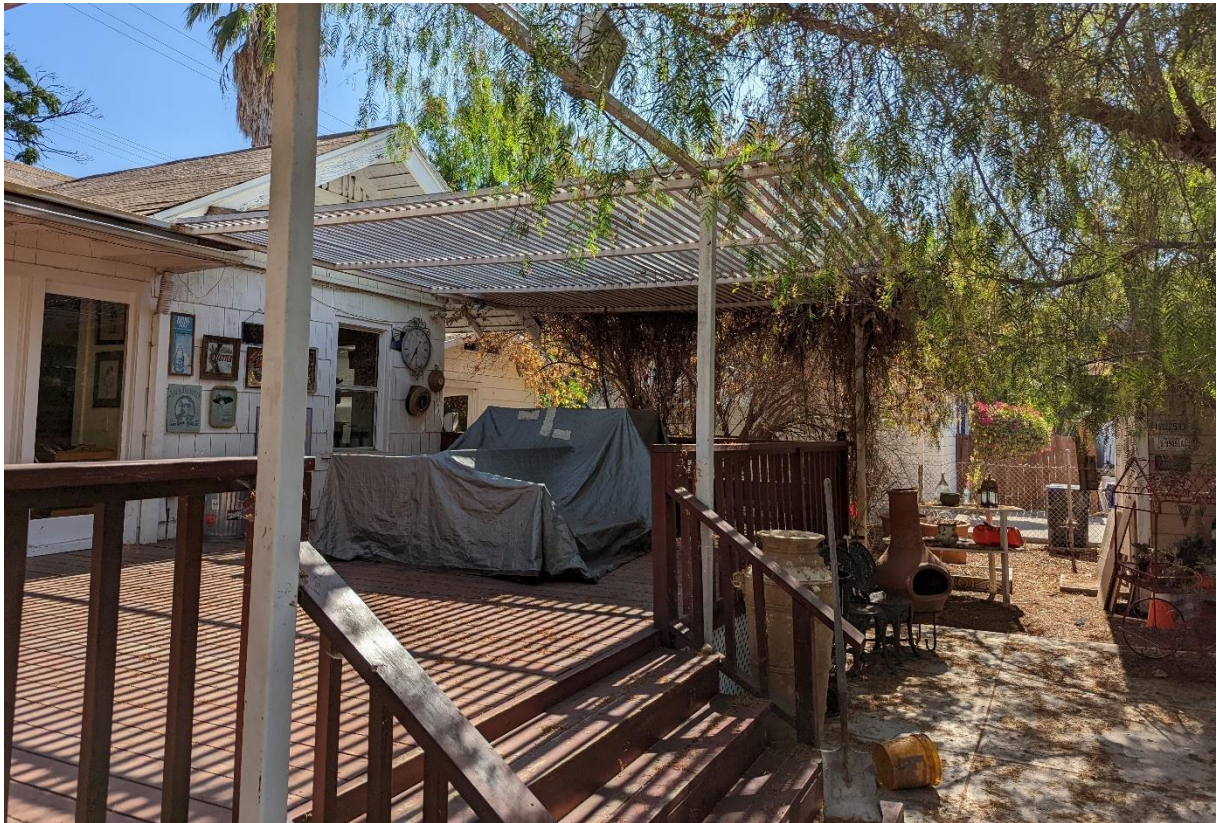
Photograph 13 Rear (South) Elevation of the Subject Building with Existing Sheds in Background
