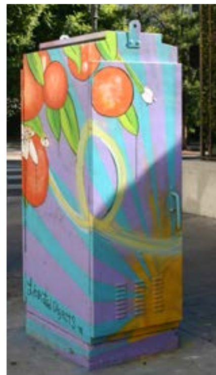
Utility boxes provide abundant opportunities to enliven the street environment.
