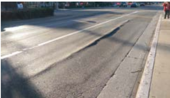
Where no bus pad exists, the weight of heavy vehicles causes rippling and cracking of the asphalt surface.
