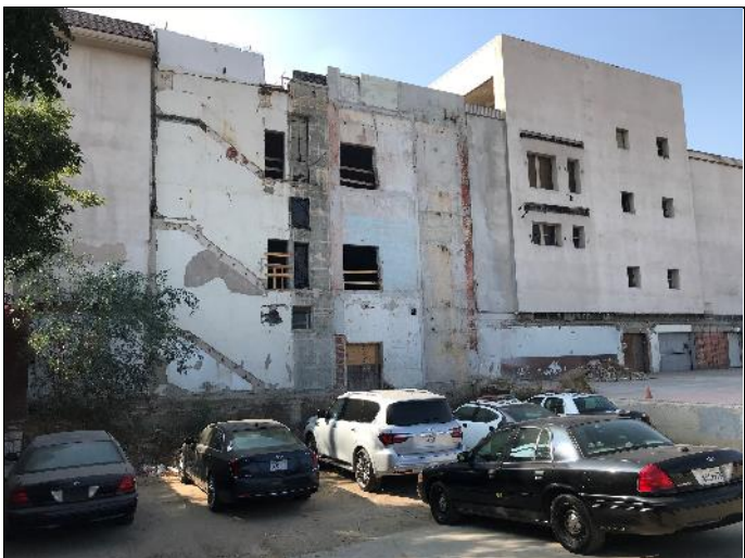
3. View of the former loading area and the rear (northern) side of the building
