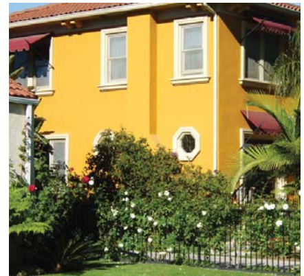
Foam plant-ons and pre-cast concrete are materials that would not have been originally used on this historic house.
