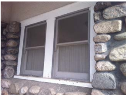
Original windows in Stonehurst are comprised of wood sashes and frames and are deeply set within stone masonry walls. Casement style windows are shown above, double-hung windows are shown below.
