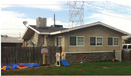
The porch at top is enclosed with screens and windows that fit within the full height of the porch opening. This “sleeping porch” style enclosure is historically appropriate. The porch at bottom has been fully enclosed and no longer reads as a porch. Enclosures such as these are inappropriate on an historic house.
