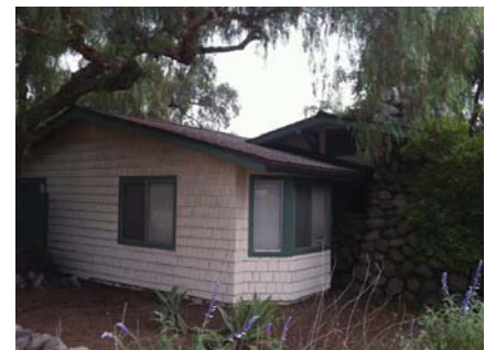
The addition shown at the foreground is compatible by virtue of its roof pitch and its use of shingled siding, a material that would have also been used during the Period of Significance.
