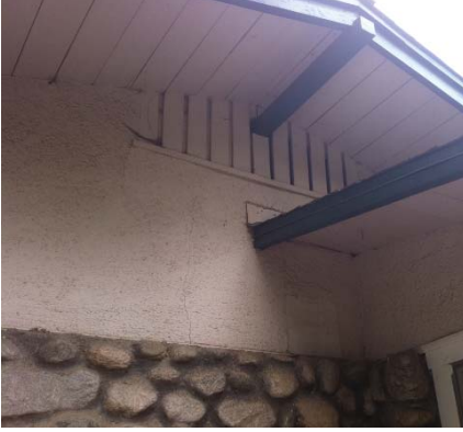
Clay tile is an inappropriate material for this Craftsman style home.
