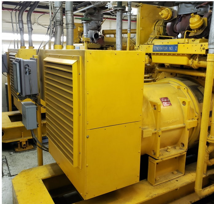
Photo 9—Emergency backup generators in northern building at the Site.
