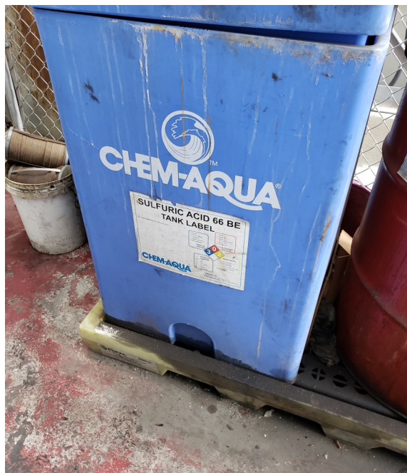
Photo 14—Container of sulfuric acid container for water treatment in the northern site building.
