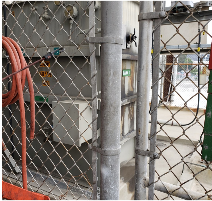
Photo 15—Southern California Edison electrical transform near southeast corner of the northern site building.
