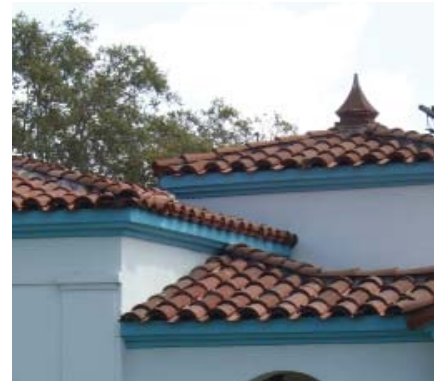
When planning a re-roof attention should be paid to how tiles are stacked, how ridges are adorned and to any other decorative features that exist.
