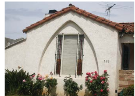
This window has been replaced with an ill-fitted window that diminishes the historic integrity of the house.
