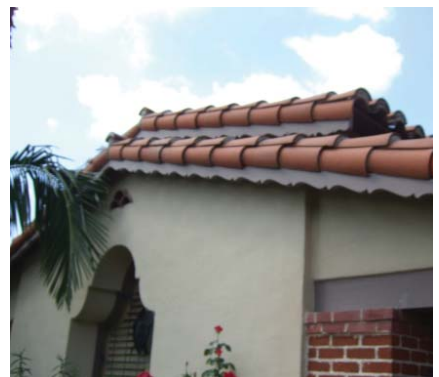
These decorative fascia or vergeboards are an equally significant part of this historic roof.
