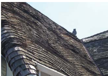
Wood shingles such as these should be carefully maintained, and replaced in small increments if needed.
