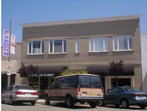
The historic casement windows on the second floor of this commercial building add to its historic character.
