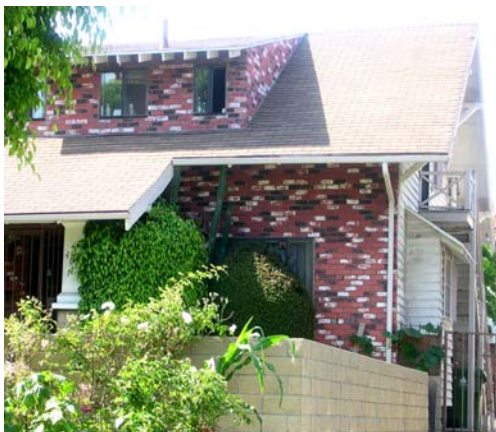
It is inappropriate to cover wood siding or other details with vinyl, stucco, or other materials. It is inappropriate to repair wood siding by adding new material that does not match the original.
