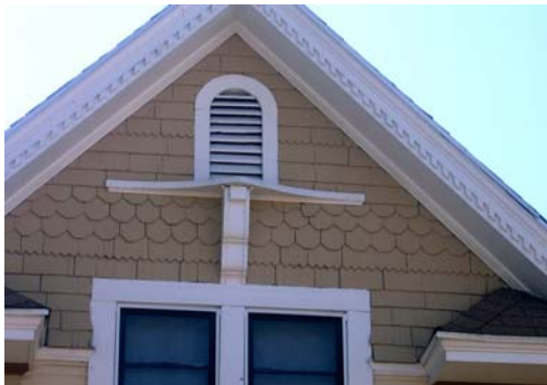
This home has speciality "fishscale" shingles. When repairing these shingles, it is important to "piece in" materials that match the original.
