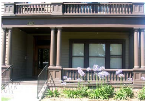
Adding a simple railing to improve safety is appropriate. However, the railing should match the existing porch in material and color.
