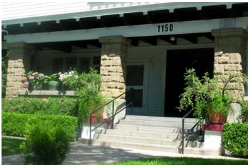
River rock is an important material used in Craftsman style homes and should be preserved. It is inappropriate to paint the river rock.
