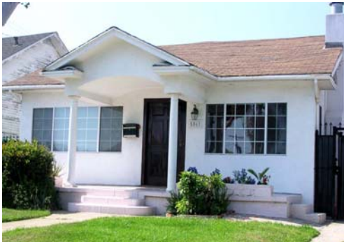
These replacement windows are inappropriate. When putting new windows on the front facade of a home, the new windows should match the historic windows in size, shape, arrangement of panes, materials, hardware, method of construction, and profile.
