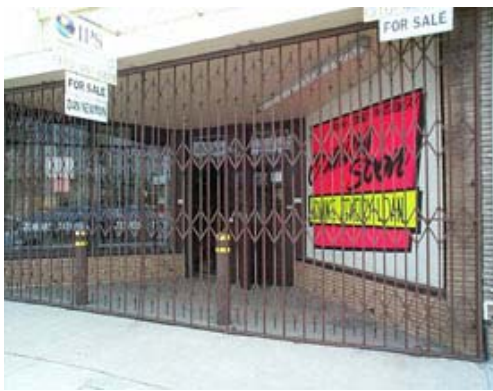
Security bars can be appropriate, but they should not completely conceal the store entrance and windows like the bars above.
