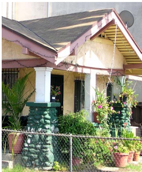
The character of the porch columns has been destroyed by inappropriate paint.
