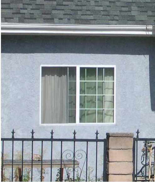
These windows are inappropriate, because they have “stick-on” muntins, instead of true divided light windows, in which small panes of glass are separated by the muntin framework.
