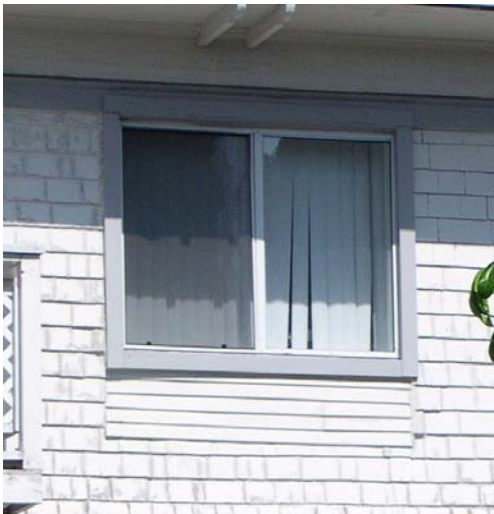
This window has been inappropriately filled in. New windows are often not the same size as historic windows, so fitting them into historic window openings is difficult.
