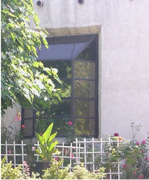
Replacing original windows with greenhouse style windows is inappropriate
