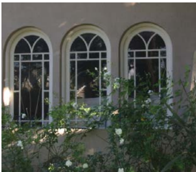
The decorative muntins in these arched windows would be difficult to replace. Repair of existing materials is always preferred.
