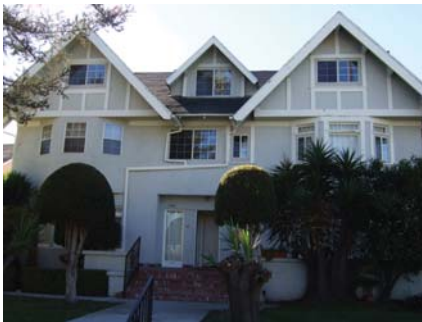
The modern windows that have been added to this home are poorly scaled and dramatically alter the home's original appearance.
