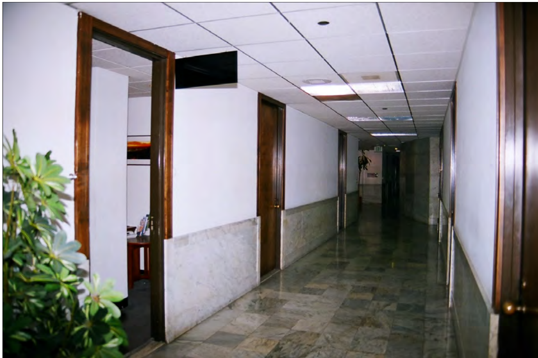
Photo 44: Fourth floor corridor, view east, note original marble wainscot and floor and original wood doors (Chattel, 2011)
