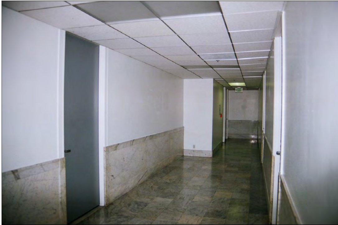
Photo 43: Third floor corridor, view east, note original marble wainscot and floor and contemporary wall enclosing stairwell (left near end of hall) (Chattel, 2011)
