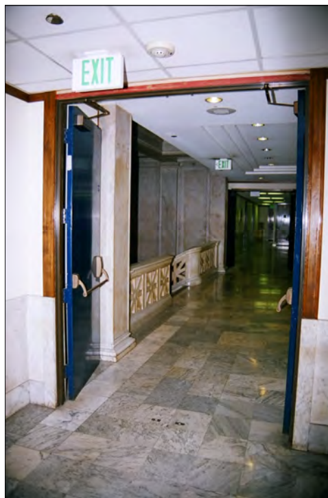
Photo 33: Second floor corridor, view west, note original marble wainscot, floor, and banisters (Chattel, 2011)
