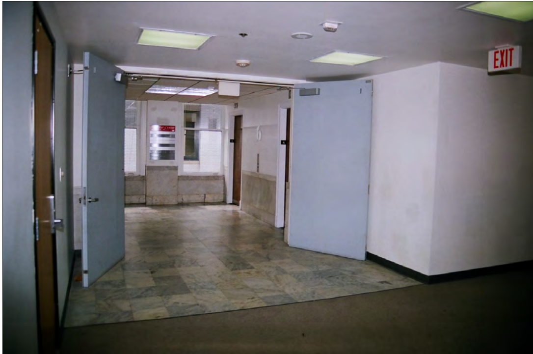
Photo 50: Sixth floor elevator corridor, view north, note original marble wainscot and floor (Chattel, 2011)
