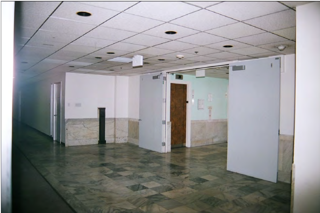
Photo 65: Eighth floor corridor, view northwest, note original marble floor and wainscot (Chattel, 2011)
