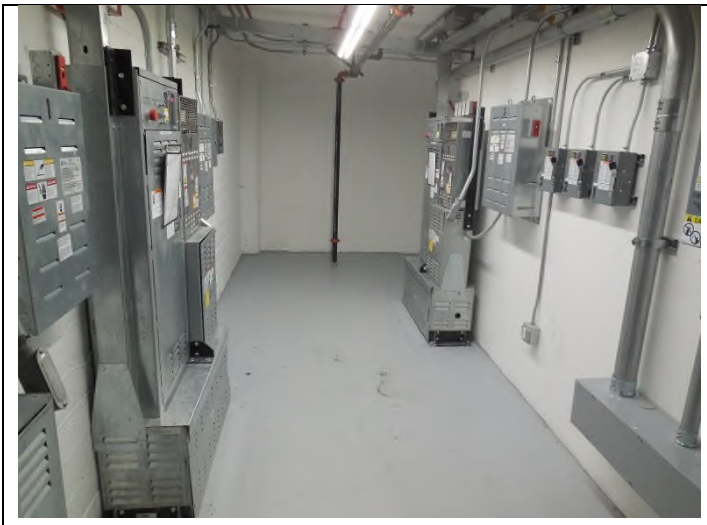
9. View of elevator equipment
