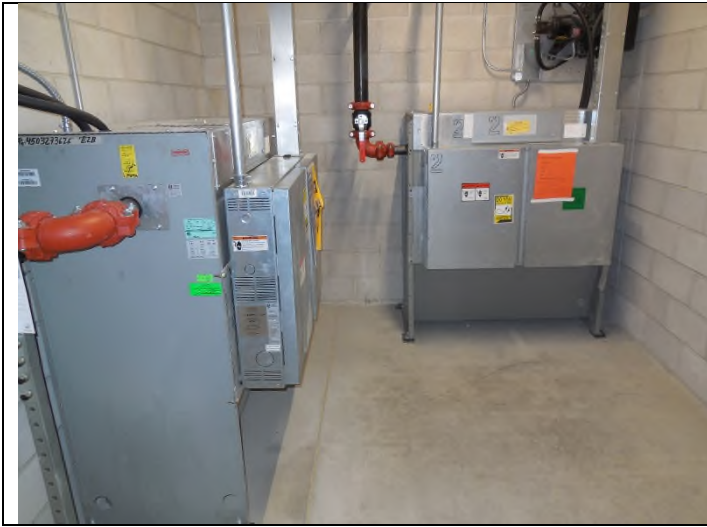
21. View of hydraulic elevators
