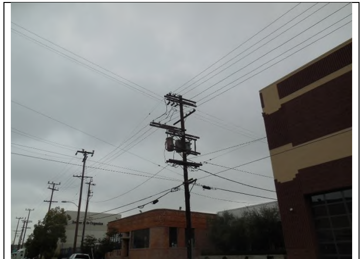
24. View of pole-mounted transformers
