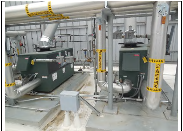
10. View of boilers
