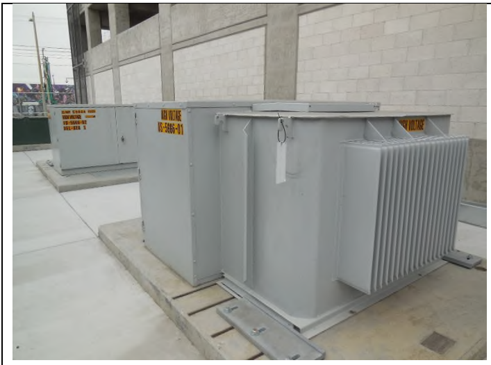
23. View of pad-mounted transformers
