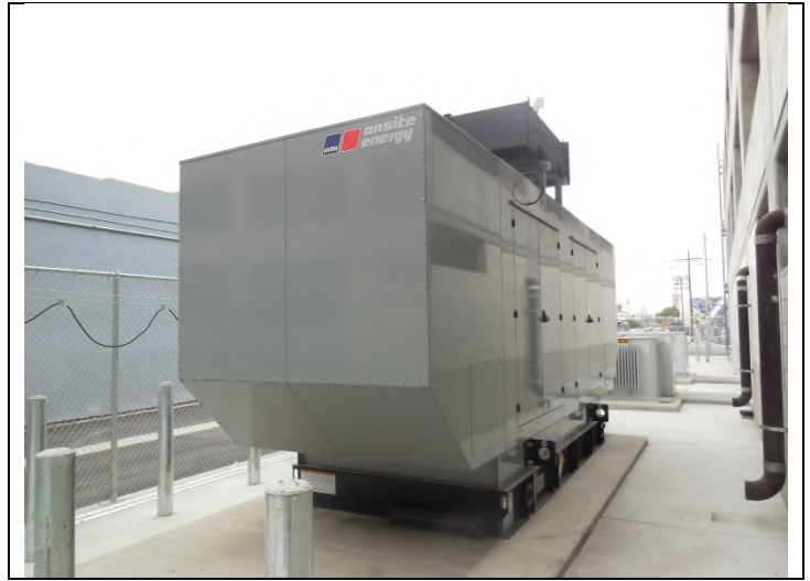
22. View of emergency generator
