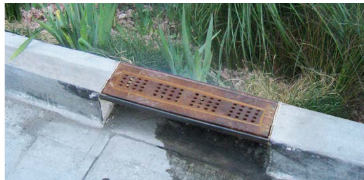
Curb drain (Condition #2) into vegetated stormwater curb extension with metal grate
