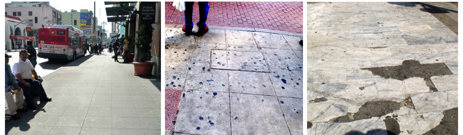
Some Sidewalk paving along Broadway has been laid in recent years, other shows its age. Other materials aside from concrete have been used, and are patched with asphalt.
