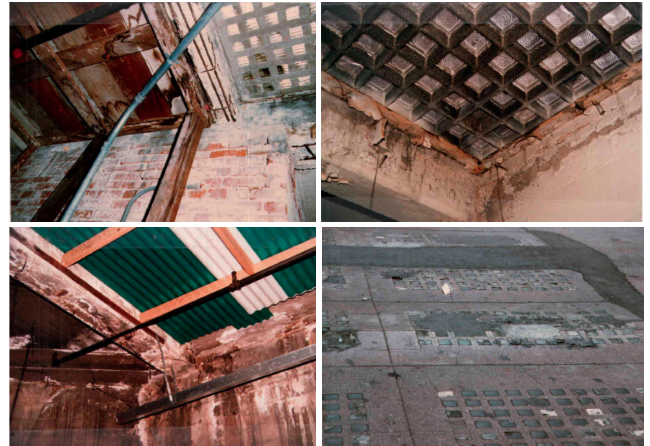
Most basements are in a serious state of deterioration, which can be seen both above and below ground.
