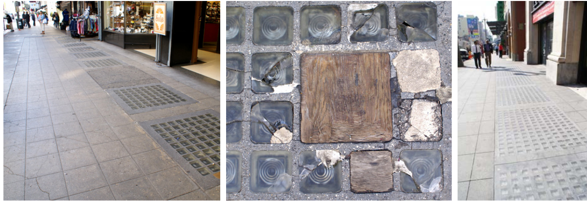
Glass Block Basement Skylights provide daytime illumination to basements below. Many are in need of critical repair and restoration.
