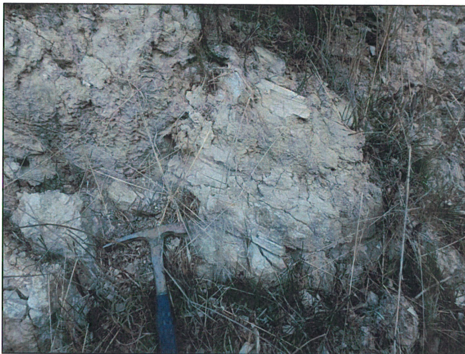
Figure 12. Monterey Formation sediments exposed on the slope of western portion of the Project area. View west.
