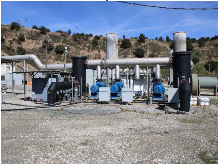
Photo 143: Flares 9, 10, 11 and Gas-to-Energy Facility: February 15, 2024
