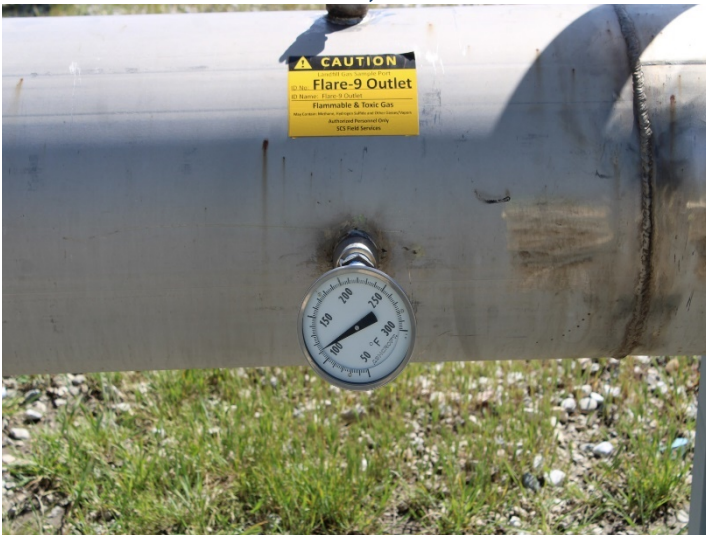
Photo 151: Flares 9, 10, 11 and Gas-to-Energy Facility: March 7, 2024
