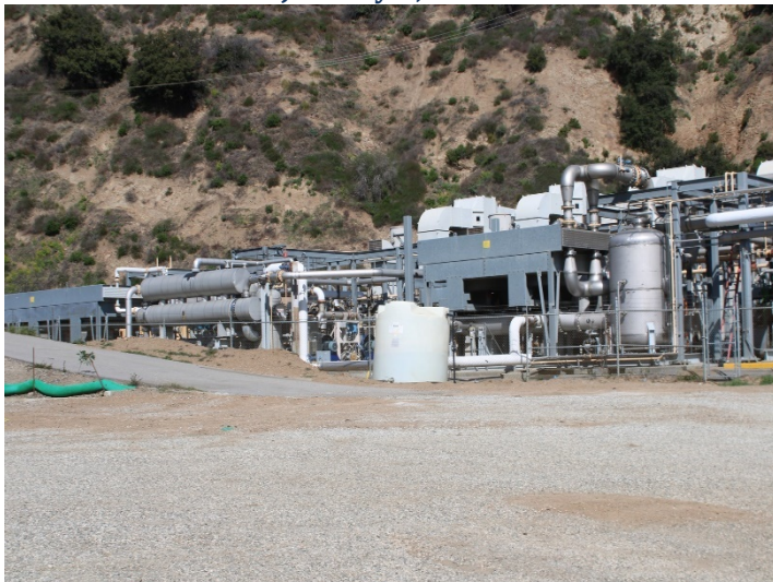
Photo 127: Flares 9, 10, 11 and Gas-to-Energy Facility: February 15, 2024
