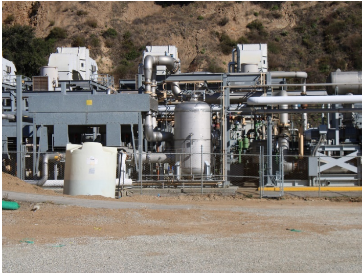
Photo 125: Flares 9, 10, 11 and Gas-to-Energy Facility: January 8, 2024
