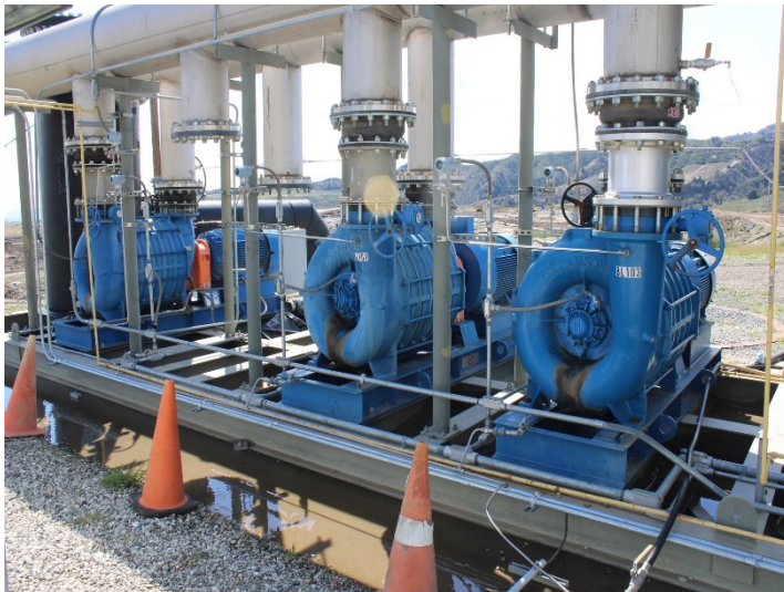
Photo 153: Flares 9, 10, 11 and Gas-to-Energy Facility: March 7, 2024
