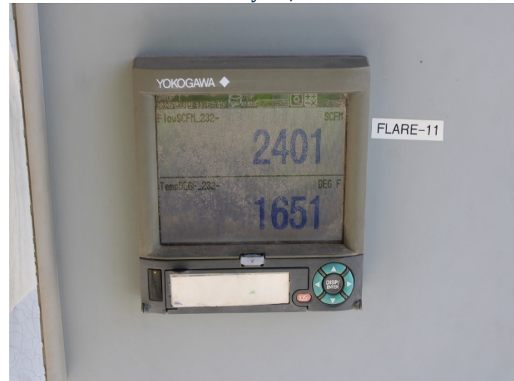
Photo 140: Flares 9, 10, 11 and Gas-to-Energy Facility: February 15, 2024
