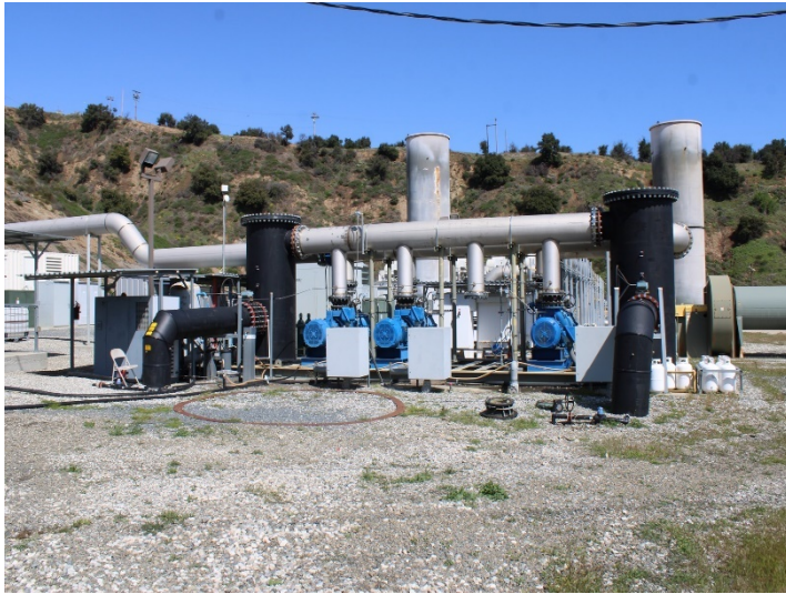
Photo 161: Flares 9, 10, 11 and Gas-to-Energy Facility: March 7, 2024
