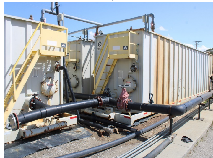
Photo 100: Alder Tank Liquids Treatment System: March 7, 2024
