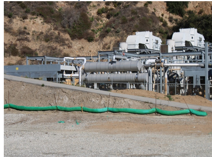
Photo 124: Flares 9, 10, 11 and Gas-to-Energy Facility: January 8, 2024
