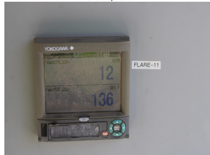
Photo 156: Flares 9, 10, 11 and Gas-to-Energy Facility: March 7, 2024
