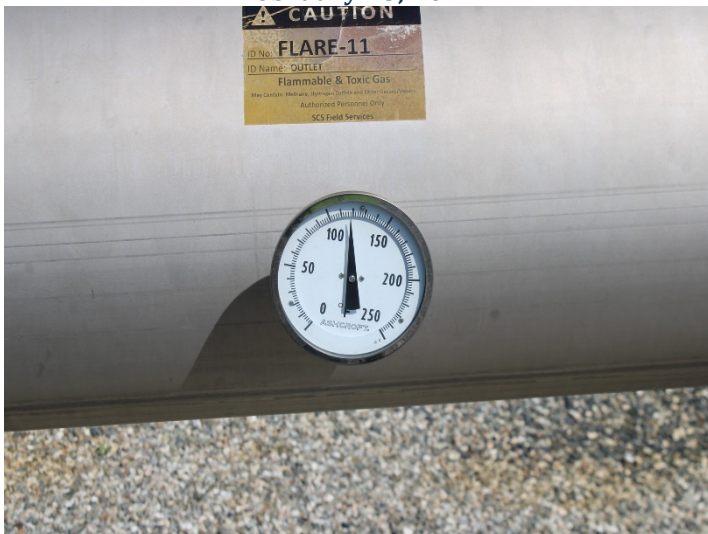
Photo 135: Flares 9, 10, 11 and Gas-to-Energy Facility: February 15, 2024
