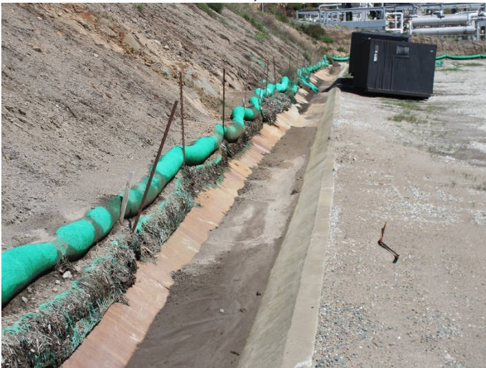
Photo 159: Flares 9, 10, 11 and Gas-to-Energy Facility: March 7, 2024
