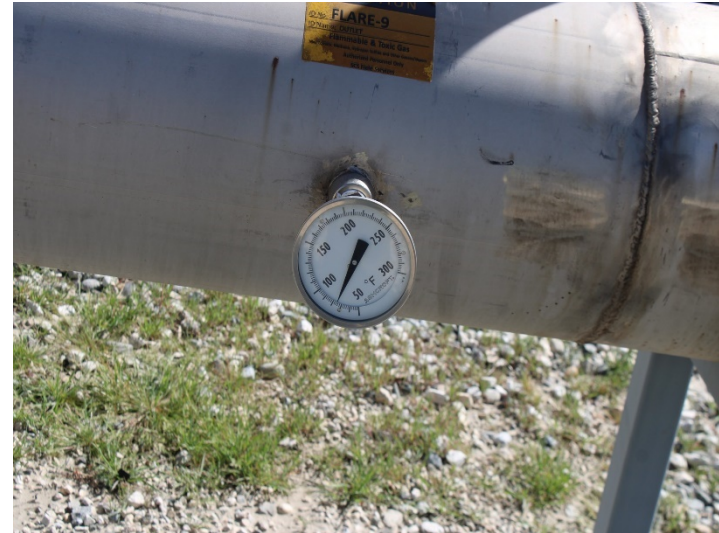
Photo 134: Flares 9, 10, 11 and Gas-to-Energy Facility: February 15, 2024
