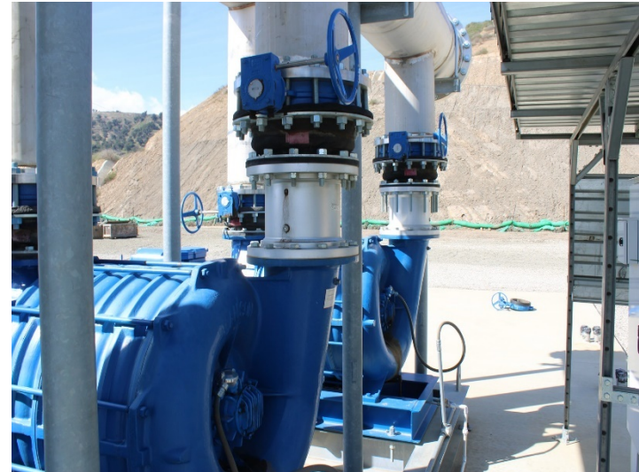
Photo 138: Flares 9, 10, 11 and Gas-to-Energy Facility: February 15, 2024
