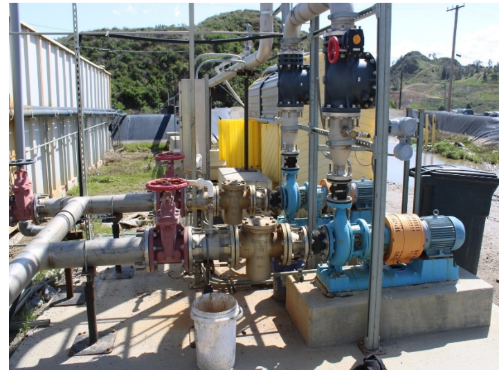
Photo 102: Alder Tank Liquids Treatment System: March 7, 2024
