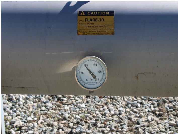
Photo 113: Flares 9, 10, 11 and Gas-to-Energy Facility: January 8, 2024
