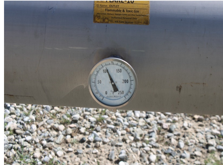
Photo 130: Flares 9, 10, 11 and Gas-to-Energy Facility: February 15, 2024
