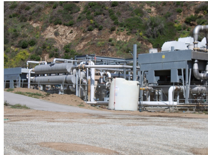
Photo 148: Flares 9, 10, 11 and Gas-to-Energy Facility: March 7, 2024
