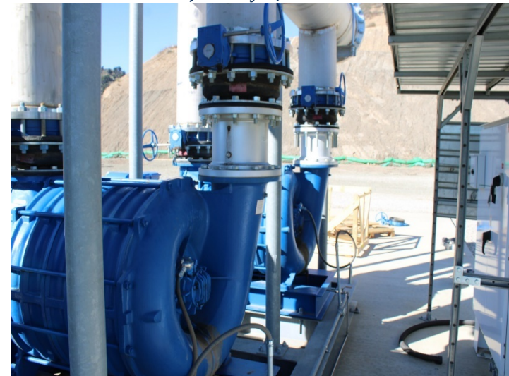
Photo 120: Flares 9, 10, 11 and Gas-to-Energy Facility: January 8, 2024
