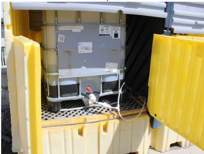
Photo 103: Alder Tank Liquids Treatment System: March 7, 2024
