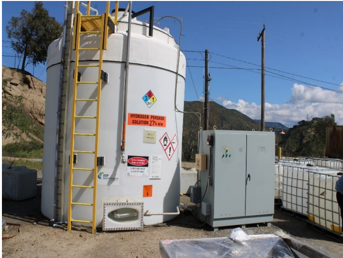
Photo 97: Alder Tank Liquids Treatment System: March 7, 2024
