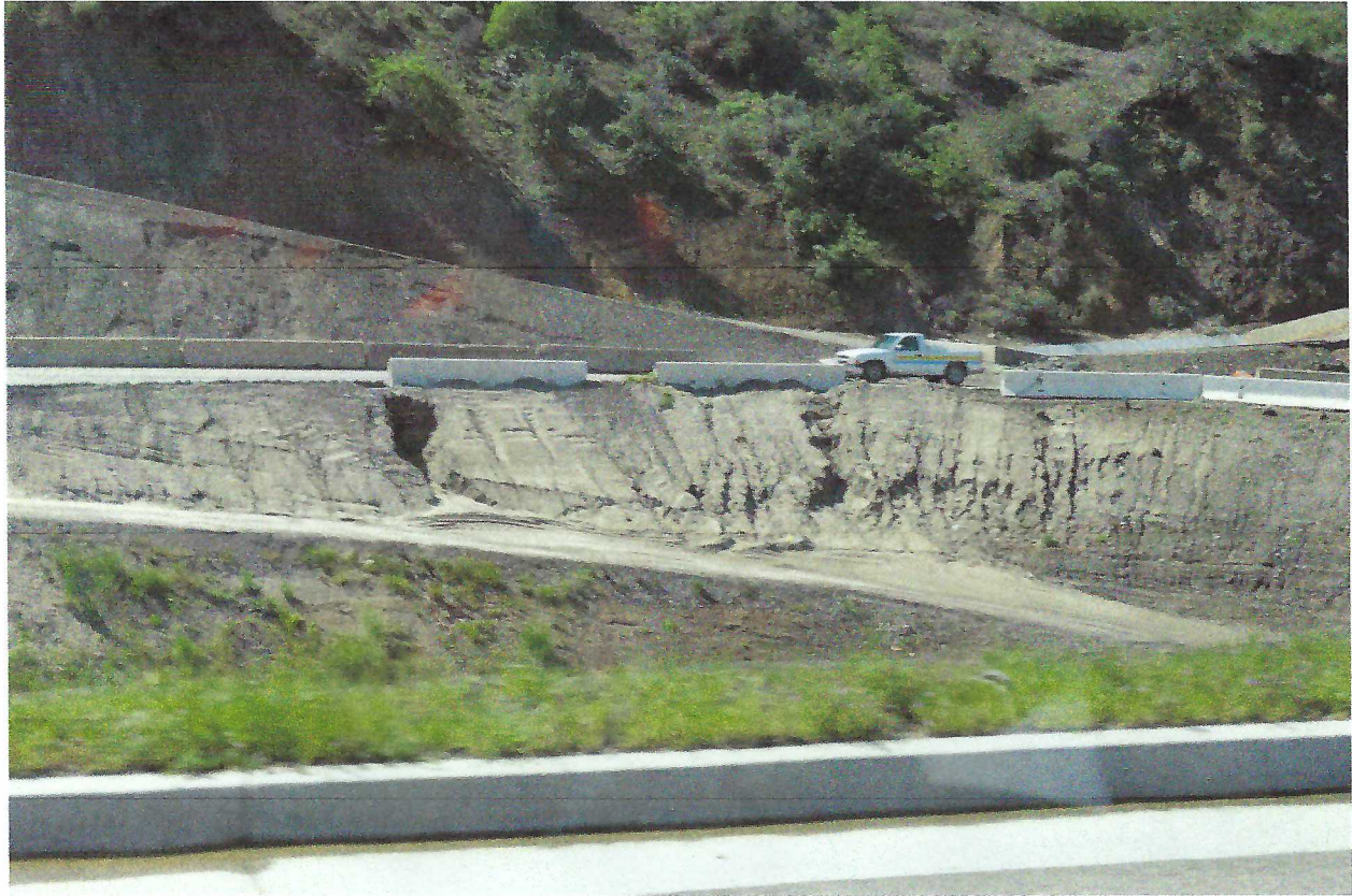
Figure 1: Erosion gullies and soil loss on access road embankment
