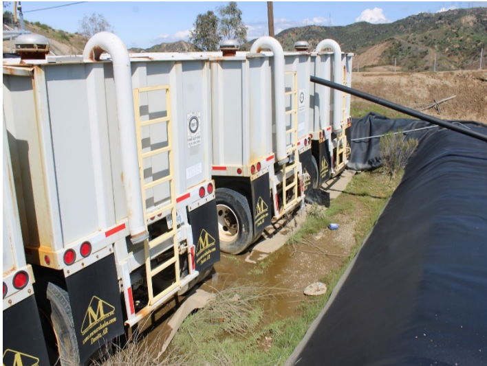
Photo 105: Alder Tank Liquids Treatment System: March 7, 2024
