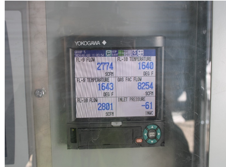
Photo 118: Flares 9, 10, 11 and Gas-to-Energy Facility: January 8, 2024
