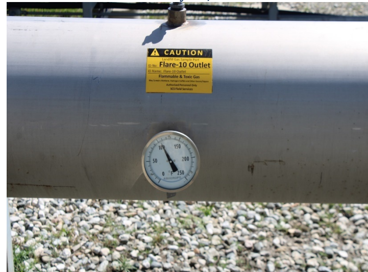
Photo 144: Flares 9, 10, 11 and Gas-to-Energy Facility: March 7, 2024
