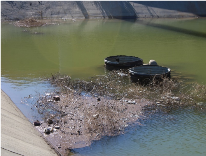
Photo 5: Basin A: January 8, 2024
