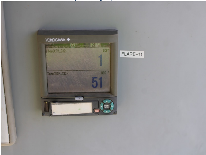
Photo 119: Flares 9, 10, 11 and Gas-to-Energy Facility: January 8, 2024
