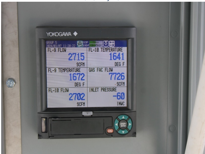
Photo 155: Flares 9, 10, 11 and Gas-to-Energy Facility: March 7, 2024
