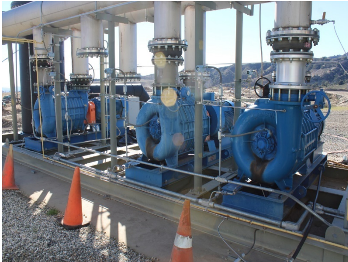
Photo 117: Flares 9, 10, 11 and Gas-to-Energy Facility: January 8, 2024
