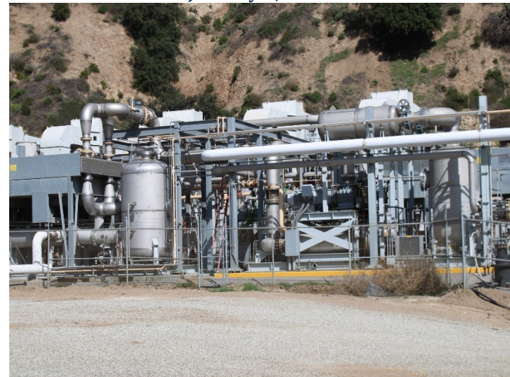
Photo 128: Flares 9, 10, 11 and Gas-to-Energy Facility: February 15, 2024
