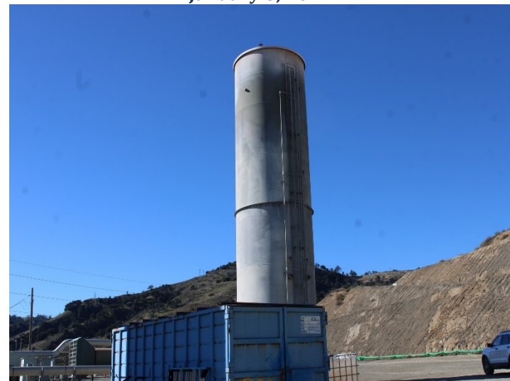
Photo 116: Flares 9, 10, 11 and Gas-to-Energy Facility: January 8, 2024
