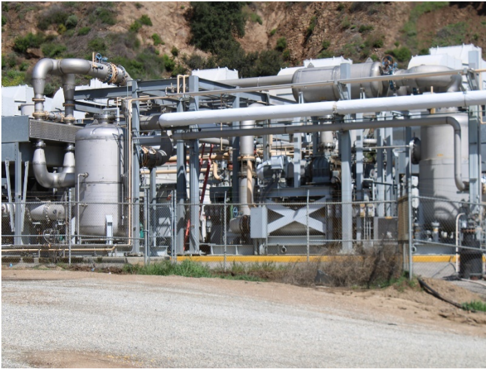
Photo 149: Flares 9, 10, 11 and Gas-to-Energy Facility: March 7, 2024
