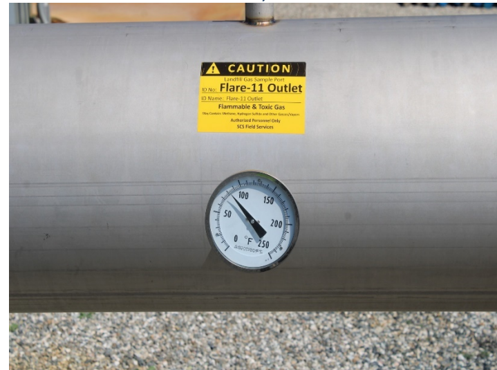
Photo 152: Flares 9, 10, 11 and Gas-to-Energy Facility: March 7, 2024
