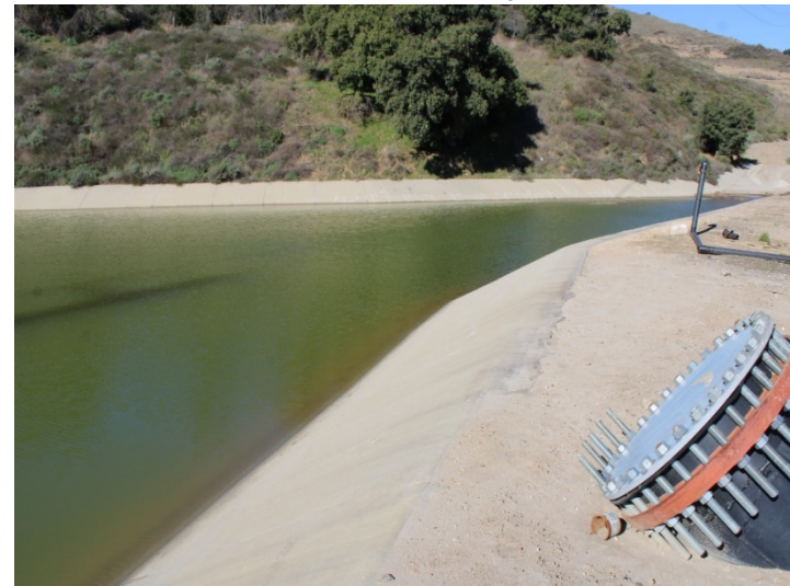
Photo 4: Basin A: January 8, 2024
