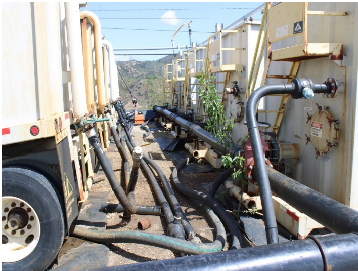
Photo 101: Alder Tank Liquids Treatment System: March 7, 2024
