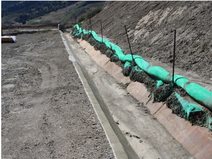
Photo 141: Flares 9, 10, 11 and Gas-to-Energy Facility: February 15, 2024
