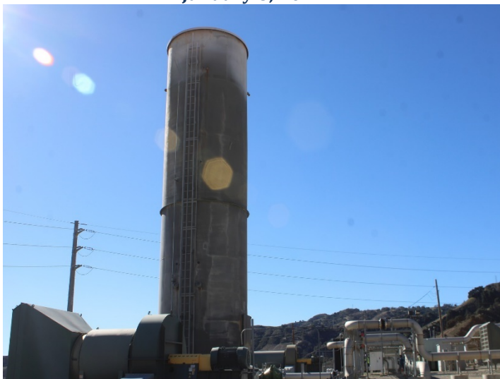
Photo 115: Flares 9, 10, 11 and Gas-to-Energy Facility: January 8, 2024
