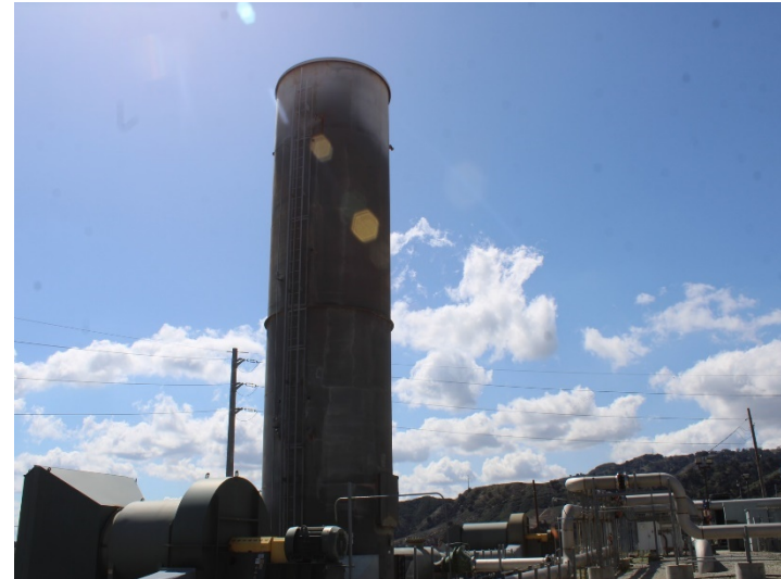
Photo 146: Flares 9, 10, 11 and Gas-to-Energy Facility: March 7, 2024
