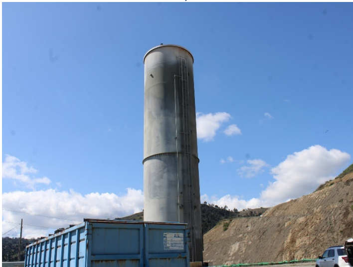
Photo 147: Flares 9, 10, 11 and Gas-to-Energy Facility: March 7, 2024
