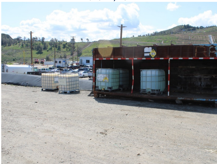
Photo 99: Alder Tank Liquids Treatment System: March 7, 2024
