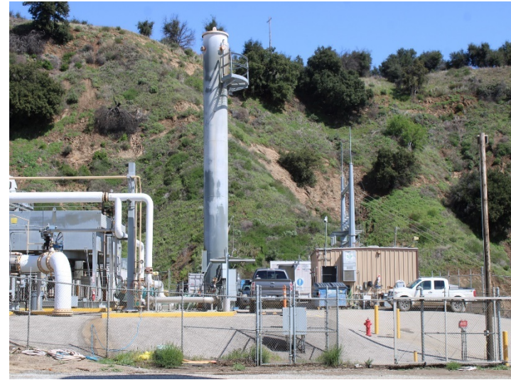
Photo 150: Flares 9, 10, 11 and Gas-to-Energy Facility: March 7, 2024
