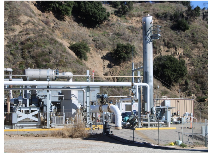
Photo 126: Flares 9, 10, 11 and Gas-to-Energy Facility: January 8, 2024
