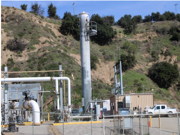
Photo 129: Flares 9, 10, 11 and Gas-to-Energy Facility: February 15, 2024
